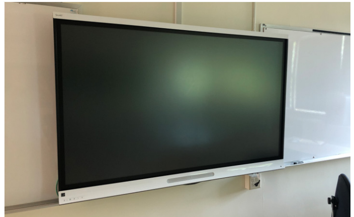
Photo of classroom AV system on second floor.
