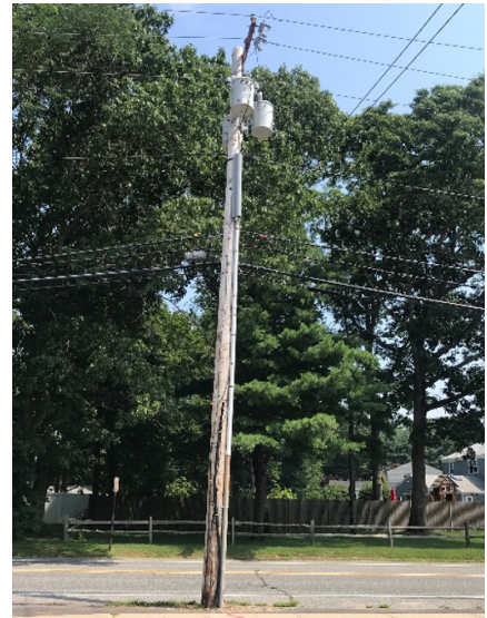
Service #1 Riser Pole #2
