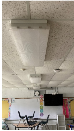
Typical Classroom Lighting with Surface Wraparounds
