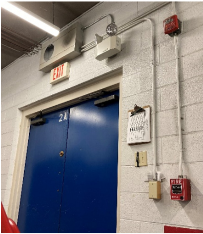
Emergency Battery Unit
