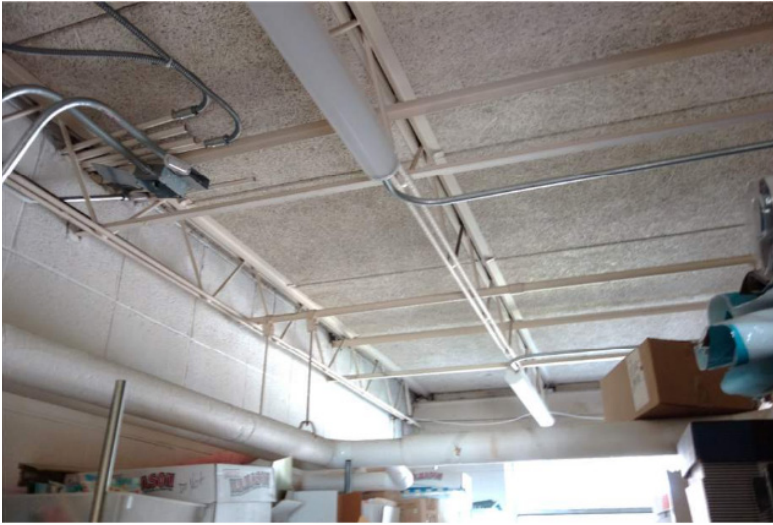
Photo of open web steel joist and tectum roof panels and bearing upon a steel beam.
