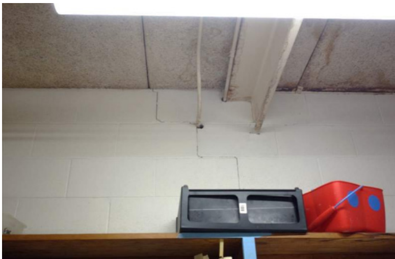
Additional photo showing a step crack in a cmu wall.
