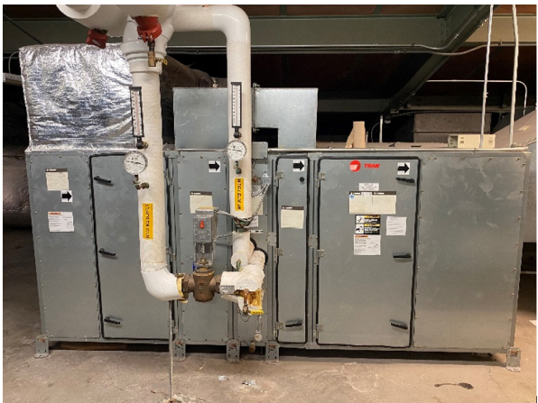
Air Handling Unit
