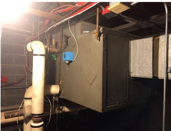
Typical Air Handling Unit
