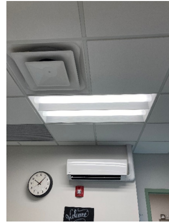
Office Recessed Lighting
