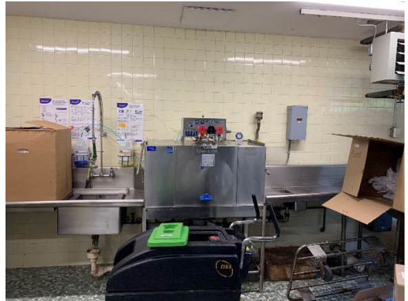
No Hood or Exhaust System at the Dishwasher
