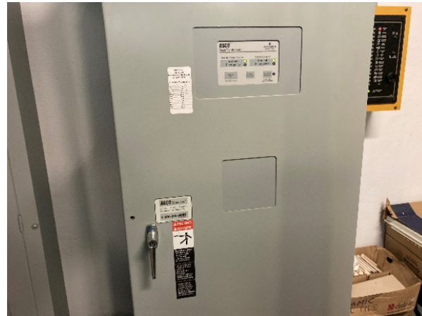
Automatic Transfer Switch
