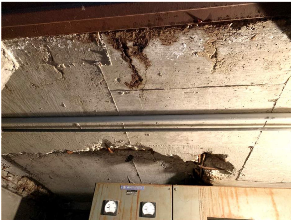
Additional photo showing spalled concrete, exposed and rusting reinforcement bars and efflorescence in the electrical room adjacent to the boiler room.
