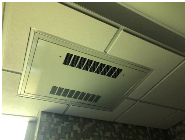
Typical Corridor Unit Heater
