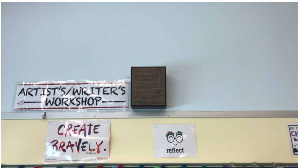
Photo of typical classroom speaker assembly
