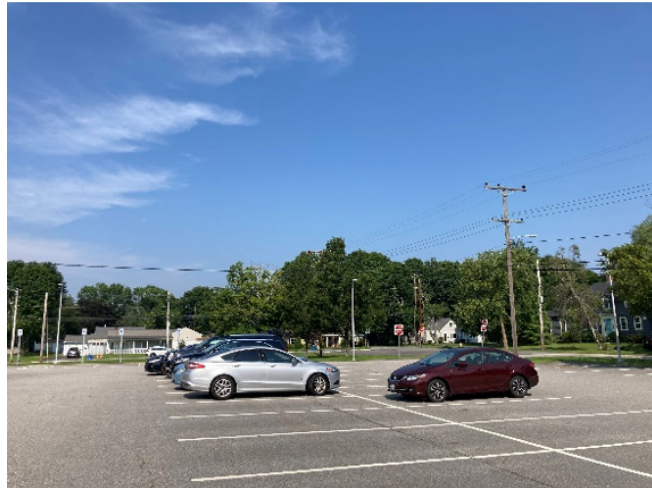
Wiring Runs Overhead From Utility Pole on Old County Road
