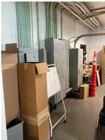
Older Westinghouse Panels in Boiler Room
