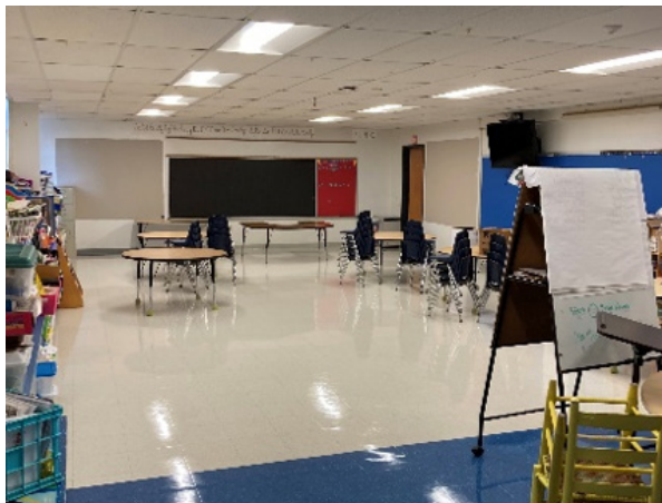
Typical Classroom Lighting with Recessed Troffers
