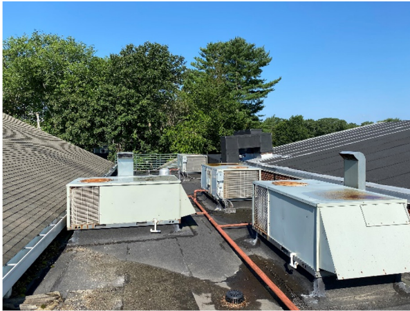
Typical Packaged Rooftop Units
