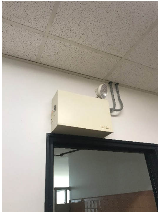
Central Battery Unit
