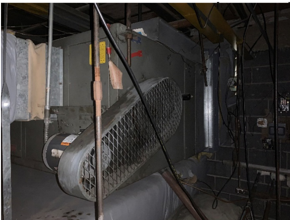
Air Handling Unit
