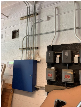
Control Panel within Mechanical Room
