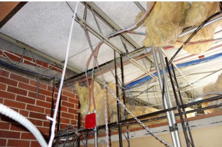
Photo of roof framing at Hampden Elementary School. The original portion of Primrose Elementary is assumed to be constructed in a similar fashion with open web steel joists and tectum roof panels.
