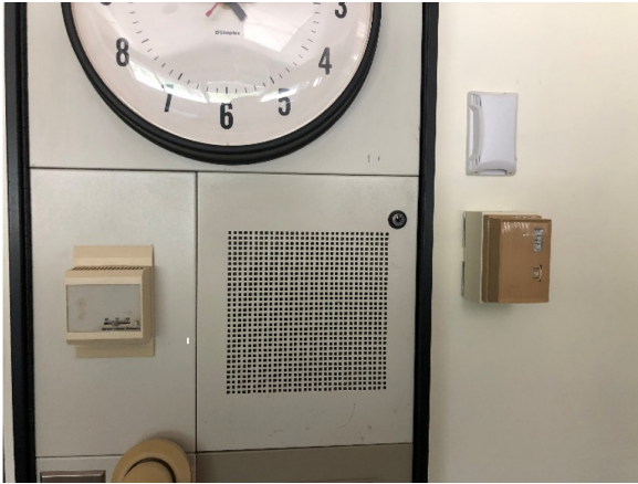
Various Thermostats Serving Same Space
