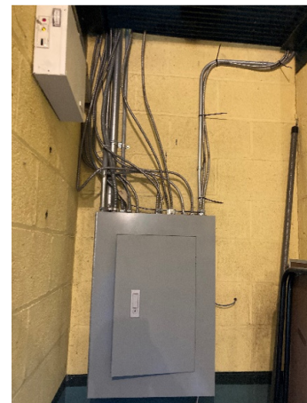
Remote Panel in Storage Closet
