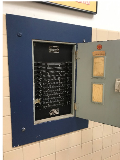
Older Westinghouse Panel in Corridor
