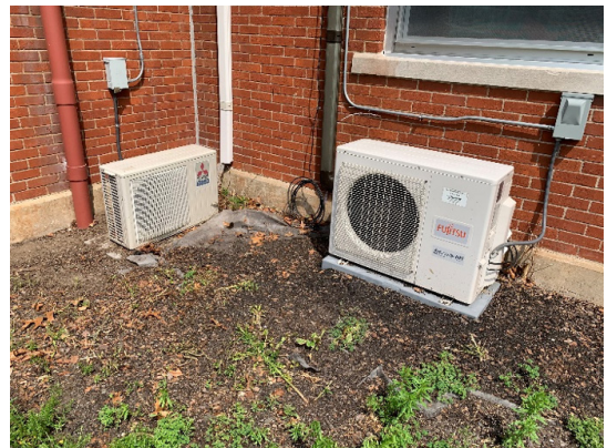
Outdoor Condensing Units Near Administration
