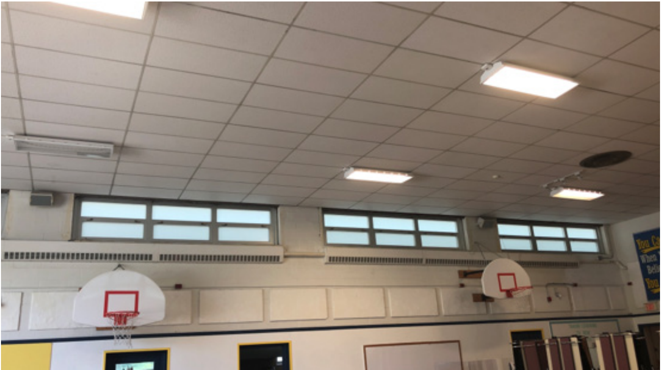
Speakers mounted on exterior walls
