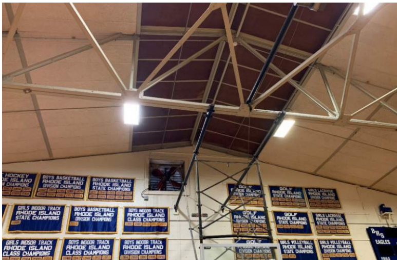
Photo of a metal truss in the gym supporting tectum roof panels.
