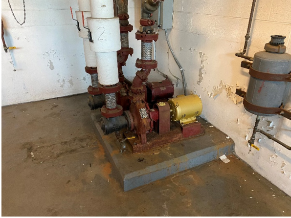
Existing Pumps (Boiler Room #2)
