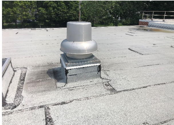
Typical Roof Exhaust Fan
