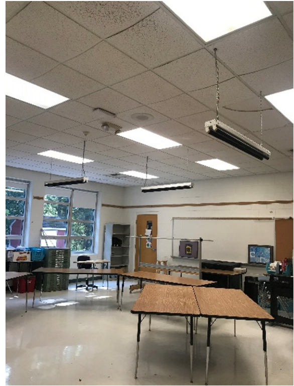
Typical Classroom Lighting in the Addition
