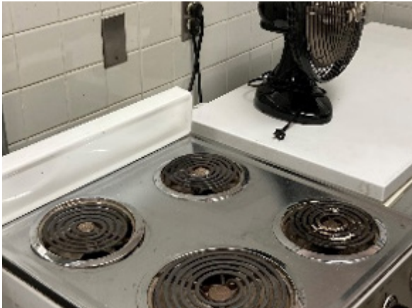
Kitchen Non-GFI Receptacles
