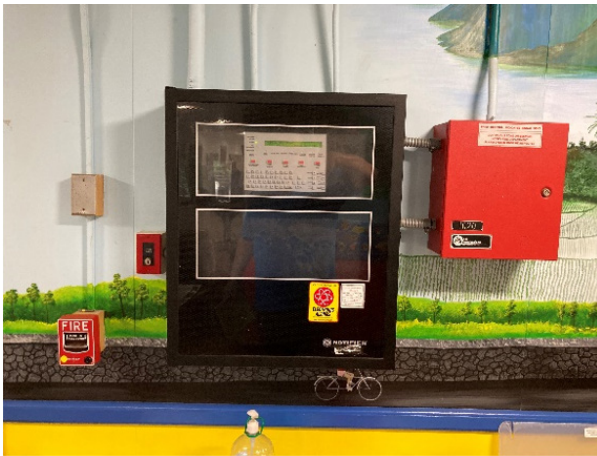
Fire Alarm Control Panel & Radio Box
