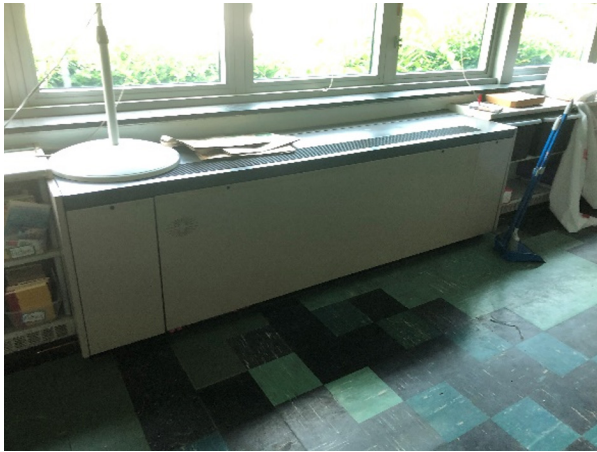
Typical Older Unit Ventilator
