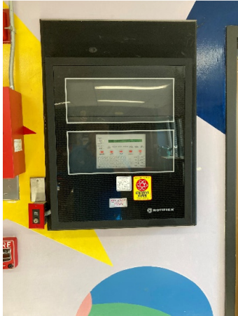
Fire Alarm Control Panel
