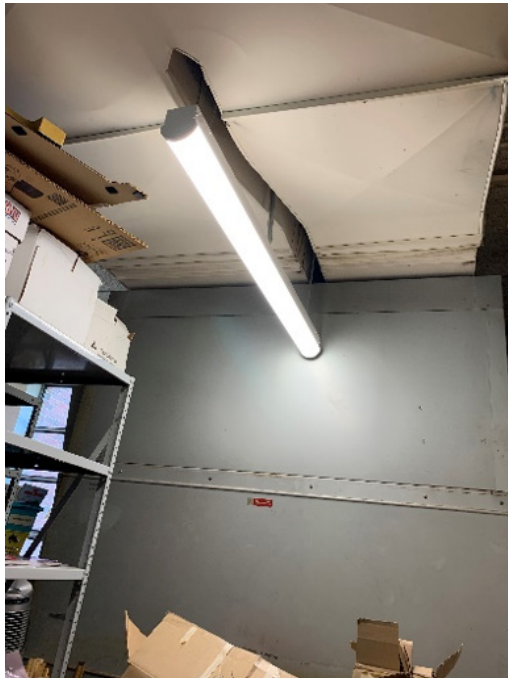
Cafetorium Air Handler
