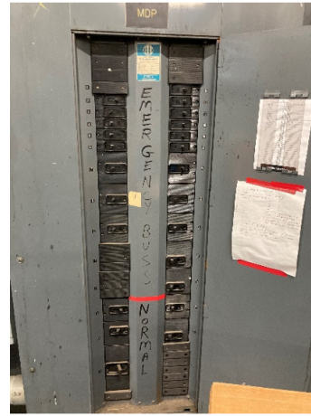
Main Dist. Panel in Boiler Room
