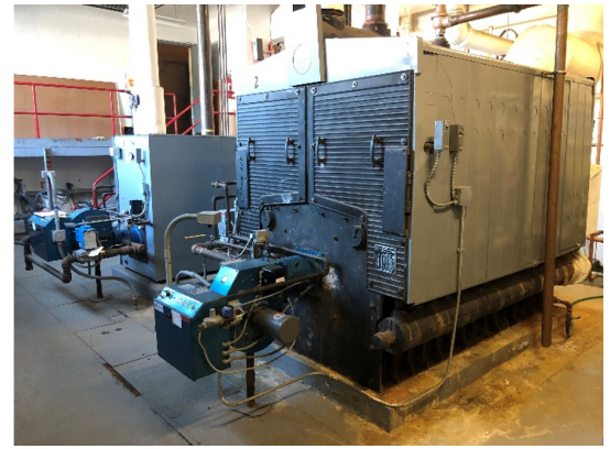
Existing Boilers (Boiler Room #1)
