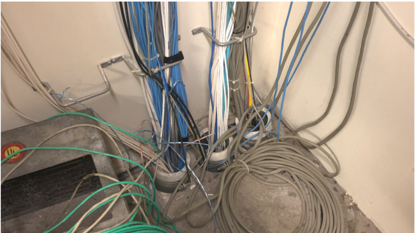
Photo of non-firestopped penetrations for cable pathways
