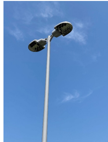
Parking Lot Pole Mounted LED Fixtures
