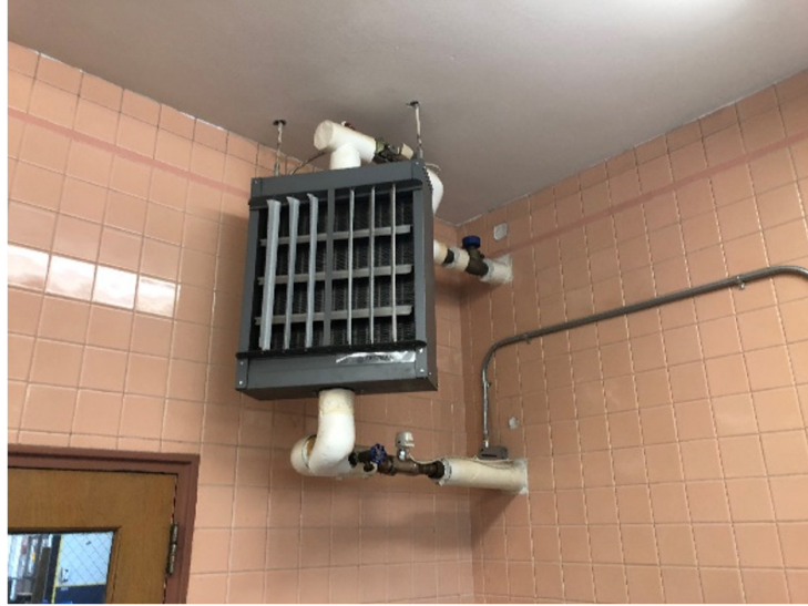
Kitchen Unit Heater
