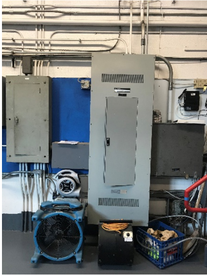
C/T Cabinet and Main Distribution. Panel in Boiler Room
