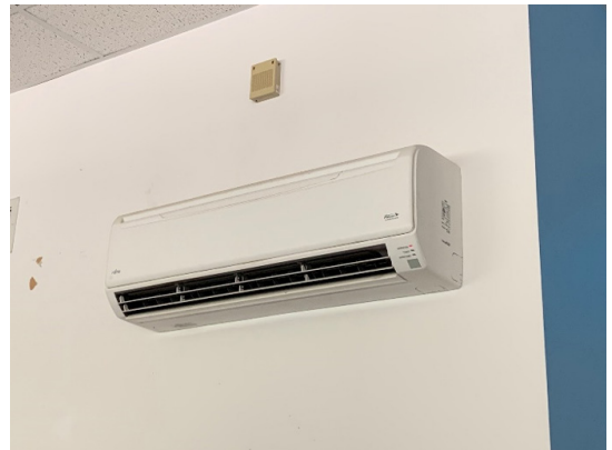
Indoor Wall Evaporative Unit Serving Library
