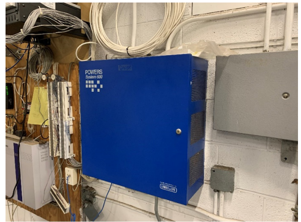
Powers System 600 Control Panel
