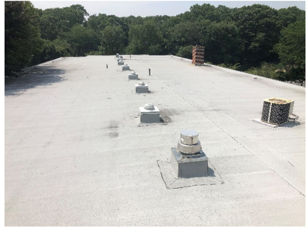
Typical Exhaust Fans
