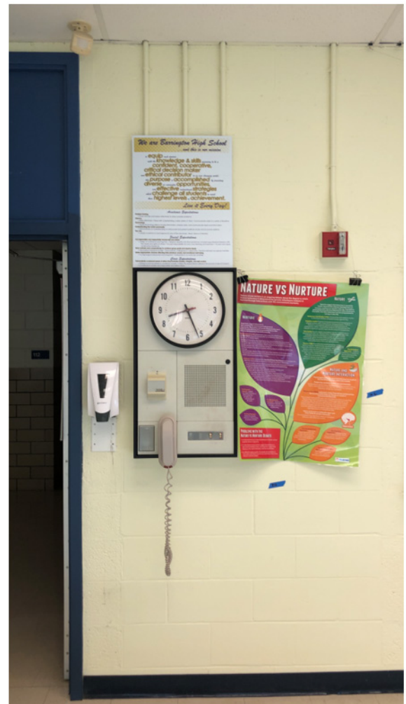
Photo of typical classroom Phone / Clock / PA Speaker assembly
