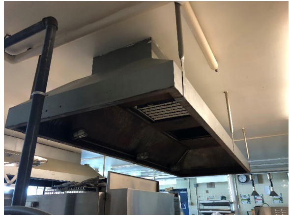
Kitchen Exhaust Fans and Make-up Air Unit
