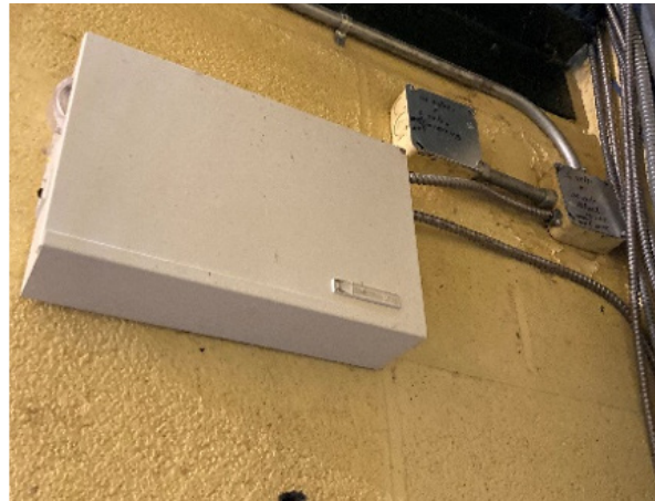
Central Battery Unit
