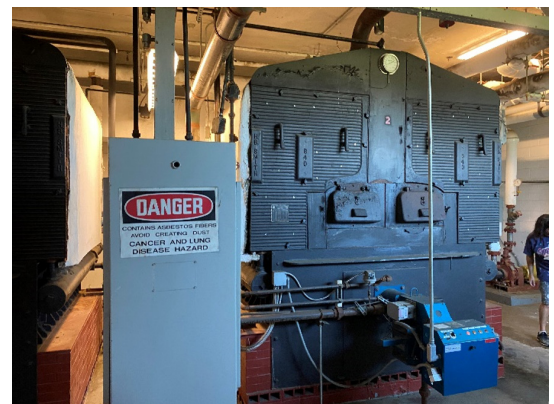
Existing Boiler 2 (Boiler Room #2)
