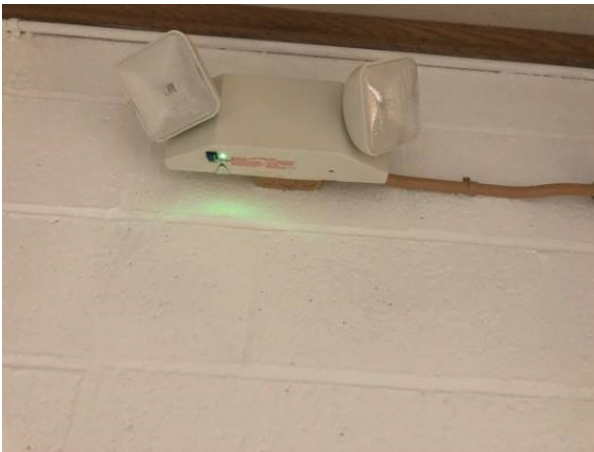
Emergency Battery Unit
