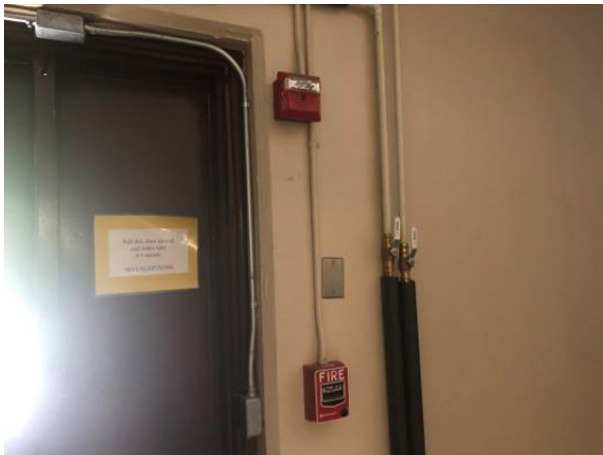
Horn/Strobe & Pull Station
