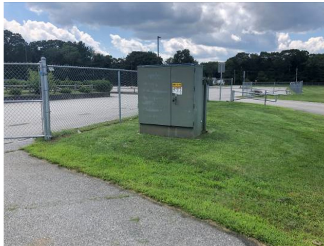
Pad Mounted Transformer
