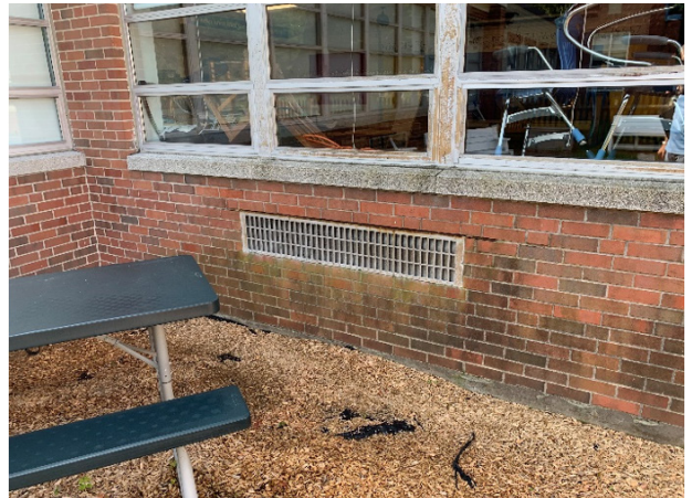
Outdoor Air Intake Louver Associated with Unit Vent
