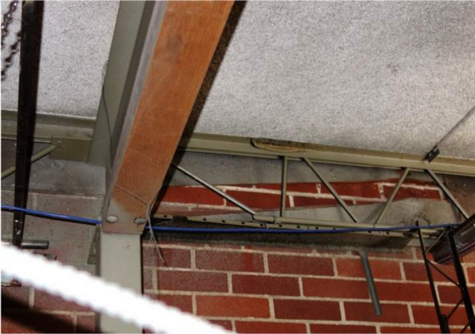
Photo of open web steel joist and tectum roof panels and bearing upon a steel beam
