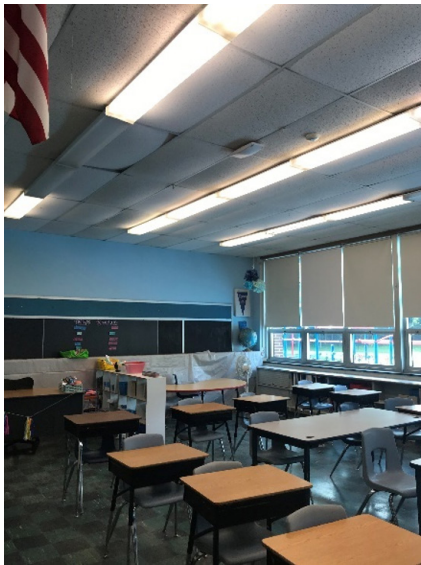
Typical Classroom Lighting with Surface Wraparounds
