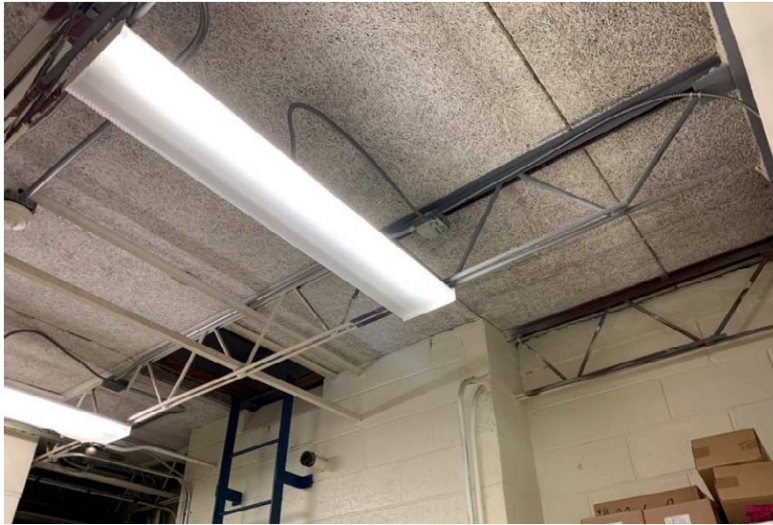
Photo of open web steel joists supporting tectum roof panels in one of the utility rooms.
