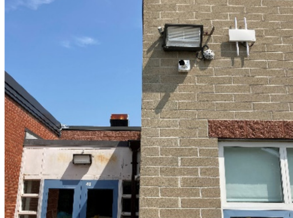
Exterior Wall Pack Fixtures
