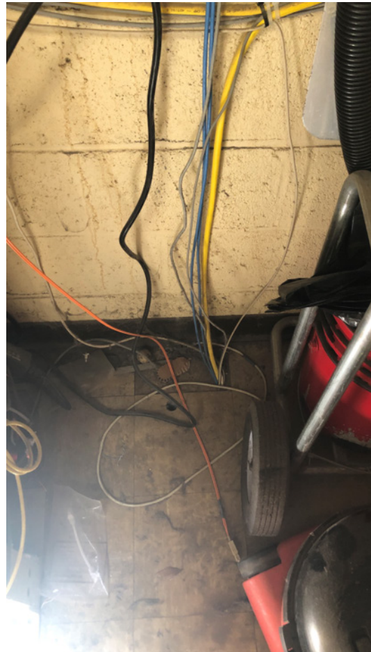
Photo of non-firestopped sleeve in IDF2 below.
