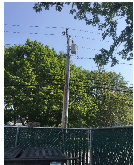
Service #2 Riser Pole #3-50
