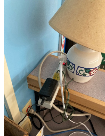
Limited Receptacles with Power Strip Use
