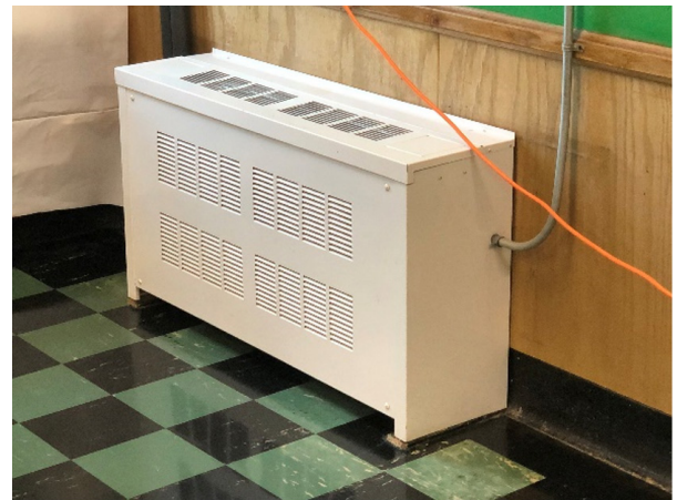
Typical Fan Coil
