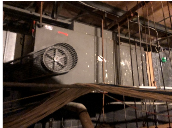
Typical Air Handling Unit
