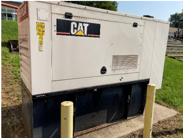
Exterior Backup Generator
