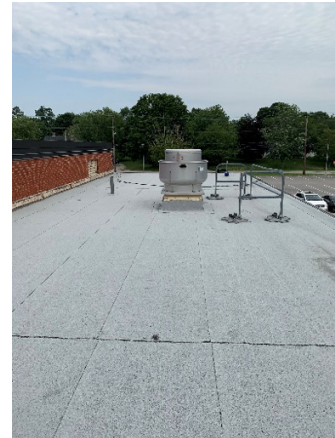
Kitchen Exhaust System Fan
