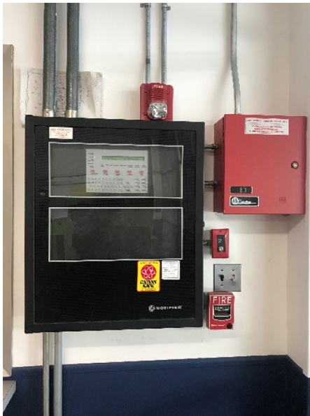
Fire Alarm Control Panel and Radio Box
