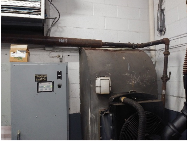
Automatic Transfer Switch
