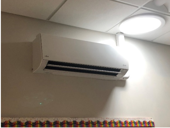
Air Conditioning Unit
