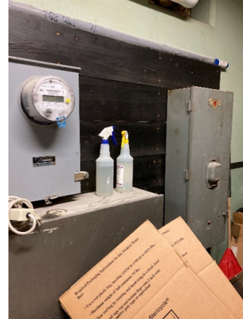
Circuit Breaker and Meter in Main Electric Room
