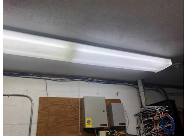
Work Room Lighting
