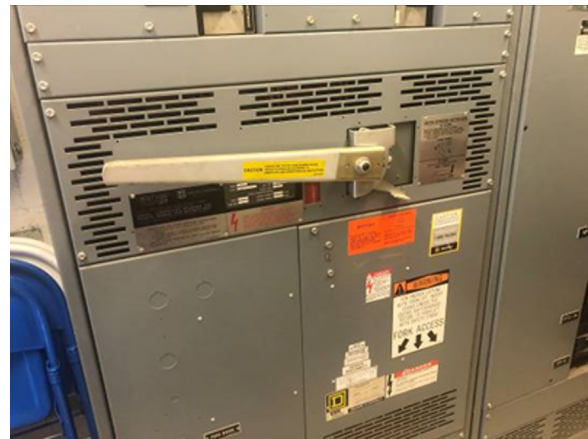
2000A Main Switch and CT Section
