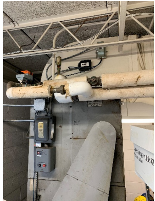
Cafetorium Air Handler
