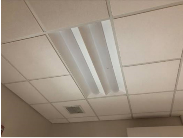
Main Office Lighting
