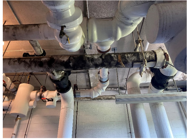
Water damaged insulation (Boiler Room #2)
