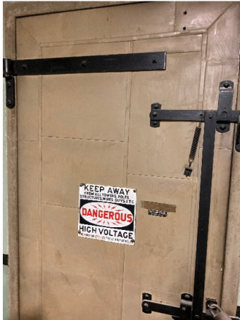
Transformer Vault for Main Electric Service
