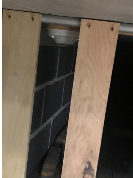
Heat Detector Below Stage
