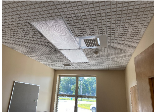
Typical Ceiling Mounted Diffuser and Register
