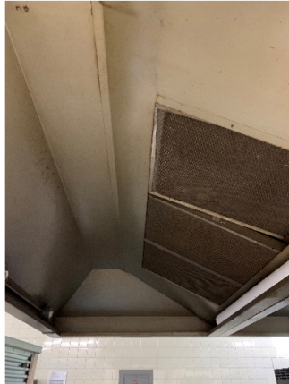
Picture of Inside of Kitchen Hood
