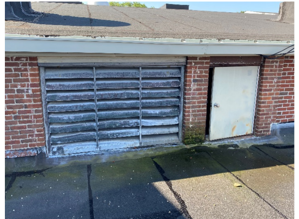
Louver Associated with Air Handler
