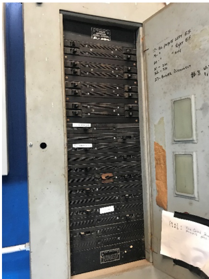
Older Westinghouse Panel in Boiler Room
