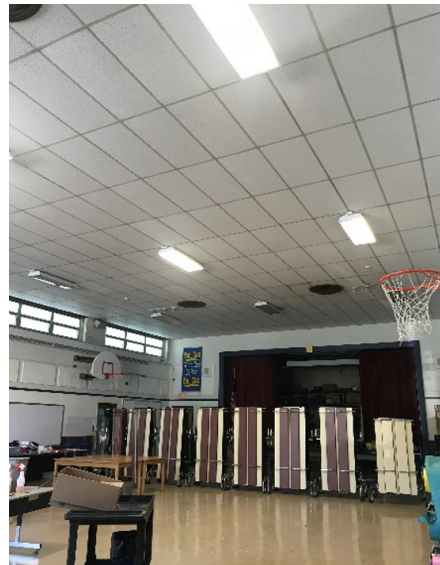
Multi-Purpose Room Lighting
