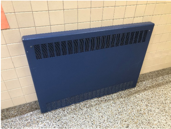
Corridor Unit Heater
