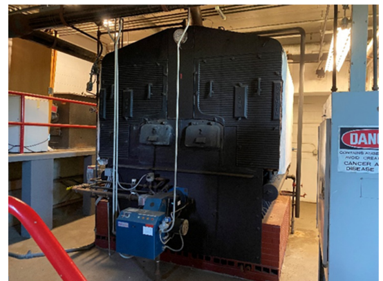
Existing Boilers 1 (Boiler Room #2)
