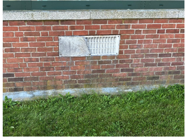
Outdoor Air Intake Louver Associated with Unit Vent
