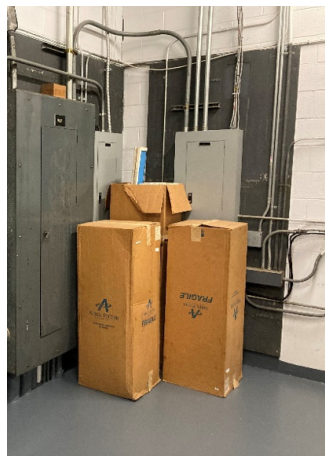
Branch Circuit Panels
