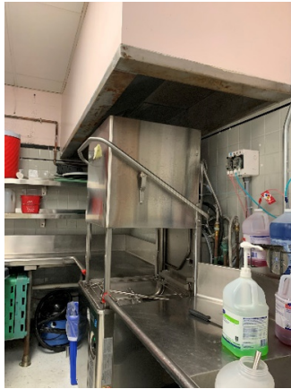
Kitchen Hood at Dishwasher
