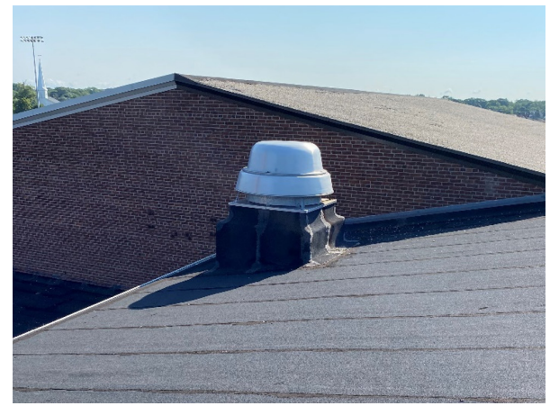
Typical Roof Mounted Exhaust Fan
