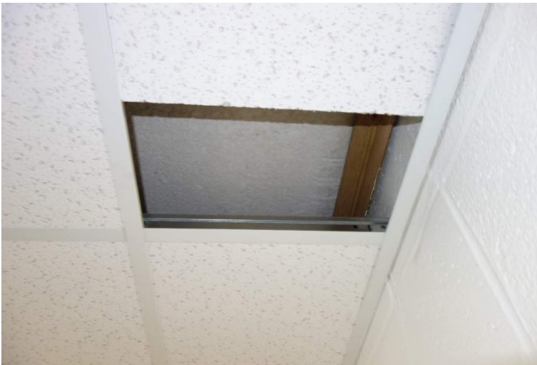
Photo of the hard ceiling above the dropped ceiling panels at Primrose Elementary.
