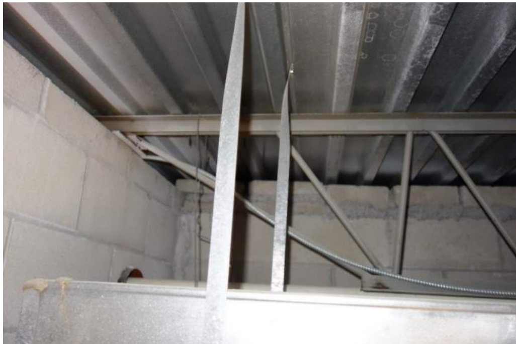
Photo of open web steel joist and metal roof deck bearing upon a cmu wall.
