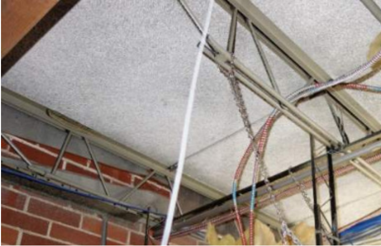
Photo of roof framing at Hampden Elementary School. The original portion of Nayatt Elementary is assumed to be constructed in a similar fashion with open web steel joists and tectum roof panels.
