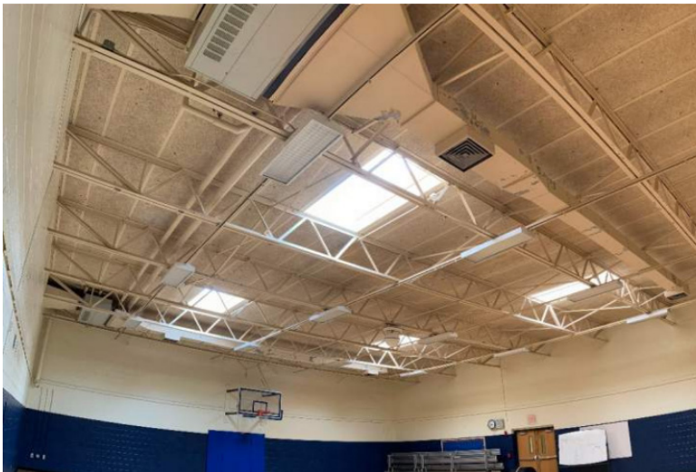
Photo of long span steel joists in the auxiliary gym supporting tectum roof panels.
