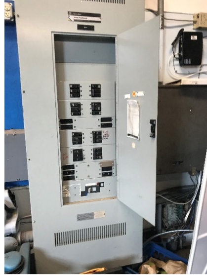
Main Dist. Panel in Boiler Room
