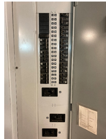
Newer Added Siemens Panel in Boiler Room
