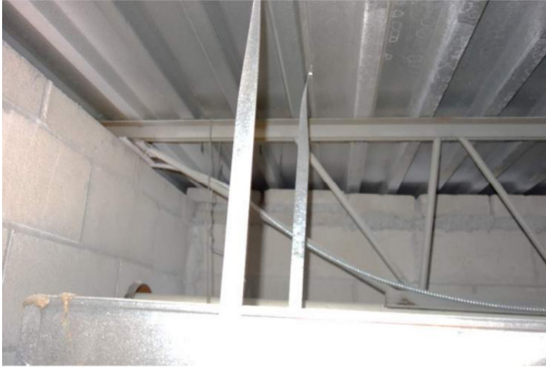
Photo of roof framing at Hampden Elementary School. The eastern addition at Primrose Elementary School is assumed to be constructed in a similar fashion with open web steel joists and steel roof decking.
