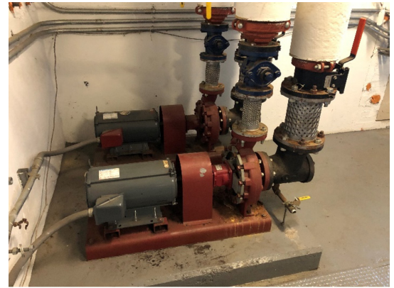
Pumps (Boiler Room #1)
