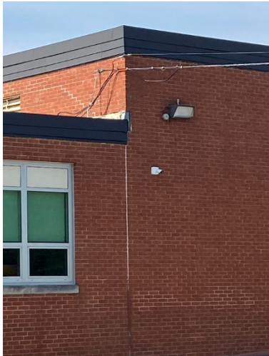
Overhead Wires Enter Building for Electric Service
