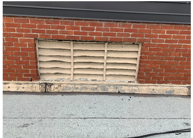
Louver Associated with Air Handler
