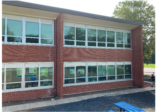
No Outdoor Air Intake Louver Associated with Unit Vent
