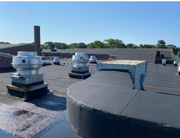
Kitchen Exhaust Fans and Make-up Air Unit
