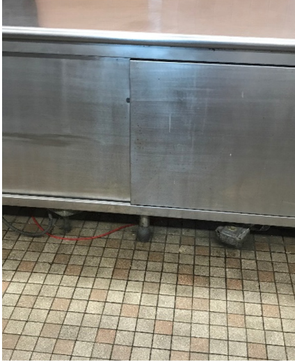
Kitchen Face-Up Non-GFI Receptacles
