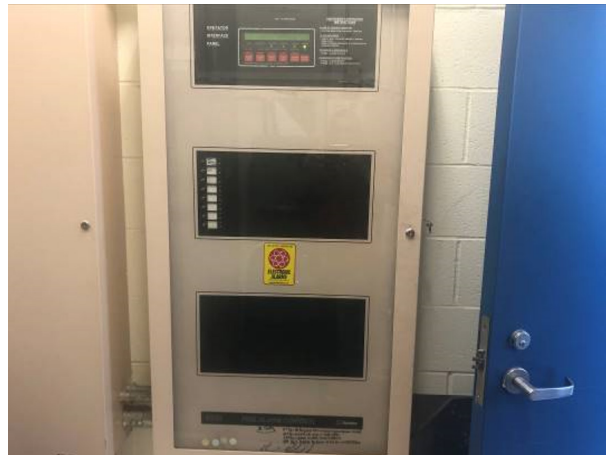
Fire Alarm Control Panel
