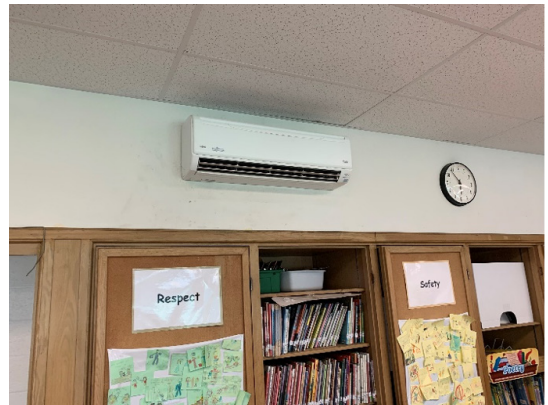
Indoor Wall Evaporative Unit
