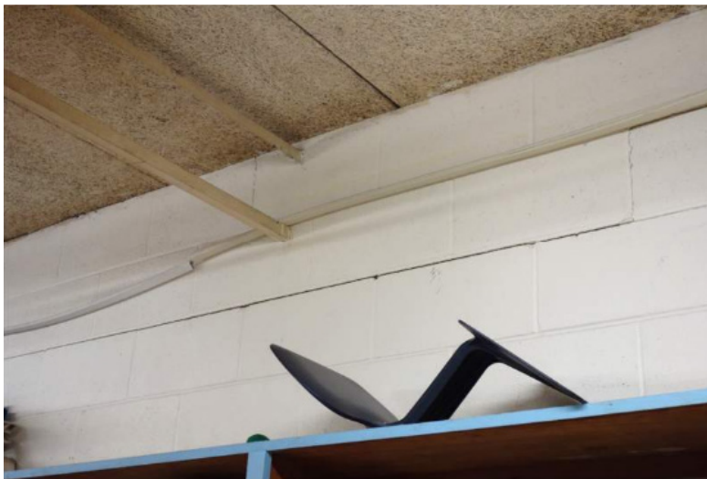
Photo of open web steel joist and tectum roof panels and bearing upon a steel beam.
