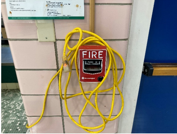
Extensive Extension Cord Use
