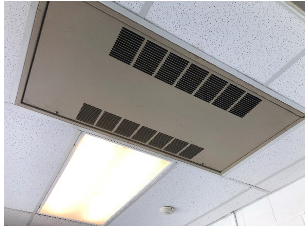
Vestibule Unit Heater
