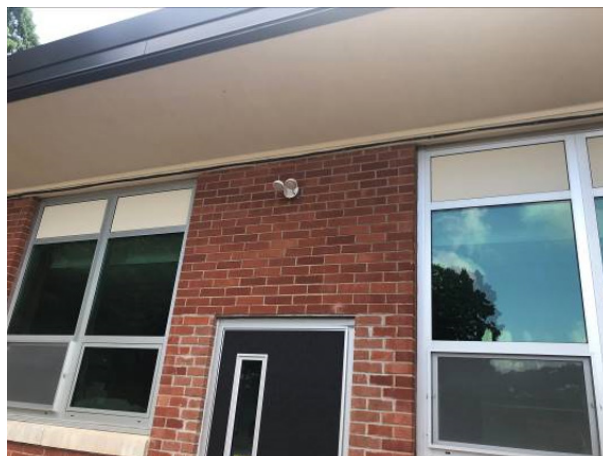
Remote Exterior Emergency Heads
