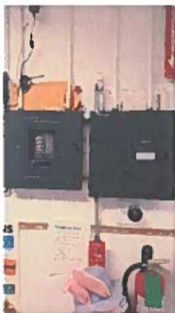
Main Fire Alarm Control Panel
