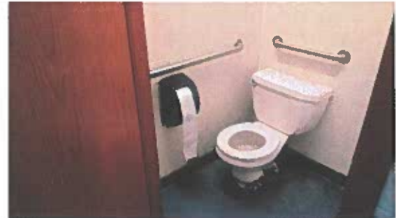
ADA toilet stalls do not meet space requirements
