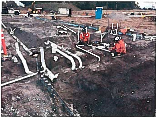
Plumbing runs under locker rooms
