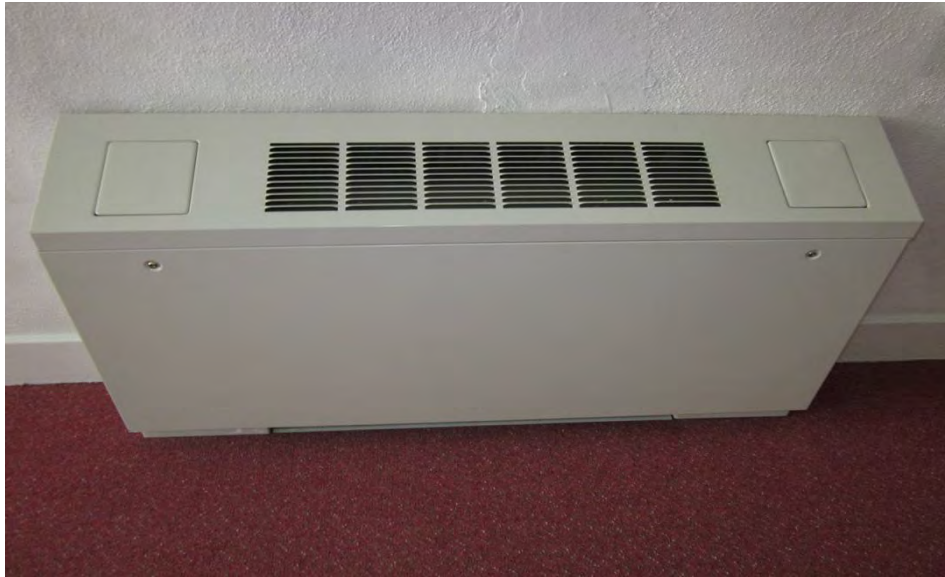
Photo 5 Location: Inside Elementary School Date: 08/06/2013 Looking at the heating unit
