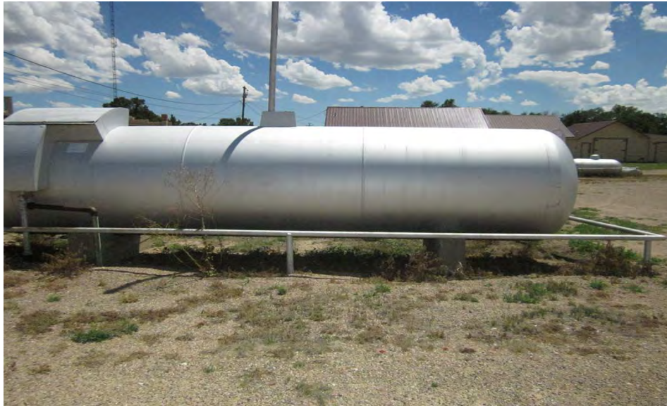
Photo 21 Location: West Side of School Date: 08/06/2013 Looking at propane AST
