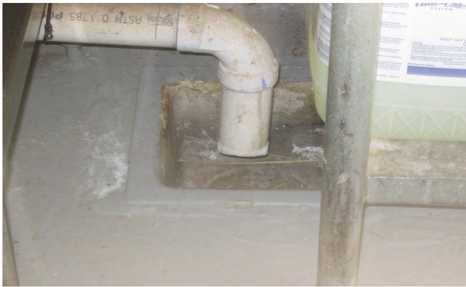
Photo 34 Location: Inside Elementary School Date: 08/06/2013 Looking at drain on floor in kitchen
