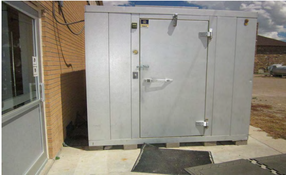
Photo 31 Location: South Side of Site Date: 08/06/2013 Looking at elevated freezer unit
