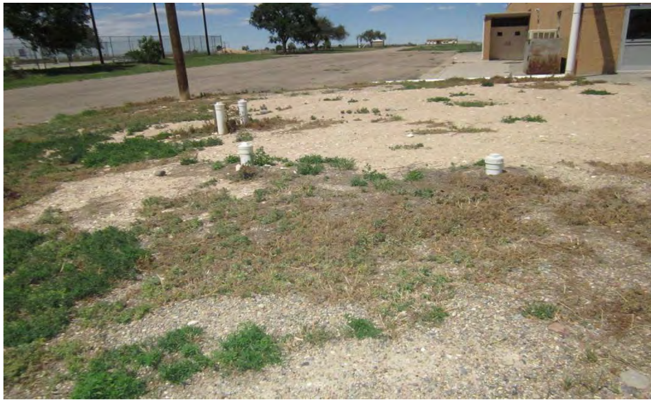
Photo 30 Location: West Side of Site Date: 08/06/2013 Facing north, looking at pipes protruding from septic system
