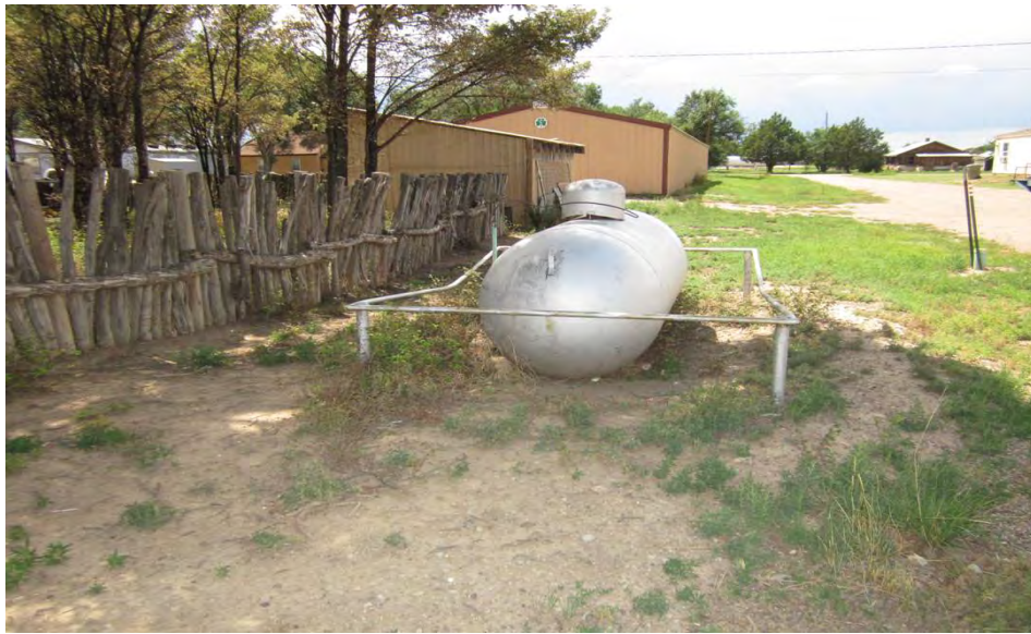
Photo 46 Location: Near Vocational Building Date: 08/06/2013 Looking at propane AST
