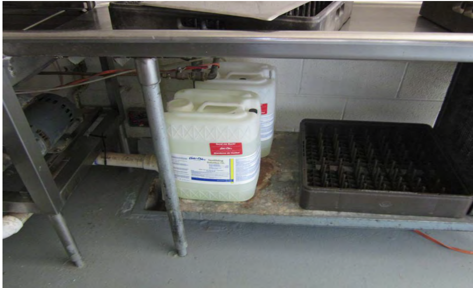
Photo 33 Location: Inside Elementary School Date: 08/06/2013 Looking at area where dishwashing detergent is stored
