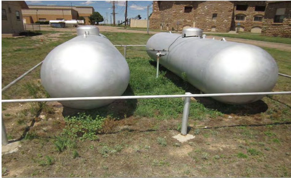
Photo 23 Location: West Side of School Date: 08/06/2013 Looking at two propane ASTs
