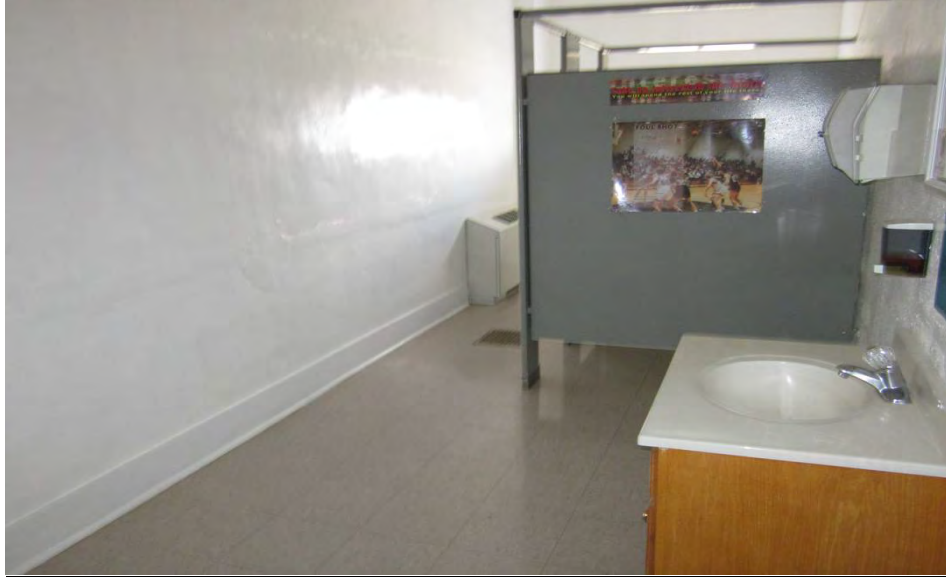
Photo 3 Location: Inside Elementary School Date: 08/06/2013 Looking inside of one of the bathrooms
