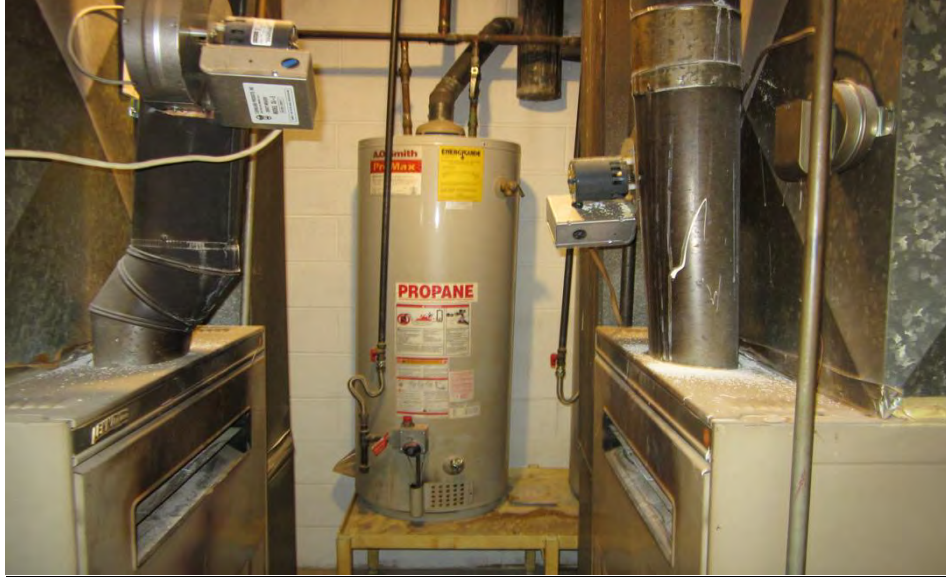
Photo 37 Location: Inside Elementary School Date: 08/06/2013 Looking at mechanical room with water heater
