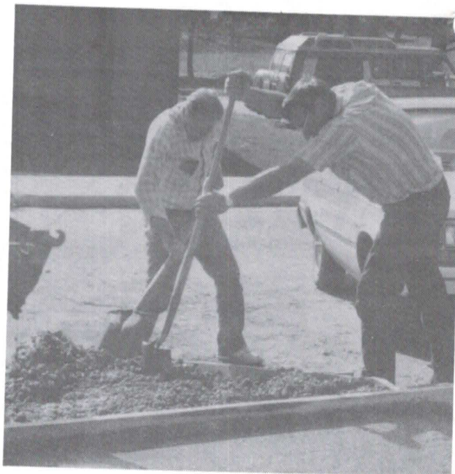
Earnie Massey and Glen Obarts place a ramp to make the business building accessible to handicapped.
