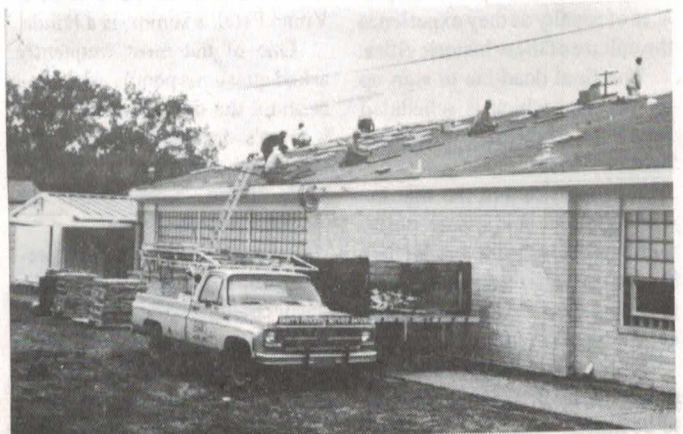
A new roof has recently been put on the math/science building at PHS.
