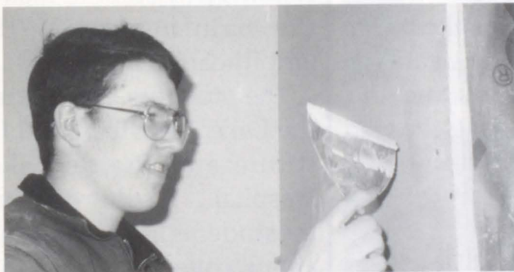
ABOVE: Sophomore Curt Ford is plastering a wall in building trades that will soon be a home auctioned for charity. This is an annual project for the class which helps many under-privileged people.
