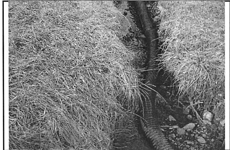
2/3/11: because water no longer flows through the upper culvert, runoff has scoured a channel across the side of the athletic field, exposing approximately 30 LF of 4" PVC drainage pipe.
