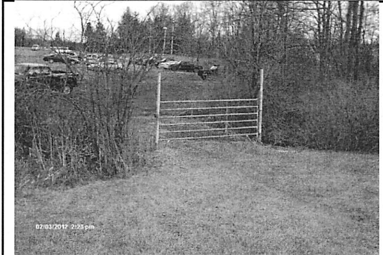
2/3/11: access road and gate used to get onto the track and field. The lower 15" CMP culvert runs under this road.
