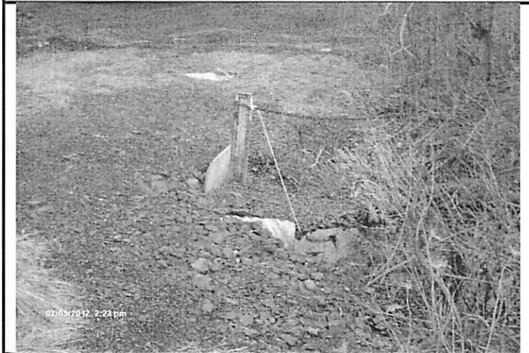
2/3/11: The northern end of the lower 15" CMP culvert, which was displaced upward by the flood waters.
