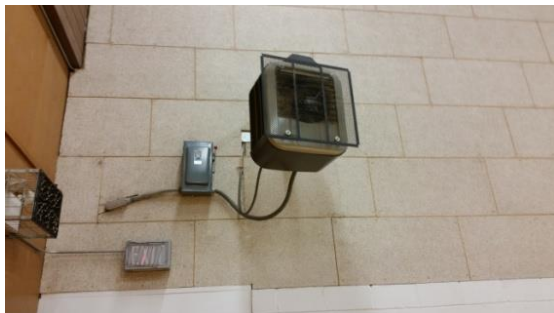
Figure 2: Electric Unit Heater in Gym
