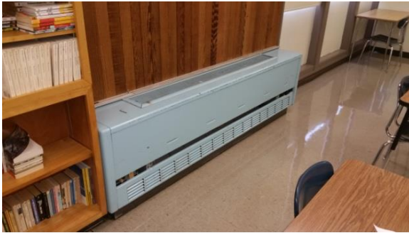
Figure 13: Older Unit Ventilator Console
