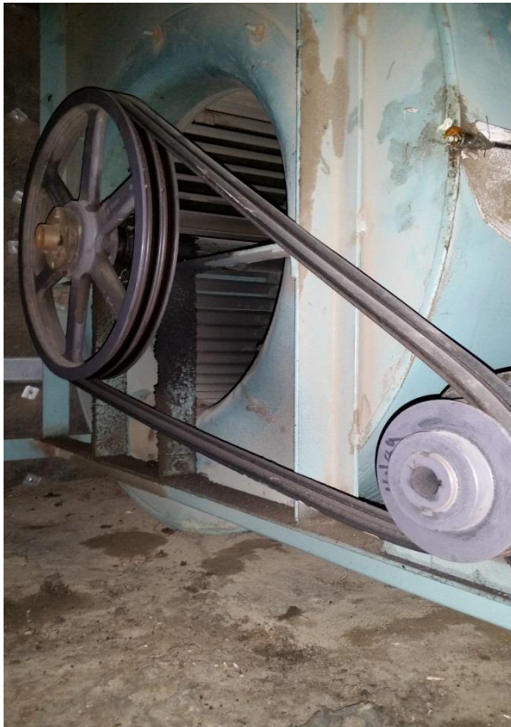
Figure 14: Gym Heating and Ventilation Unit
