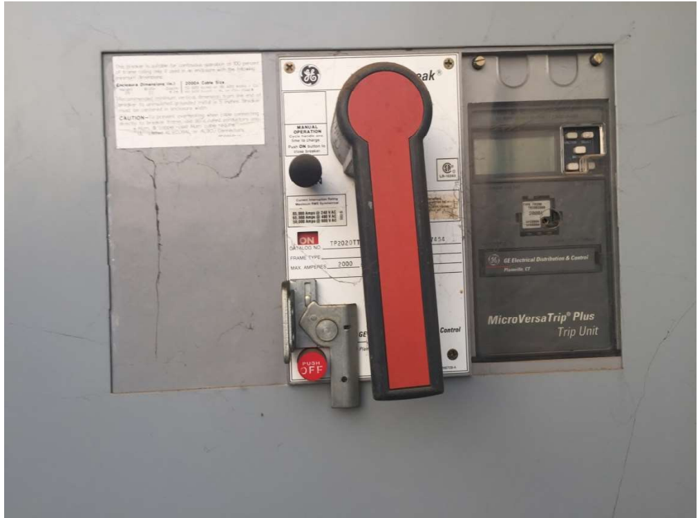
Picture 3: Main AC disconnect
