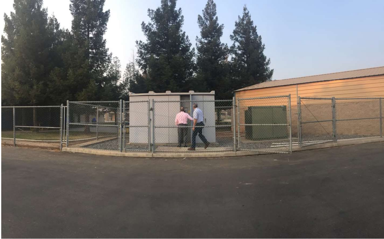
Picture 1: Gated meter switchboard yard, south of campus
