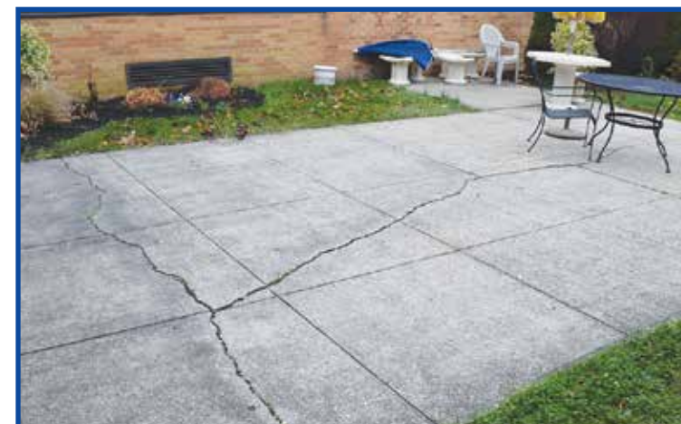
Important infrastructure will be repaired throughout the district, including parking lots, sidewalks, roofs and ceilings.
