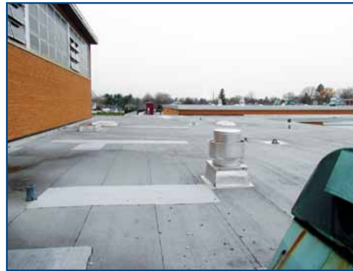
Replacement of leaking and inefficient roofs is included in the proposed work.
