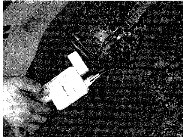
This view shows the Delmhorst Moisture Gauge verifying that the wood fiber deck is dry at Test Cut #R-8.
