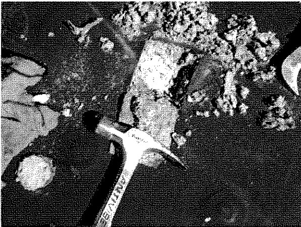
Another view of the test cut with all materials removed and the deck exposed.
