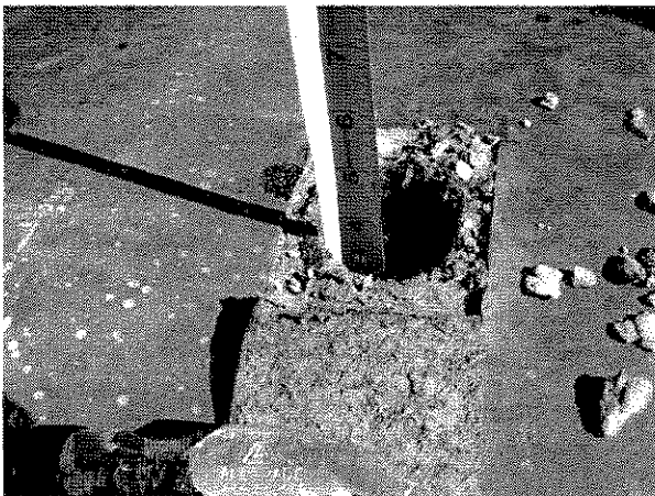
This view shows the total core was approximately 4" thick to the deck surface.
