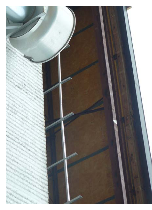
PHOTO OF FASCIA FROM PREVIOUS PHASE. IN SOME AREAS BAR JOINT ENDS MAY PROJECT PAST THE BEAM AND BE PACKED OUT IN BETWEEN
