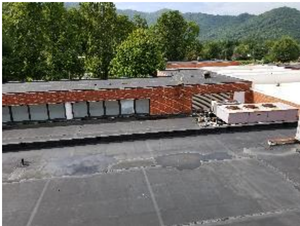
Photo #3 View of the roof system over the eastern portion of the building.
