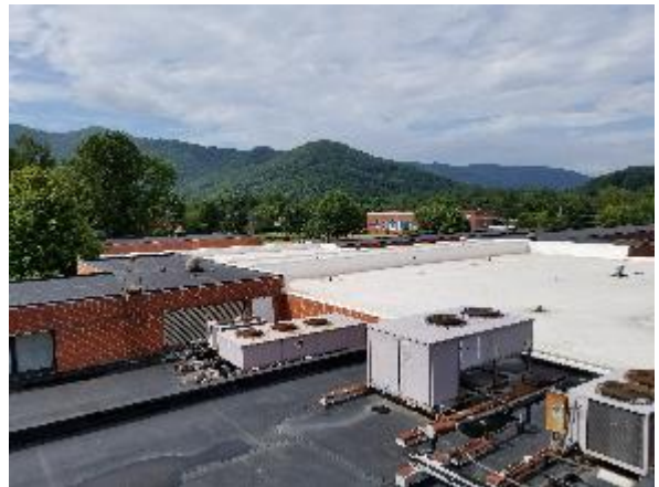
Photo #4 View of the center roof section (not in scope) and the western roof sections.
