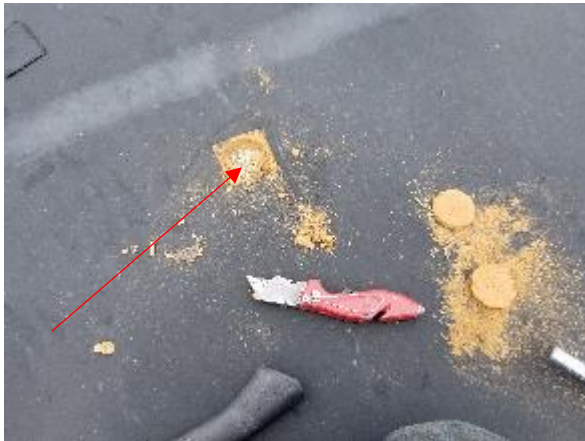
Photo #9 View of non-suspect roof materials (wood-fiber insulation and Tectum®) on the high-bay gym roof.
