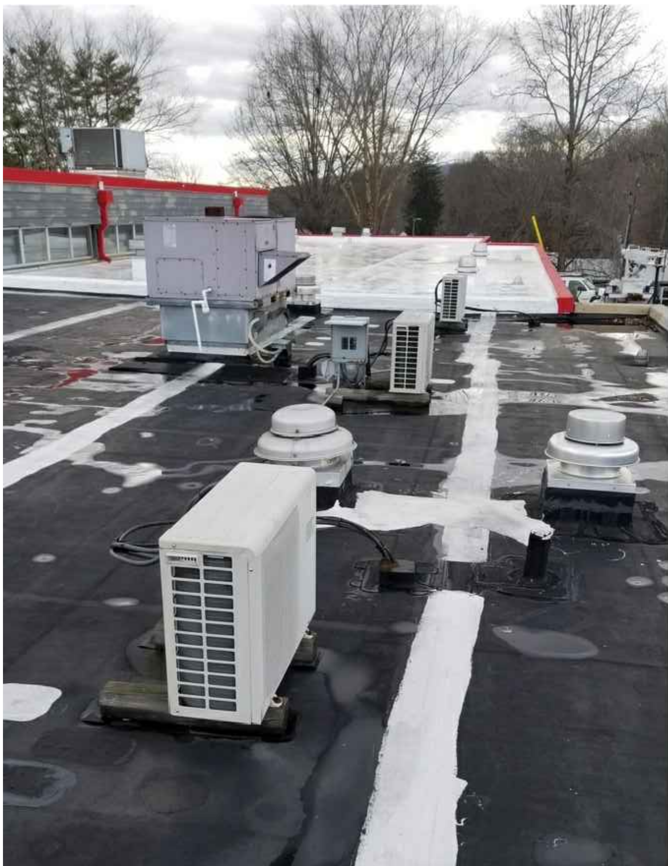
8 Rooftop Condensing units to be raised or disconnected and installed on new sleeper curbs. Contractor is responsible for replacing any damaged lines. NTS
