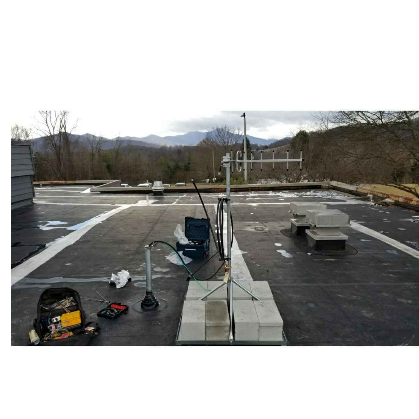
7 BDA Antenna on ballast base will need to be disconnected by the BDA company. Once roofing has been accomplished, will need to be reinstalled by BDA company. NTS
