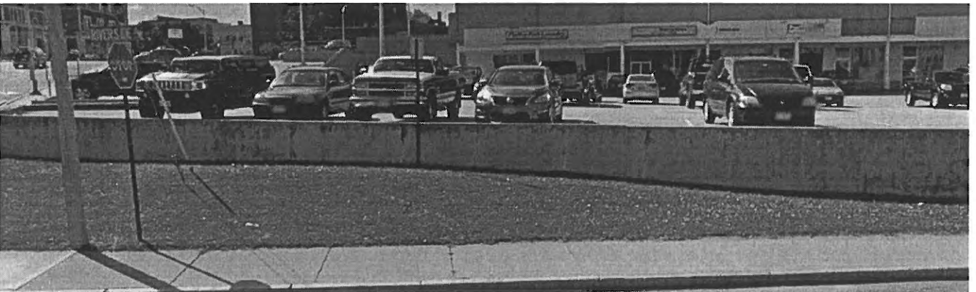
Photos of wall along Riverside Avenue showing cracked, chipped and spalling concrete
