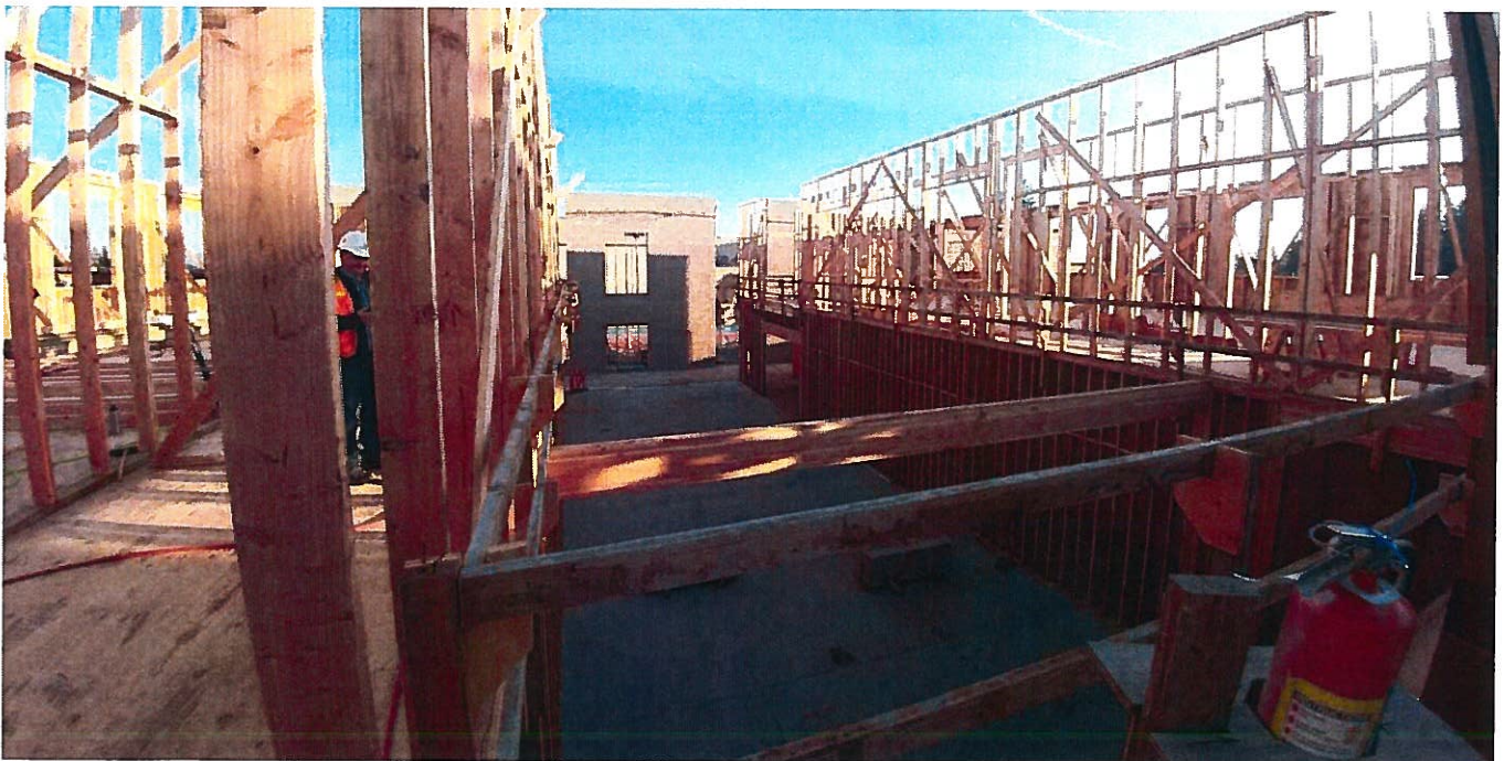
RHS – Second floor framing. All structural is in place and infill framing starting. The lower photo is the look down into the new media center.
