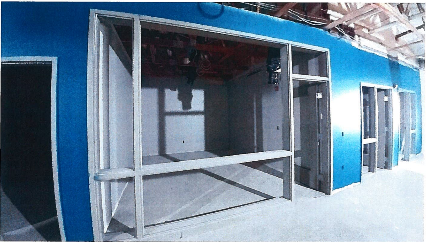
Old VRMS (New Services Center) – City offices painted and interior frames set. Glass and doors set to arrive next week.
