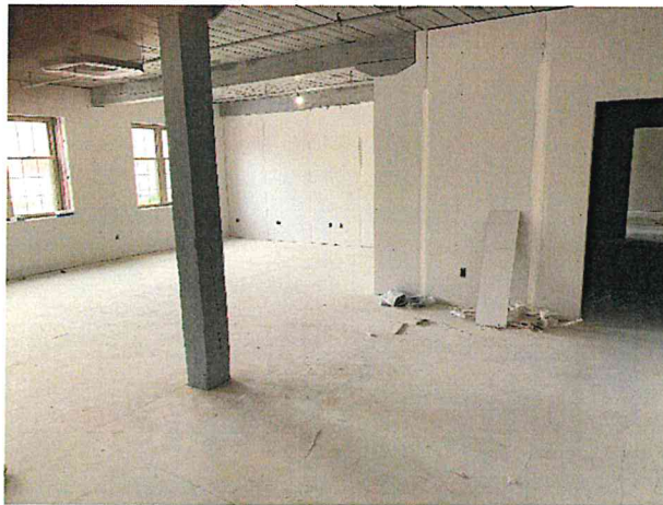
LPN Clinical Lab at the Gateway. The walls are rocked and taping is in progress. (4/28/23)
