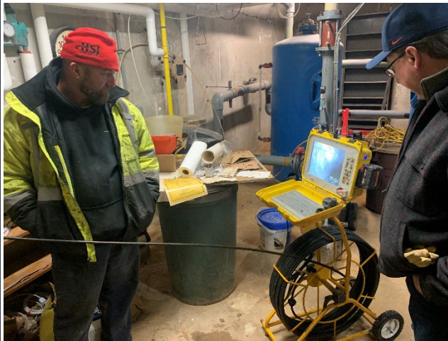
Engineers use a jet cleaner and video scope to inspect the foundation drains near the basement at the WEB.
