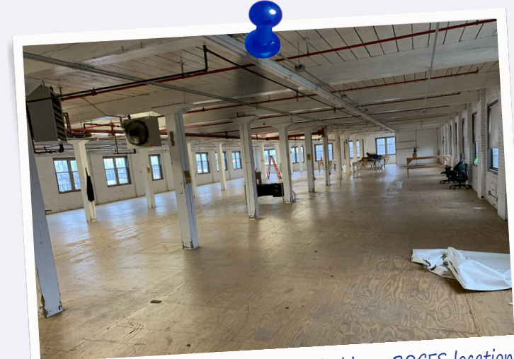
This is the “before” picture of the Herkimer BOCES location on the second floor of 420 E. German St. in Herkimer. Arc Herkimer began construction here on Jan. 16, and the work is expected to be completed in April..
