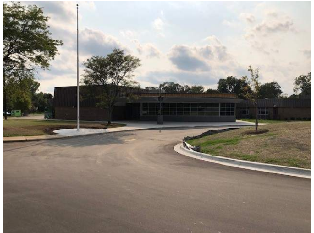
New asphalt pavement, flagpole and sidewalks are complete at the new Secured Entry Addition. Only exterior metal panels at the Canopy are remaining to be installed
