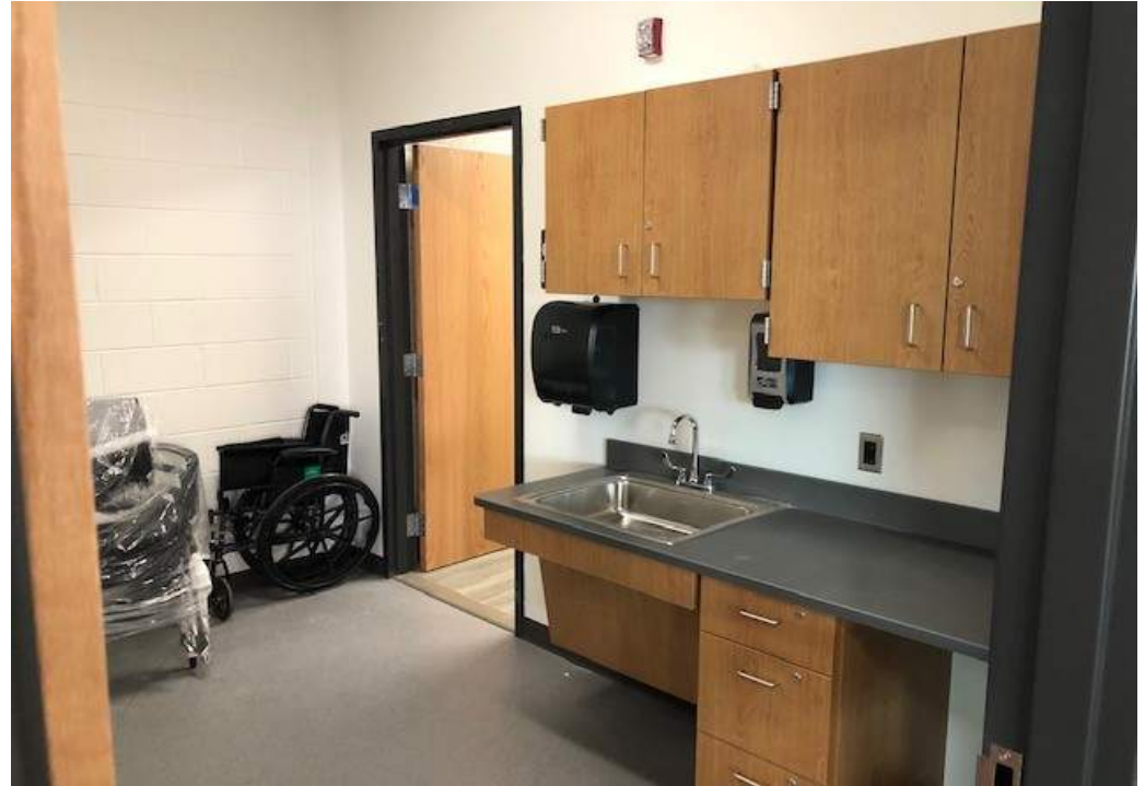
Millwork and sink are installed in the new Clinic Room within the Secured Entry Addition
