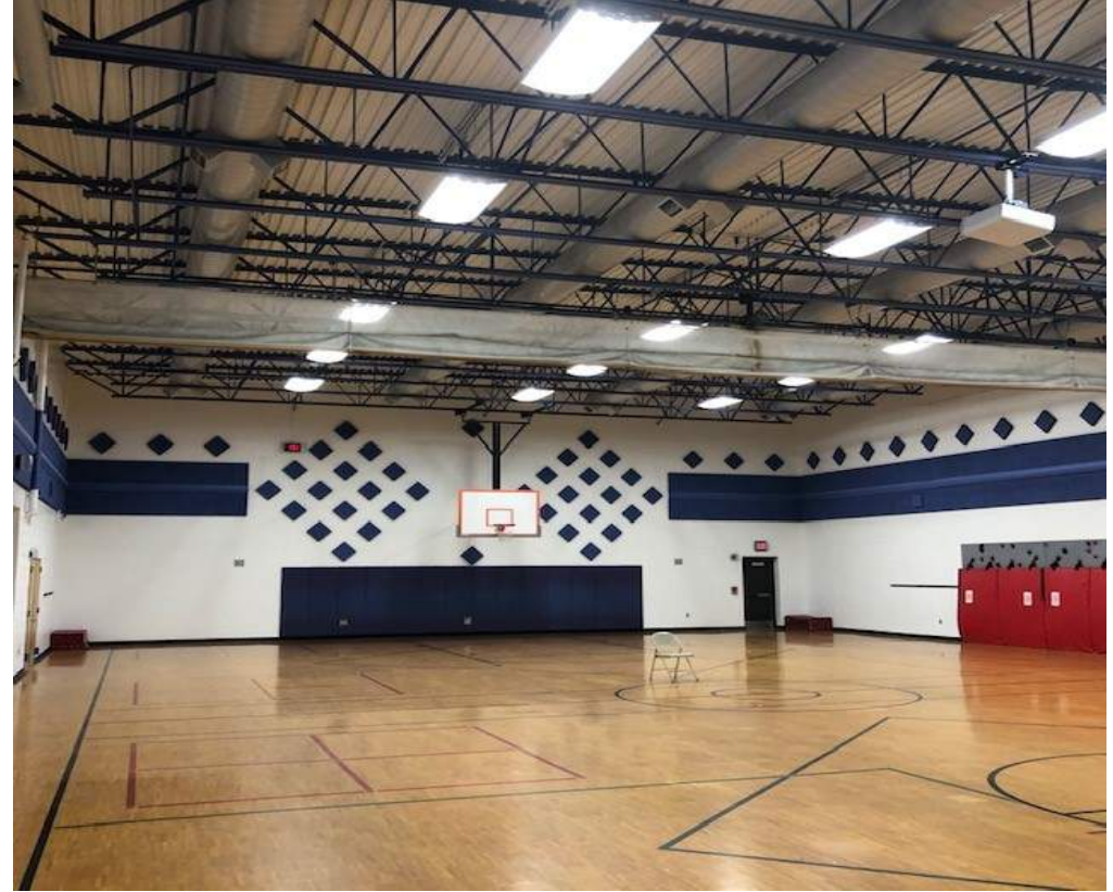
Existing gymnasium has been repainted and new acoustical wall panels and wall pads have been installed
