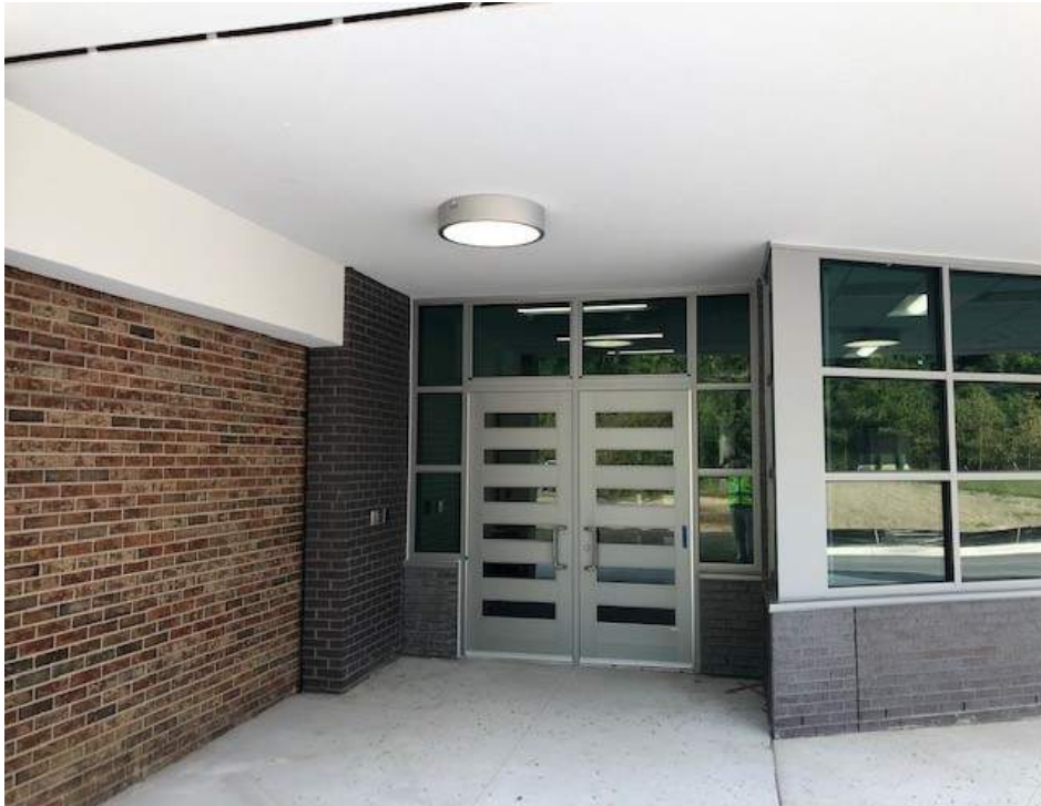
The new main entrance doors as part of the Secured Entry Addition are in place and the card reader and intercom are operational
