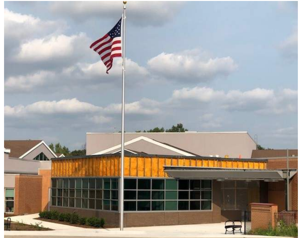
The Secured Entry Addition is nearing completion pending installation of the exterior metal panels, main entrance vestibule doors and new roof top mechanical unit for ventilation
