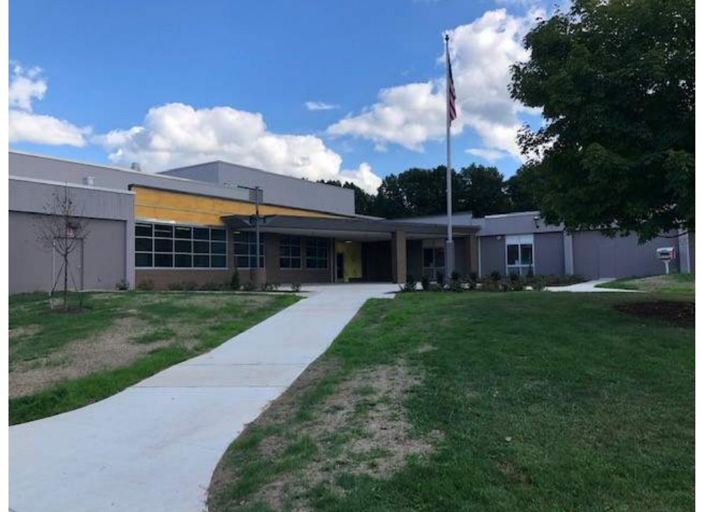
The Secured Entrance Canopy Addition is nearing completion pending installation of the exterior metal panels and main entrance vestibule doors.
