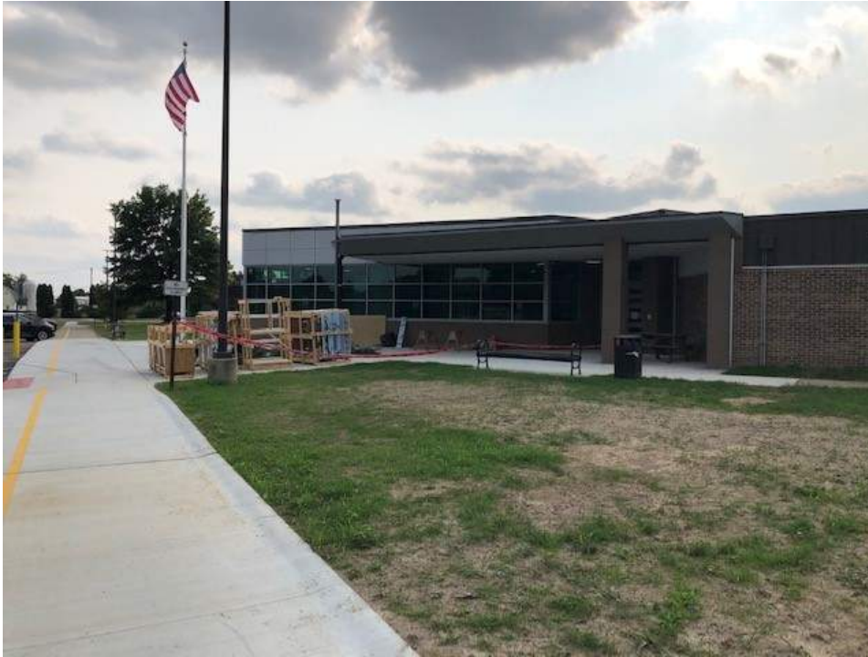
Secured Entry Addition main entrance. New benches and flagpole are in place.
