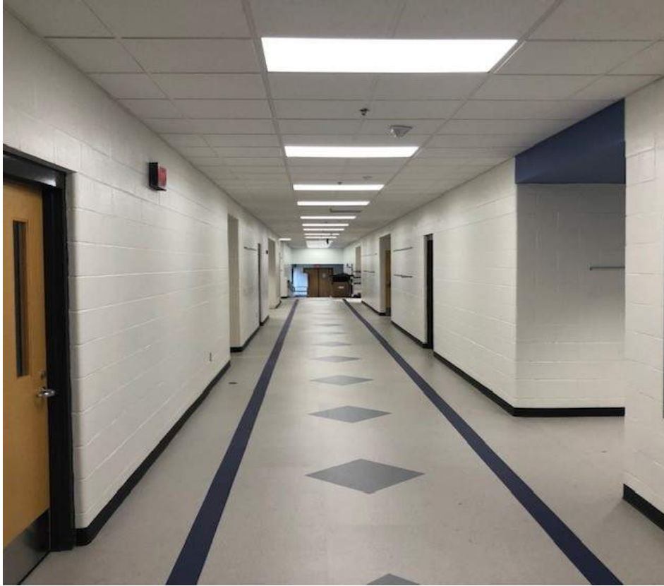
New ceilings, lighting, painted walls, LVT flooring and base is complete in the Corridors
