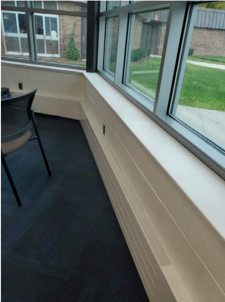
New Runtal heating panel in the secured entry addition.
