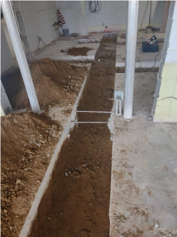
Underground plumbing trenches at interface with the Secured Entry Area are prepared for concrete infill
