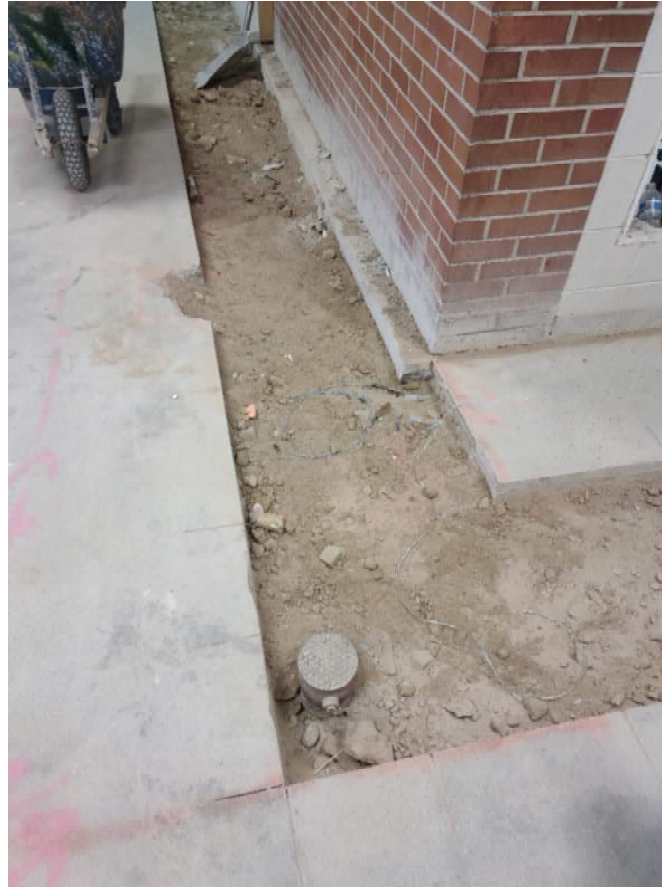
Underground going in the hallway between the office area and the secured entry.
