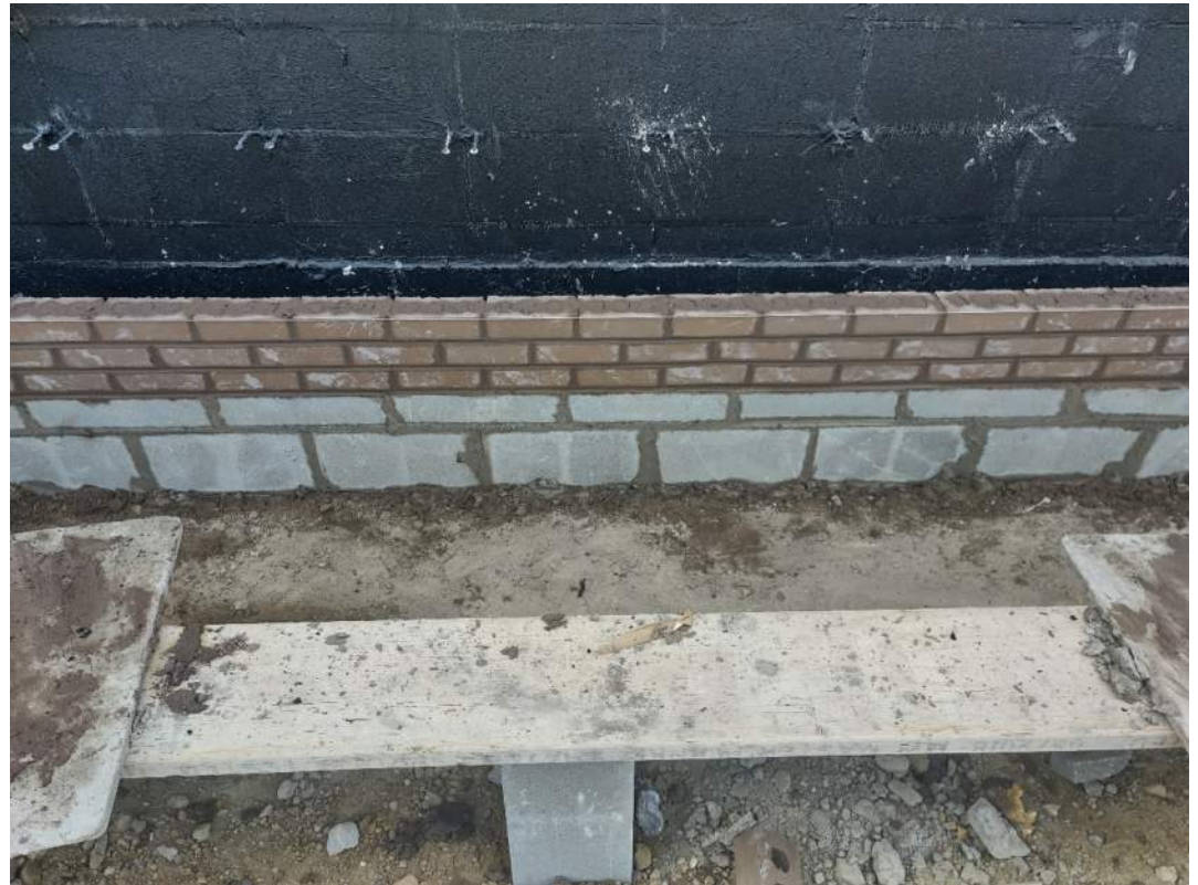
Masonry brick is being put in place for the new secured entry.
