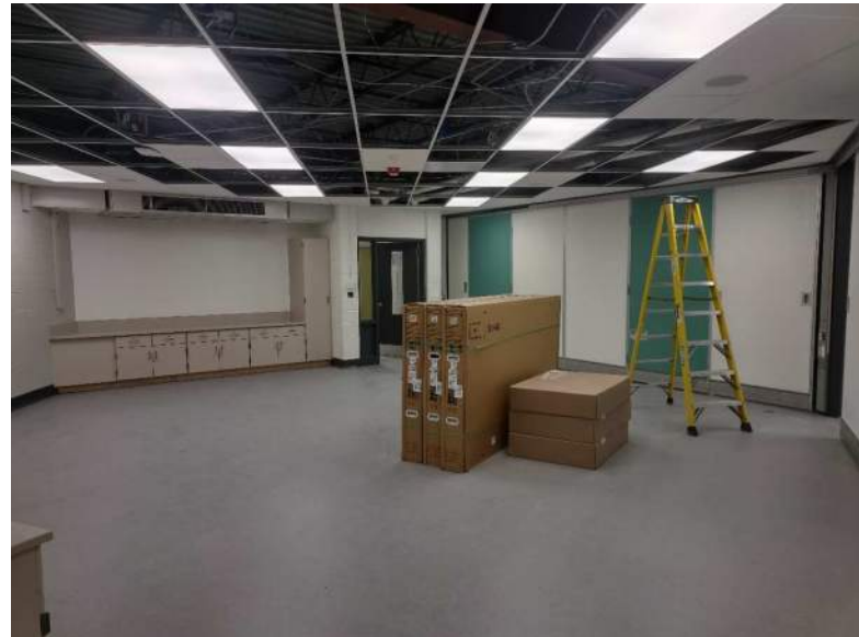
Flooring is completed in the classrooms and full ceiling tiles are being installed
