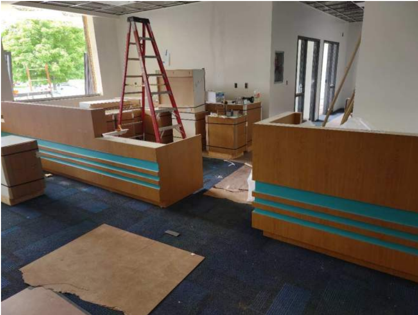
Secured entry office area carpet has been installed and casework is being set in place
