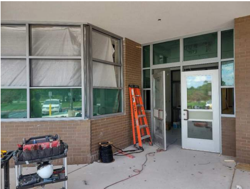
Window framing and glass is being installed at the Secured Entry Addition
