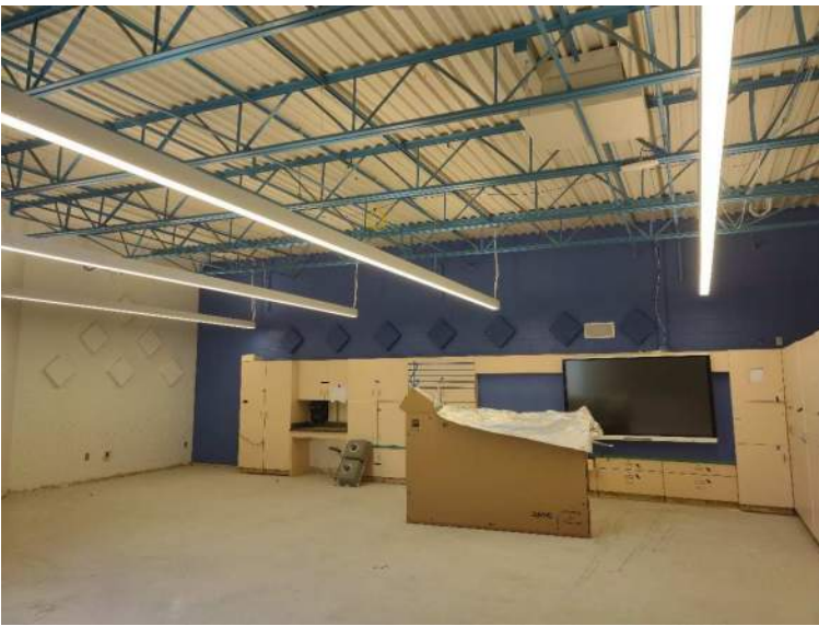
Smart Board installed in the Music room
