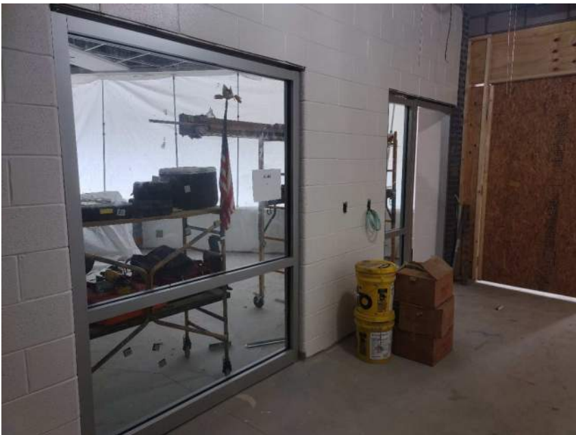
Secured Entry Addition aluminum framing and glass at interior openings is being installed
