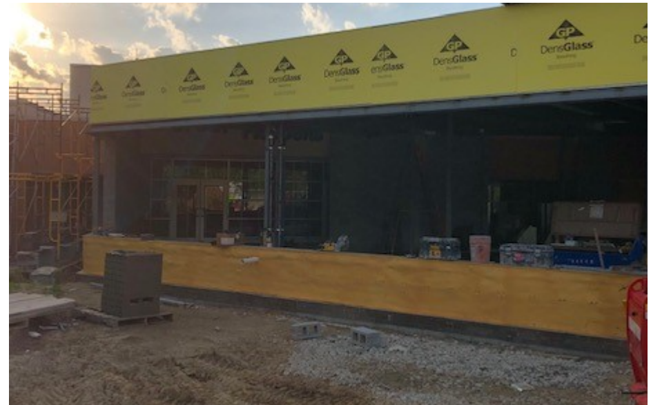
Spray foam insulation is completed in preparation for face brick at exterior walls and densglass installed.
