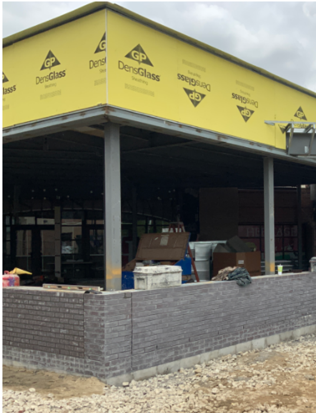
Face brick laid at new addition and Densglass Sheathing put in place on exterior walls.
