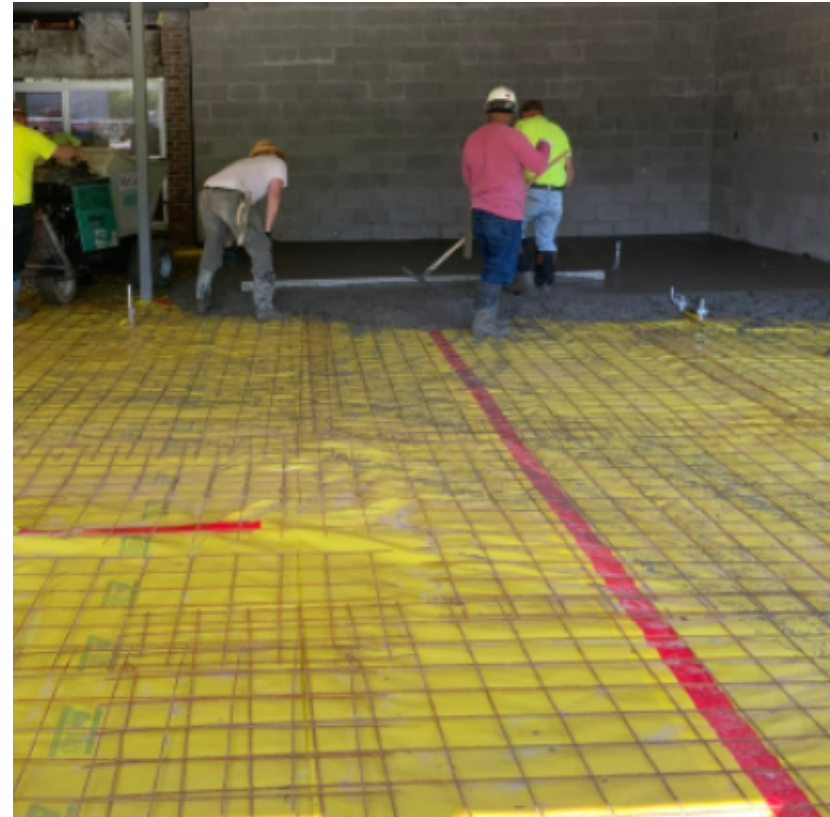
Concrete floor slab being poured and leveled in the Secured Entry Addition
