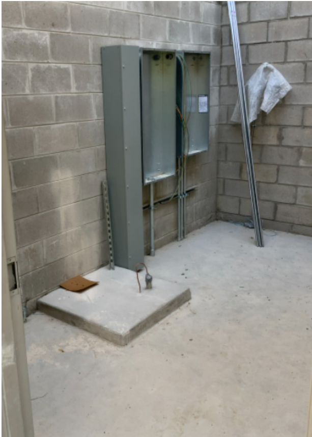
Electrical panel boxes installed, and equipment pad is ready for transformer
