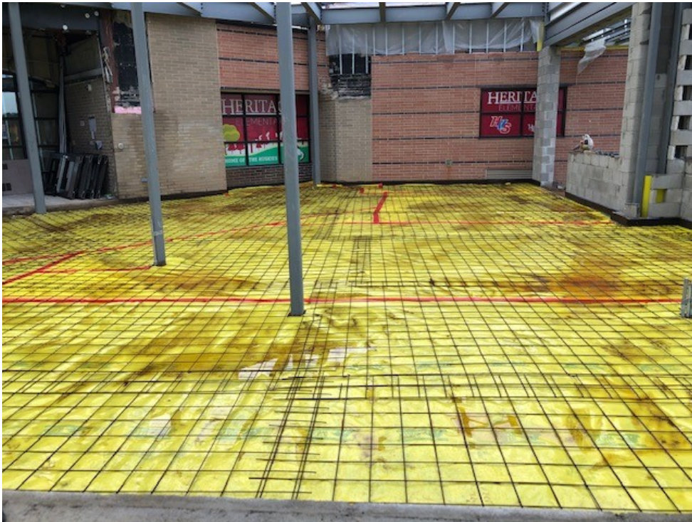
Vapor barrier and reinforcing steel are in place ahead of concrete floor slab pour
