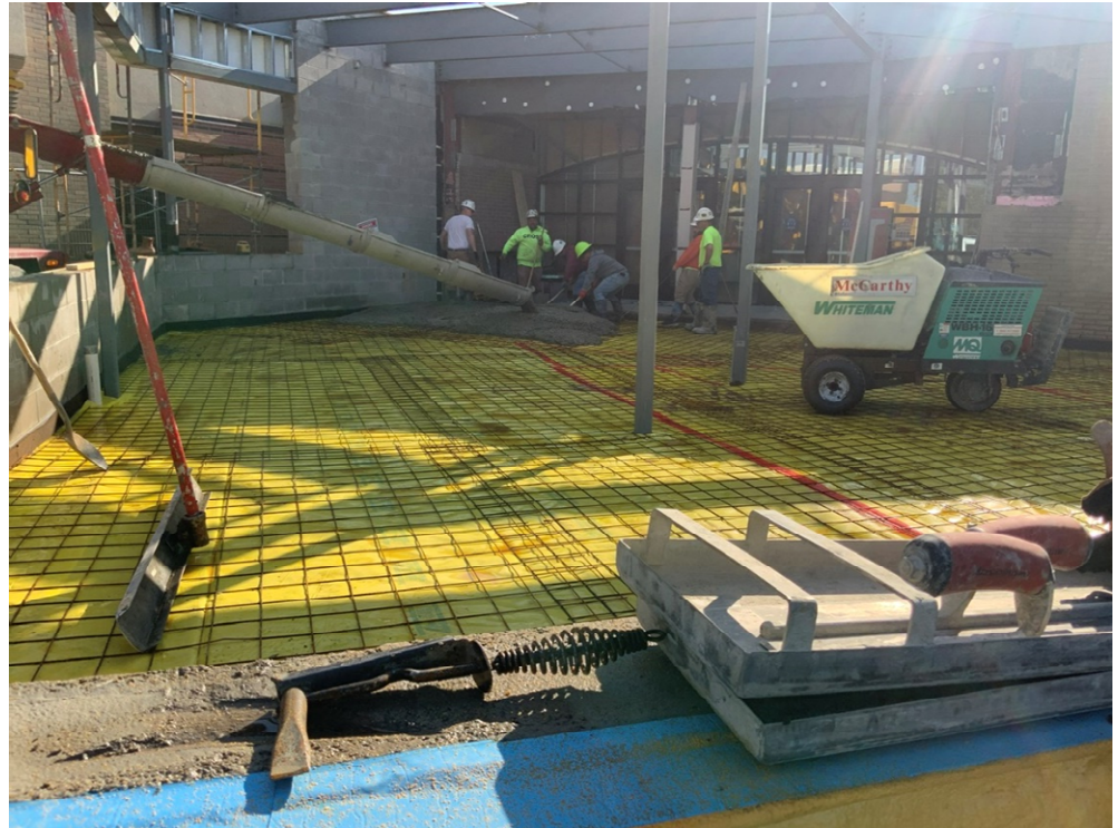
Concrete floor slab being poured and leveled in the Secured Entry Addition
