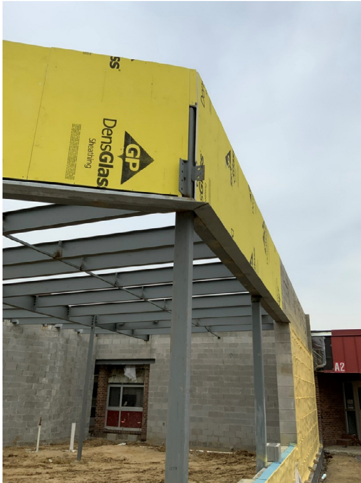
Densglas sheathing, damp proofing and spray foam insulation are put in place ahead of face brick installation
