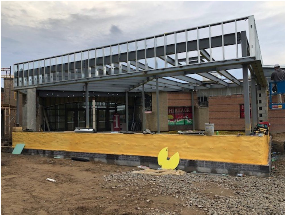
Cold formed metal framing is being installed for the new Secured Entrance Addition
