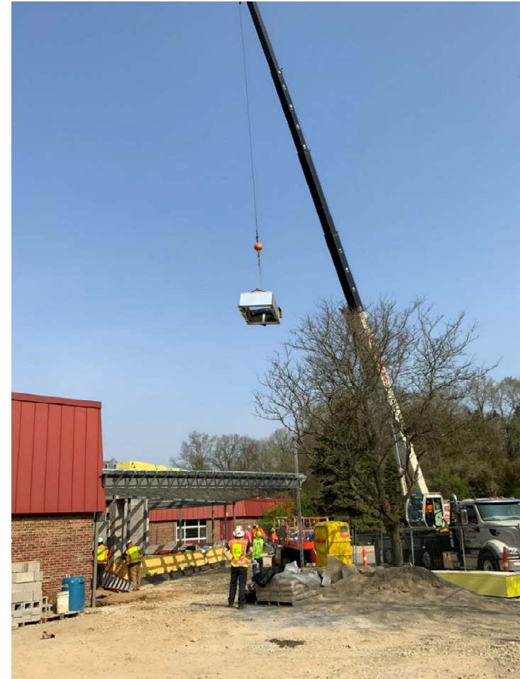
Curb for support of new roof top air handling unit to serve the Secured Entry Addition is being set in place
