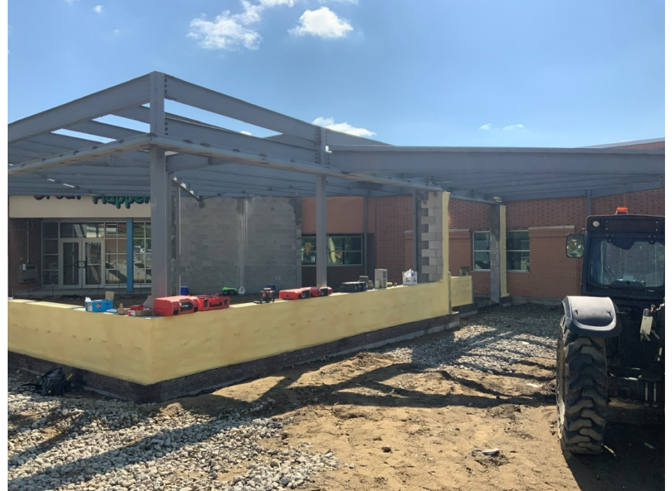
Spray foam insulation is completed in preparation for face brick at exterior walls
