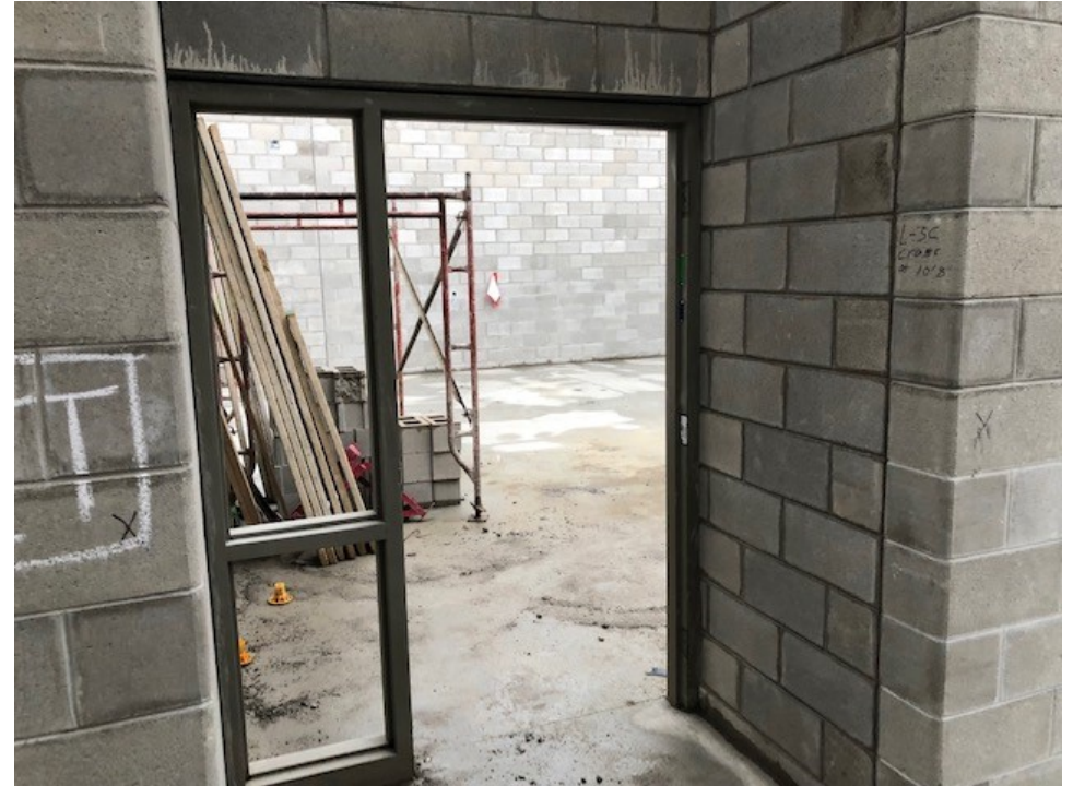
Interior door frame with sidelight is set for the new Art Classroom.
