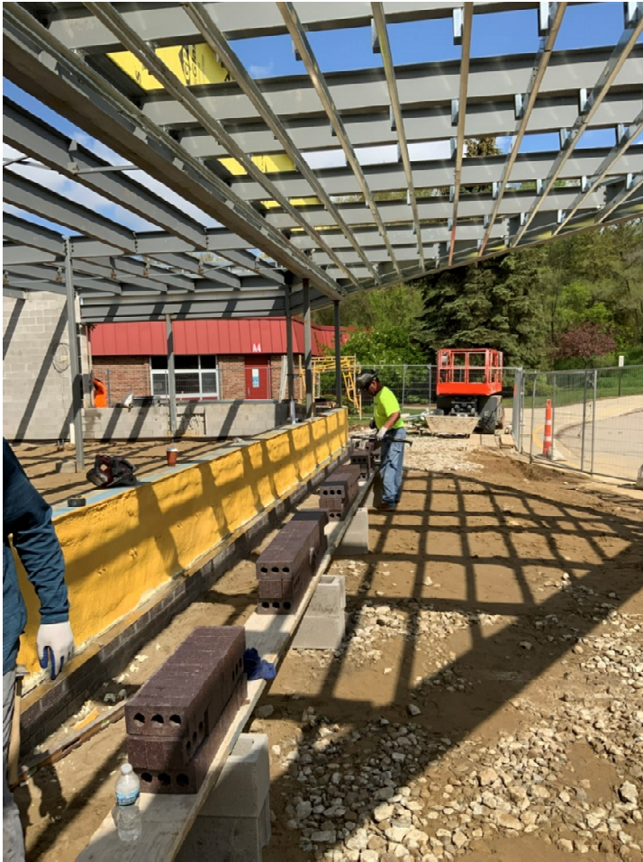
Masons preparing to lay face brick on the exterior walls of the new Secured Entry Addition.
