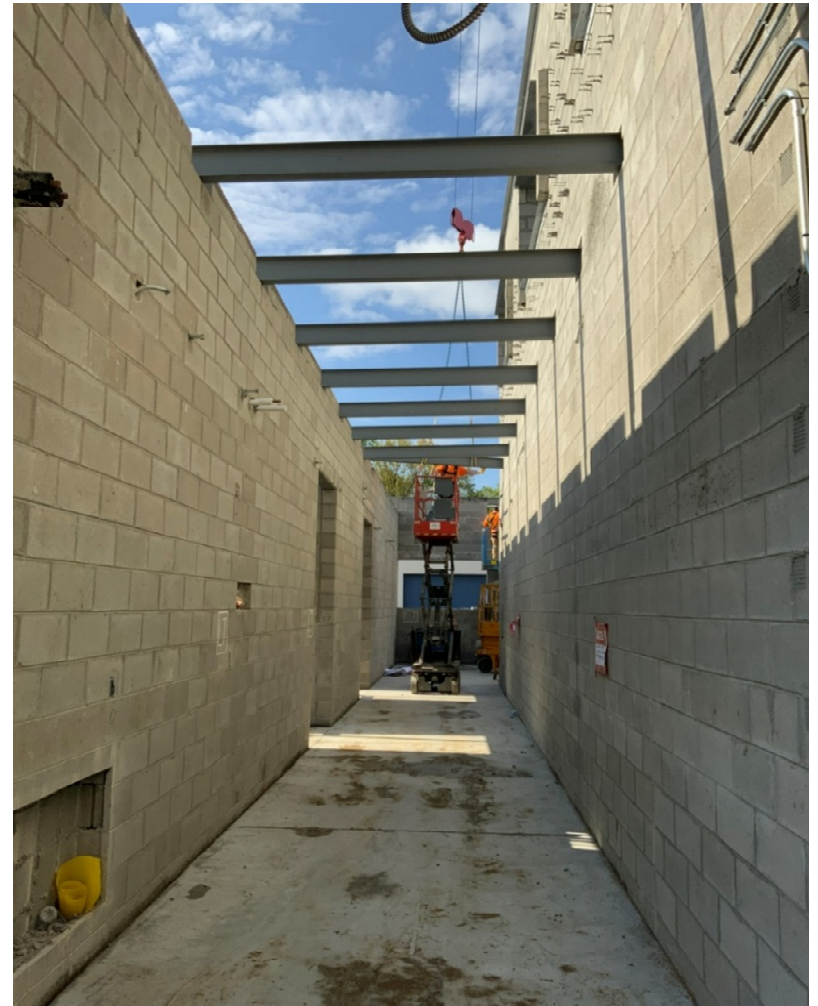
Steel Beams put in place and being installed in the Corridor outside of the gymnasium and two new classrooms
