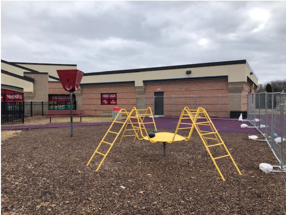
Secured Entry Addition – Temporary Fencing is in Place Around a Portion of Playground. Bench and Ball Hoop to be Removed and Salvaged for Relocation
