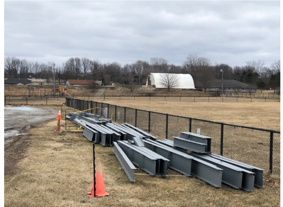
Secured Entry Addition – Structural Steel Framing Material Has Been Delivered to the Site
