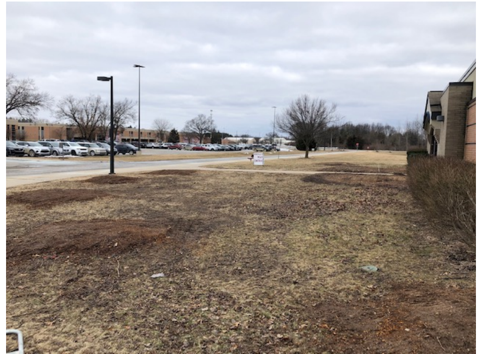
Secured Entry Addition - Trees Removed on West Elevation Adjacent to Temporary Main Entrance
