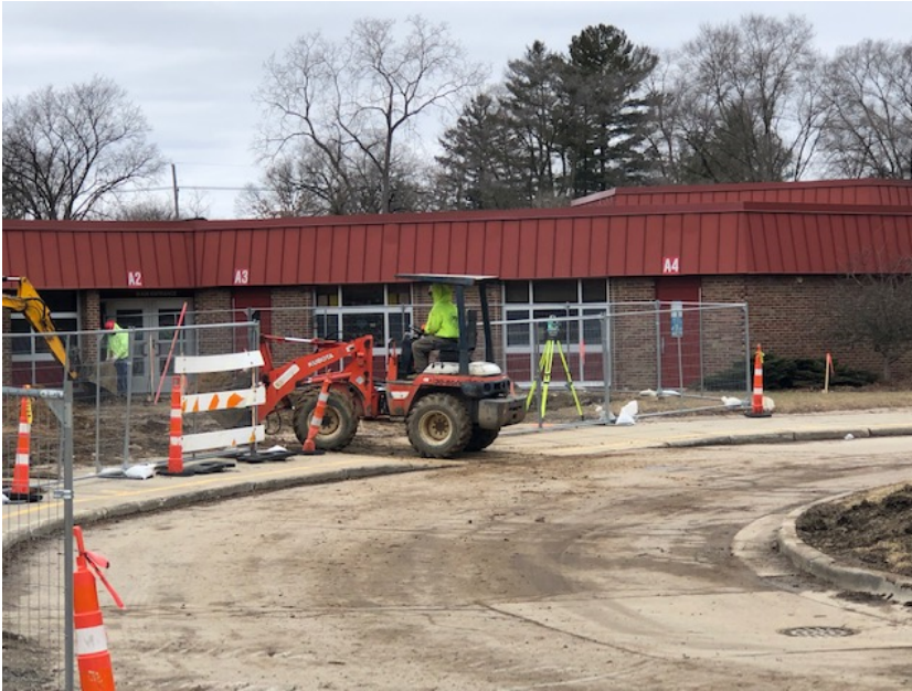
Secured Entry Addition – Temporary Fencing is in Place and Foundation Work is Underway
