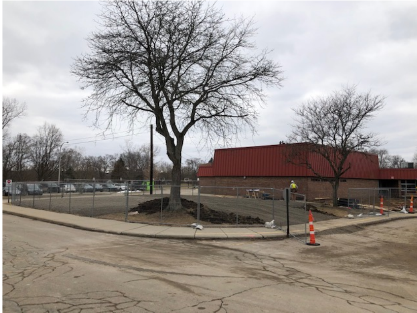
Secured Entry Addition – Staging Area is Established, and Temporary Fencing is in Place
