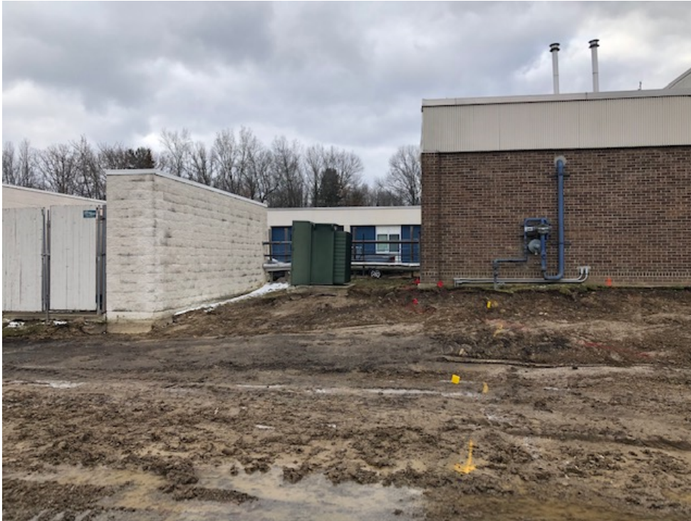
Gymnasium & Classroom Addition – Site Clearing is Complete Except For Removal of Existing Chiller Enclosure
