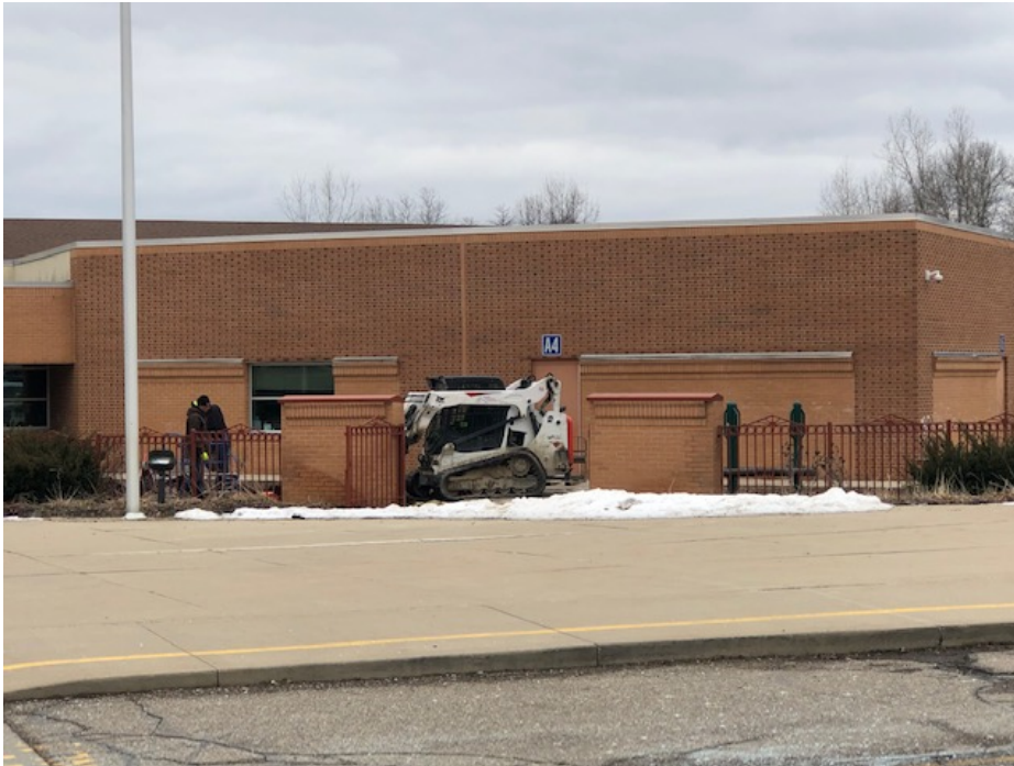
Secured Entry Addition - Removal and Salvaging of Existing Playground Equipment for Relocation
