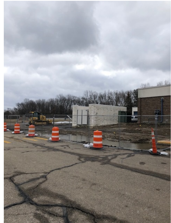
Gymnasium & Classroom Addition – Temporary Fencing to Secure the Site is in Place
