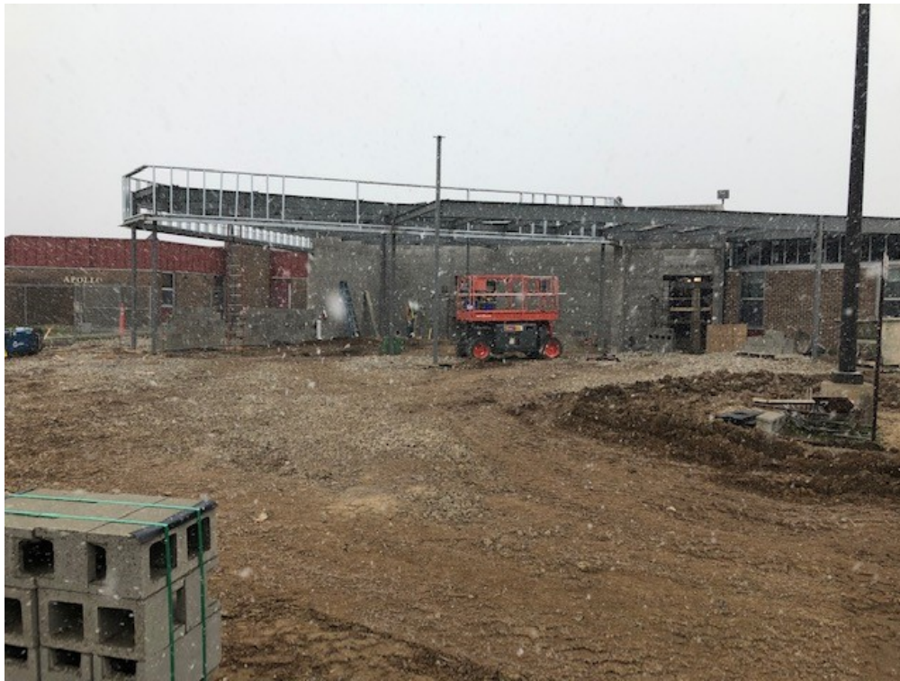
Steel Erection for Secured Entry Addition is complete and exterior cold formed metal framing has started
