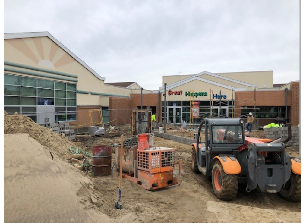
Steel columns are set, and masonry walls are being built for Secured Entry Addition
