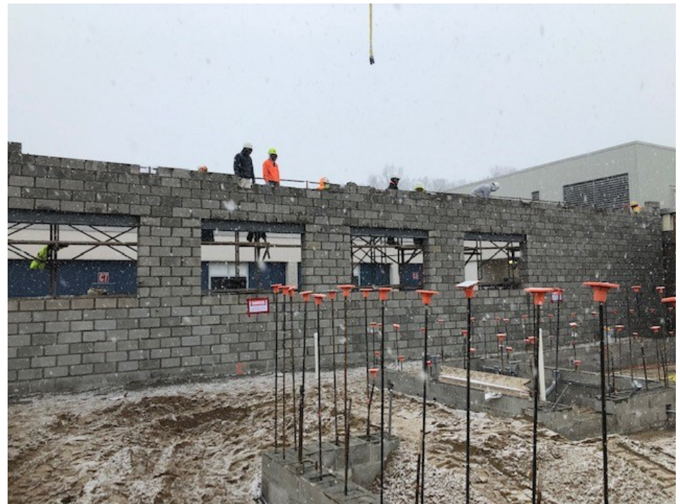
Masonry wall along the south side of the Gymnasium and Classroom Addition is under construction
