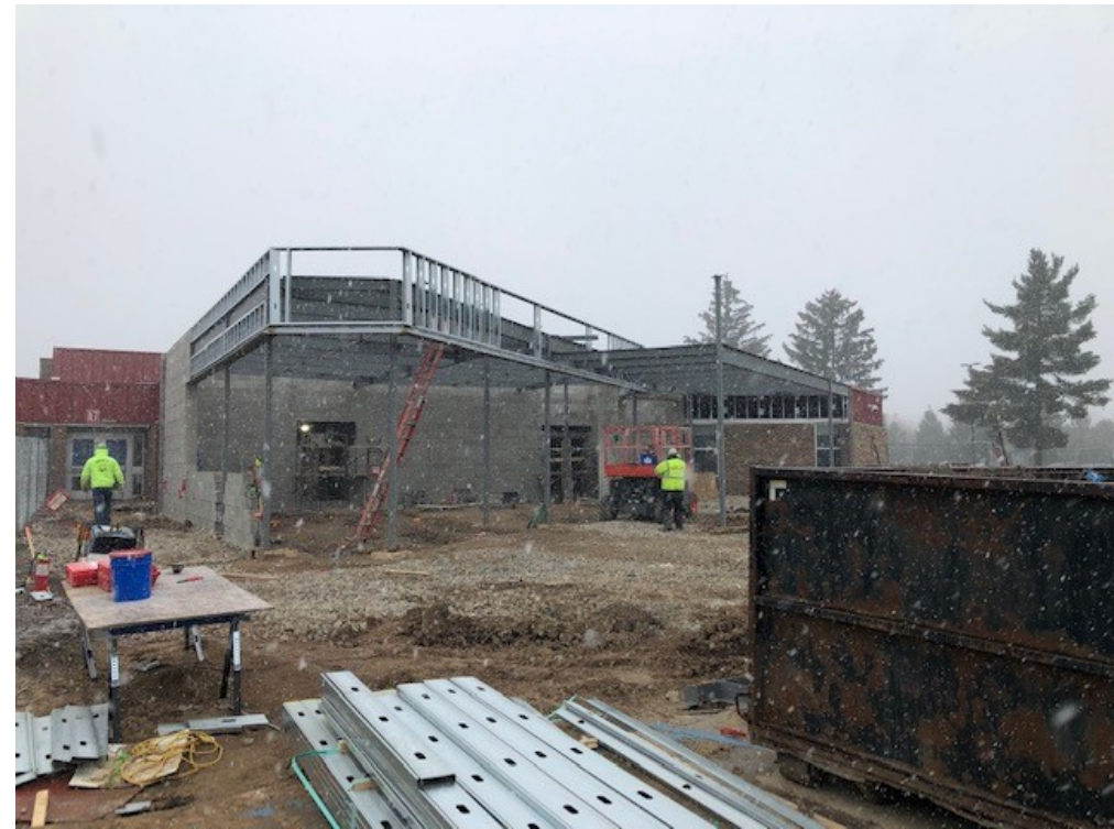
Steel Erection for Secured Entry Addition is complete and exterior cold formed metal framing has started
