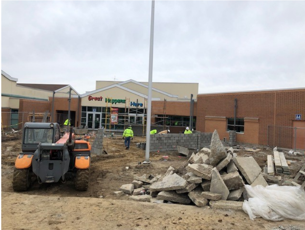
Steel columns are set, and masonry walls are being built for Secured Entry Addition
