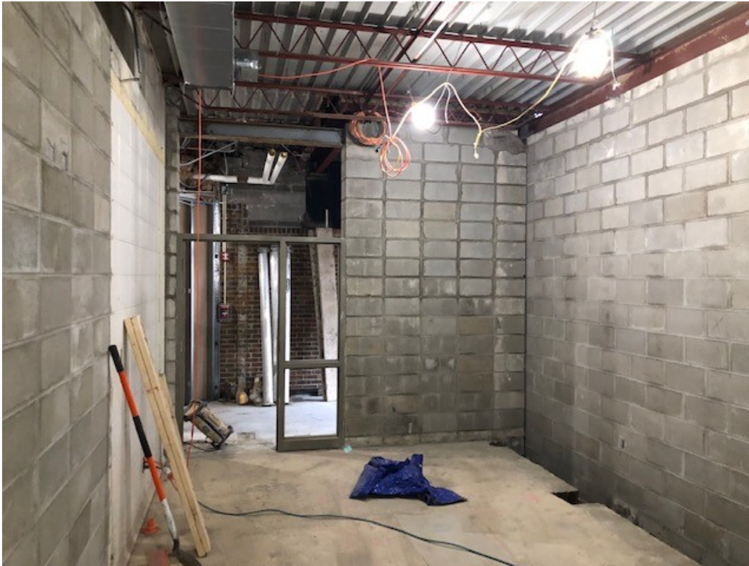
Masonry walls and hollow metal door frame and sidelight are set for Conference Room B150
