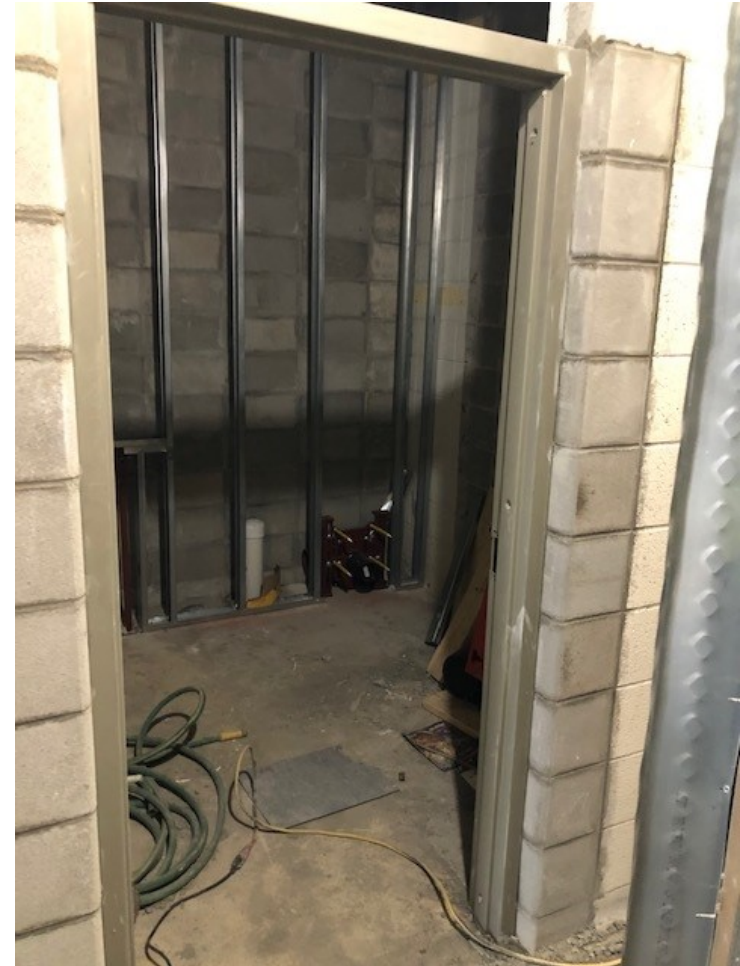
New masonry walls, hollow metal door frame and plumbing rough-in for Adult Toilet B149
