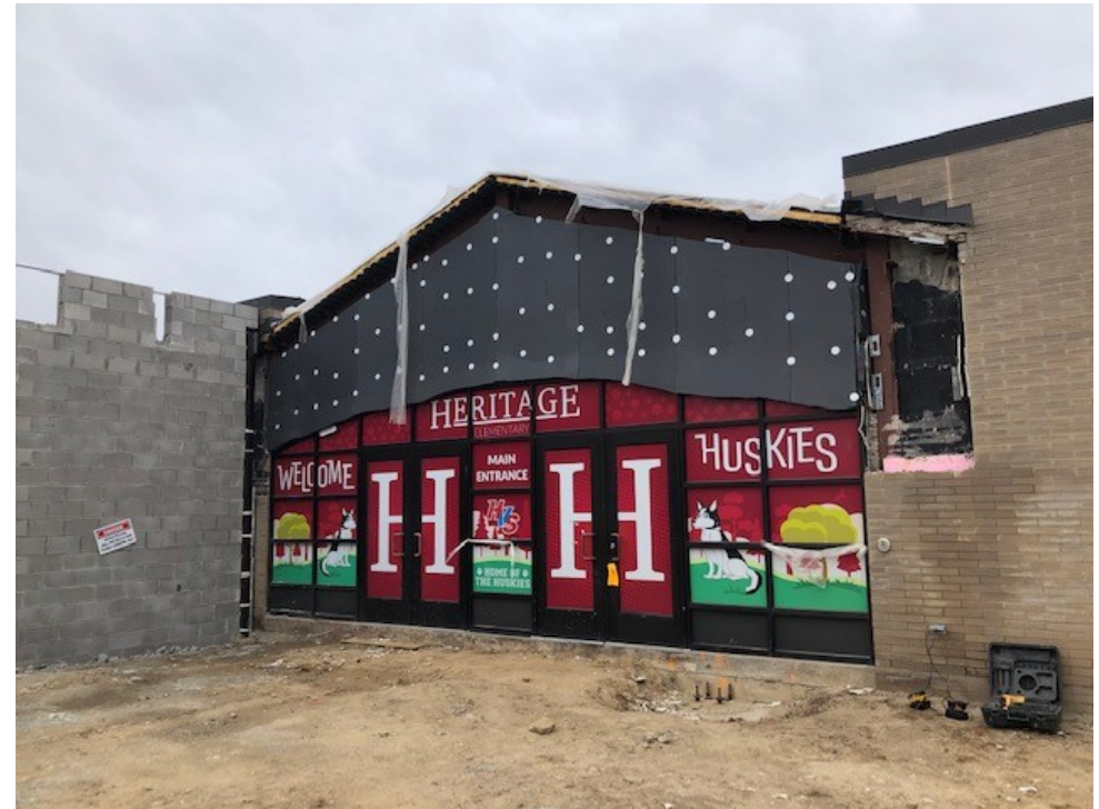
Temporary enclosure is in place at interface of existing school with the new Secured Entry Addition
