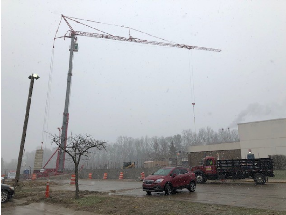
Brazen and Greer Masonry has mobilized a tower crane to facilitate masonry wall construction for the new Gymnasium and Classroom Addition
