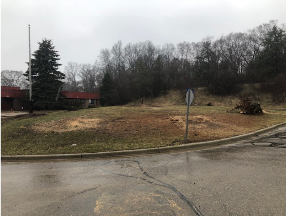
Site clearing and tree removal at island is completed in preparation for reconfigured drop off
