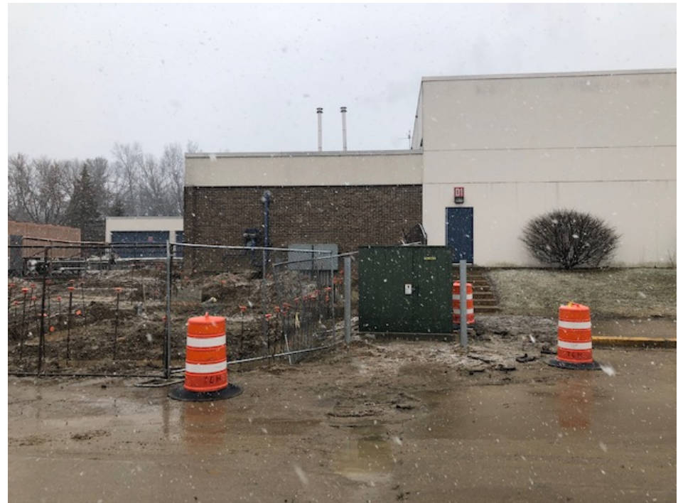
DTE Transformer has been relocated
