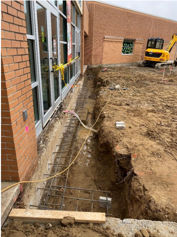
Secured Entry Addition – Excavation for addition foundations is ongoing, foundations will be poured over the new few days.
