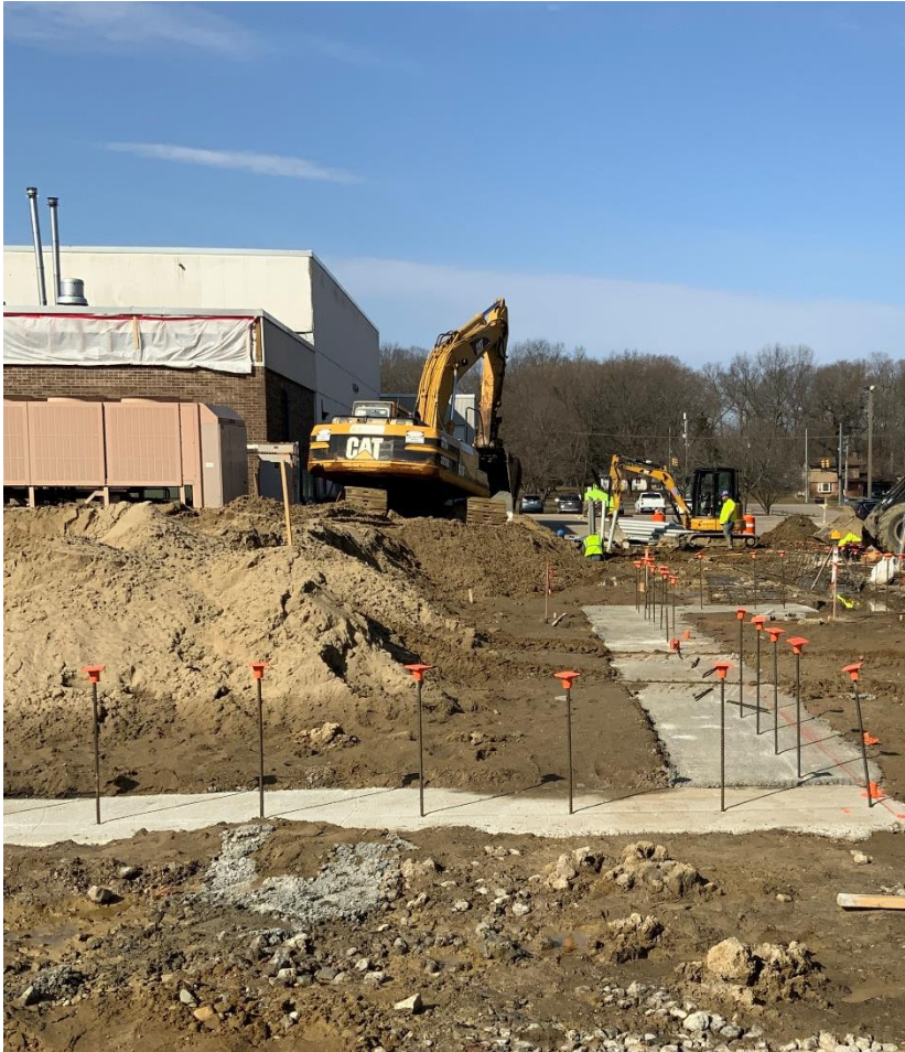
Gymnasium & Classroom Addition – Foundations have been poured and ready for masonry walls.
