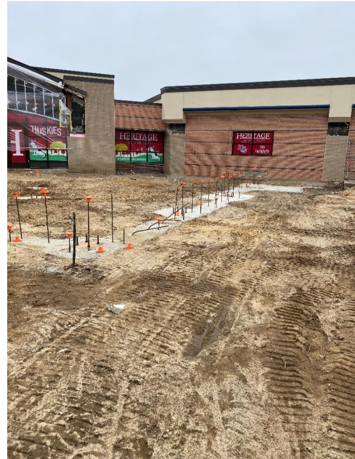
Secured Entry Addition – Foundations are installed and ready for masonry walls to begin.
