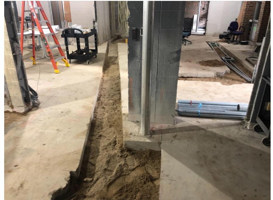
Existing Office – Foundations being prepped to support new interior masonry walls in the office area.
