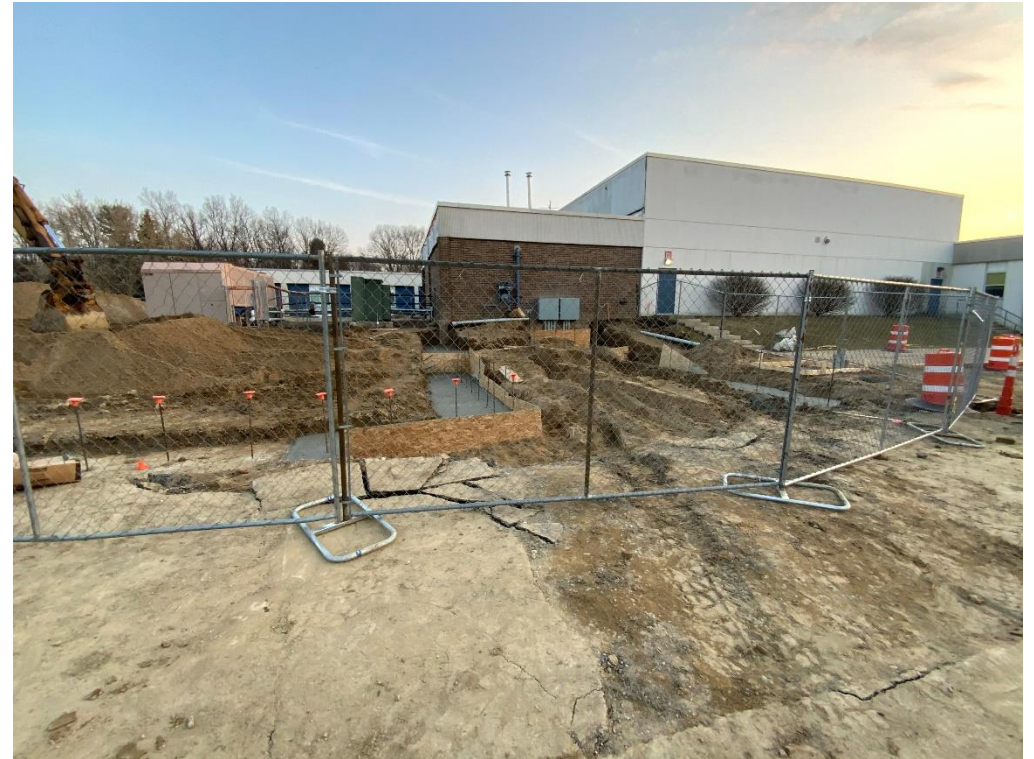
Gymnasium & Classroom Addition – Electrical main has been relocated and foundations have been poured.
