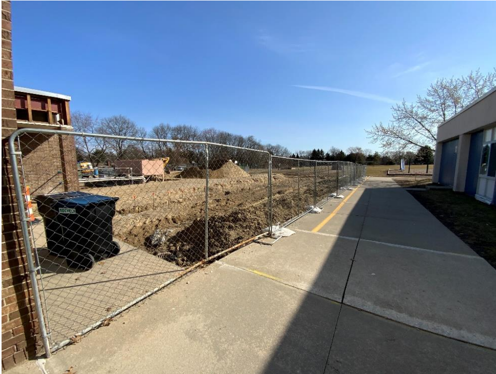
Gymnasium & Classroom Addition – Temporary Fencing to Secure Material and Equipment Staging Area is in Place and Sand Material Has Been Delivered
