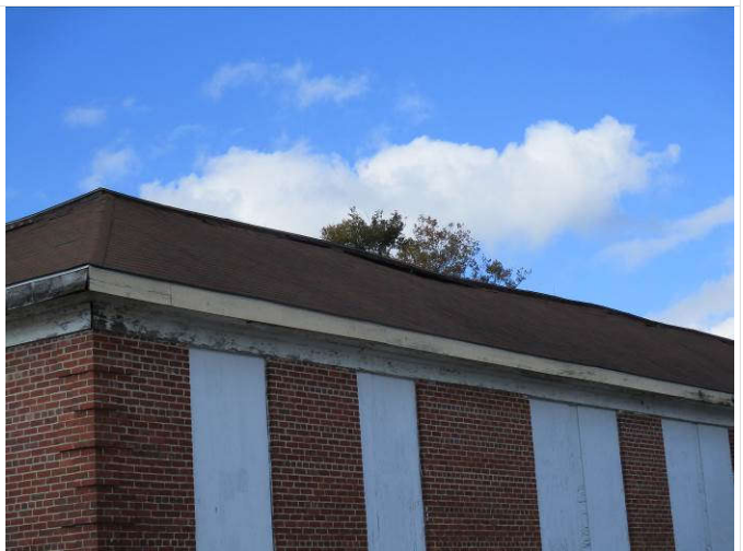
12. View of roof damage on administration building.
