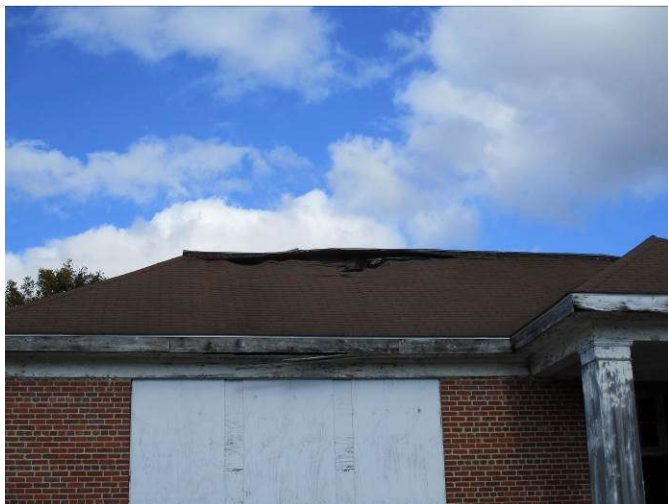
11. View of roof damage on administration building.
