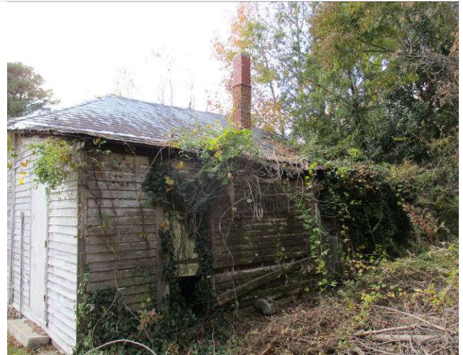
16. View of asbestos roofing on the north side of the dining room/kitchen building.
