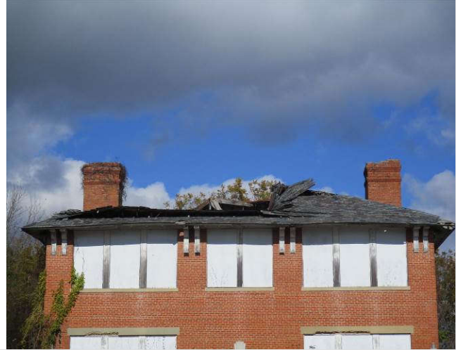
2. View of damaged roof on main school building.
