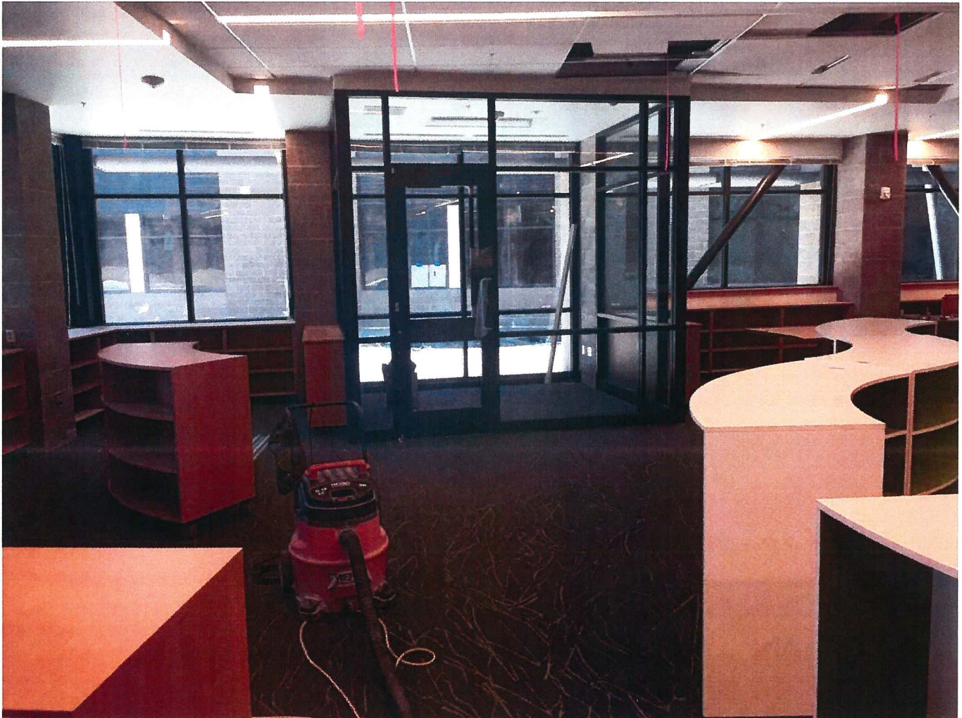
SRIS / VRMS – Media Center – Interior glass finishing, furniture distributed, final cleaning taking place.
