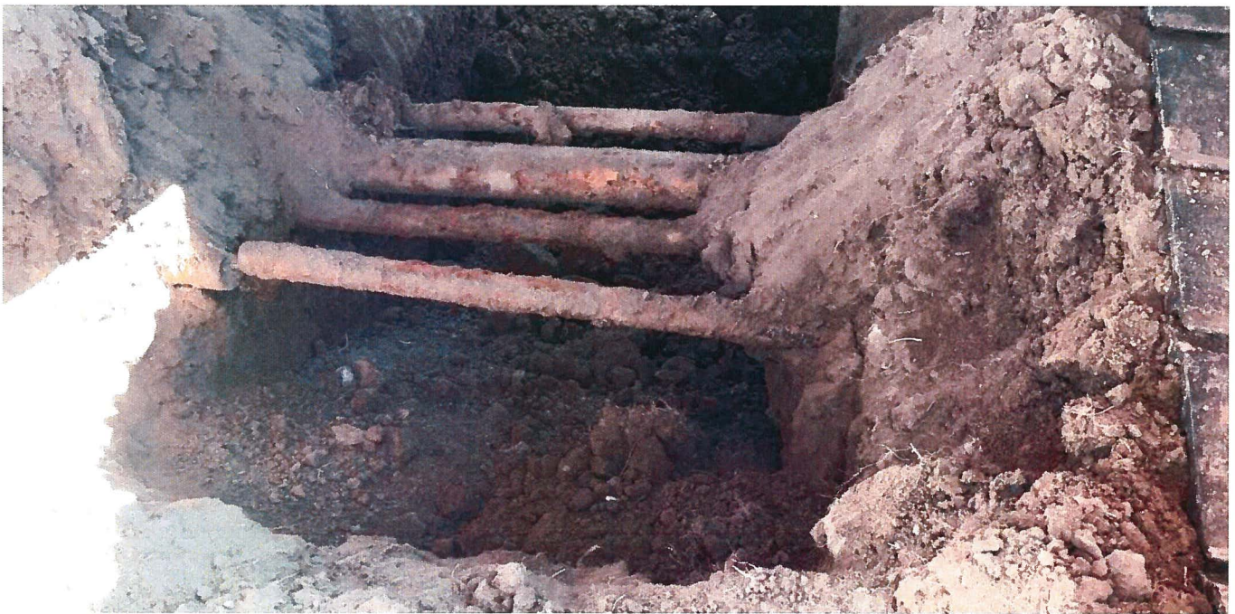
HIGH SCHOOL – This is what most photos look like right now – finding utilities known and unknown.
