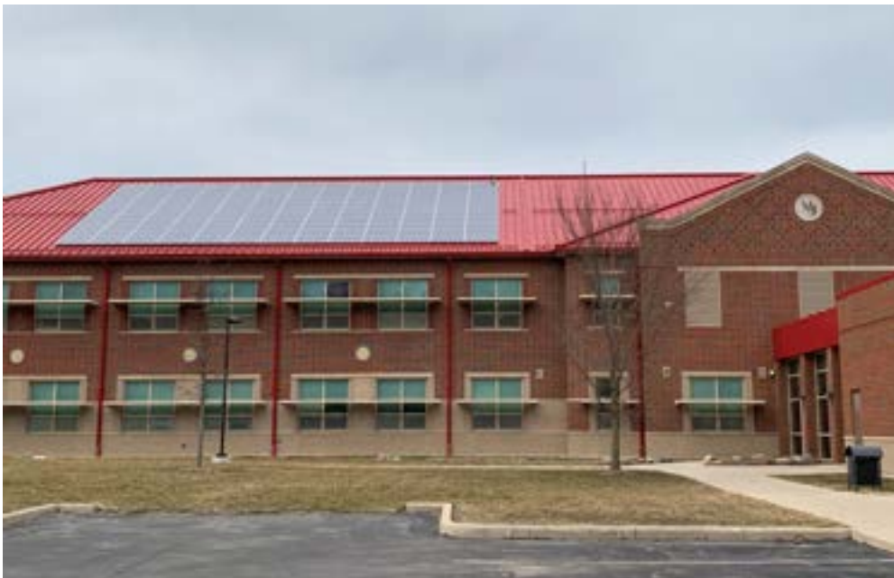
Solar panels on roof of building
