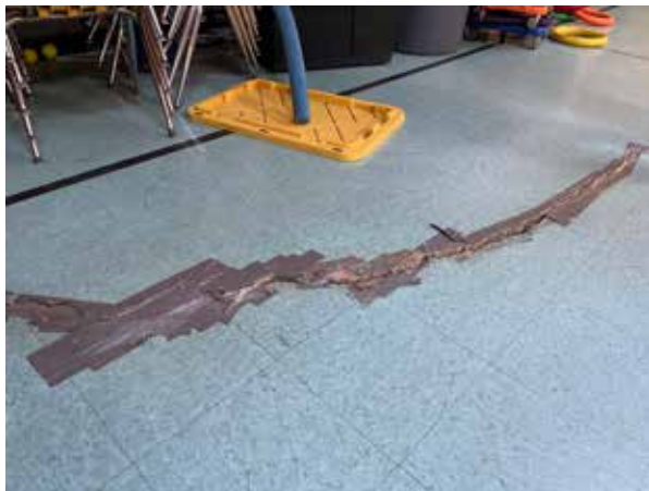
Multipurpose foundation cracks
