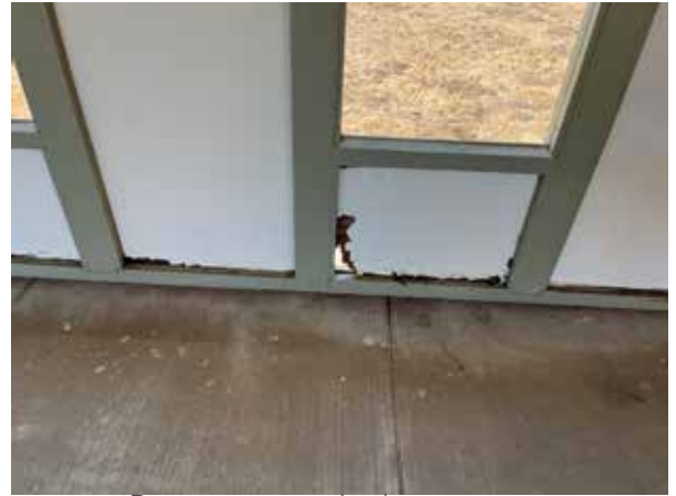
Dry rot on exterior breezeway
