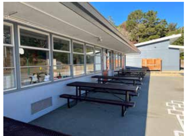
Replace original window systems
