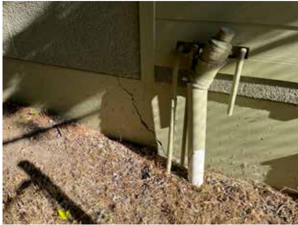
Multipurpose foundation cracks
