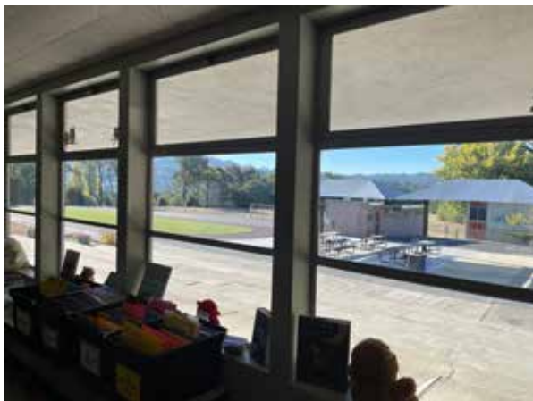
Replace original window systems
