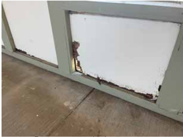
Dry rot on exterior breezeway
