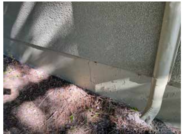
Multipurpose foundation cracks
