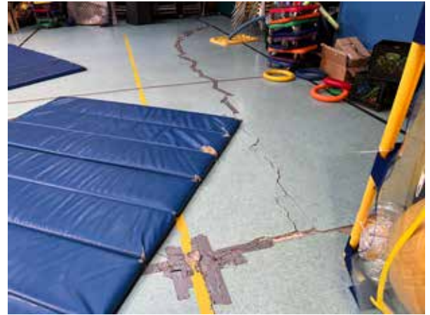
Multipurpose foundation cracks
