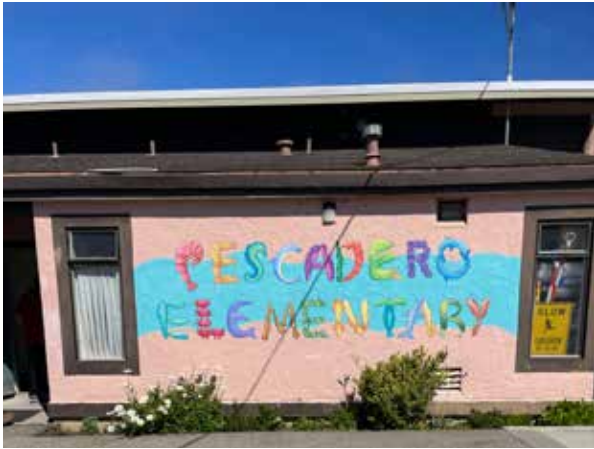
Replace original window systems
