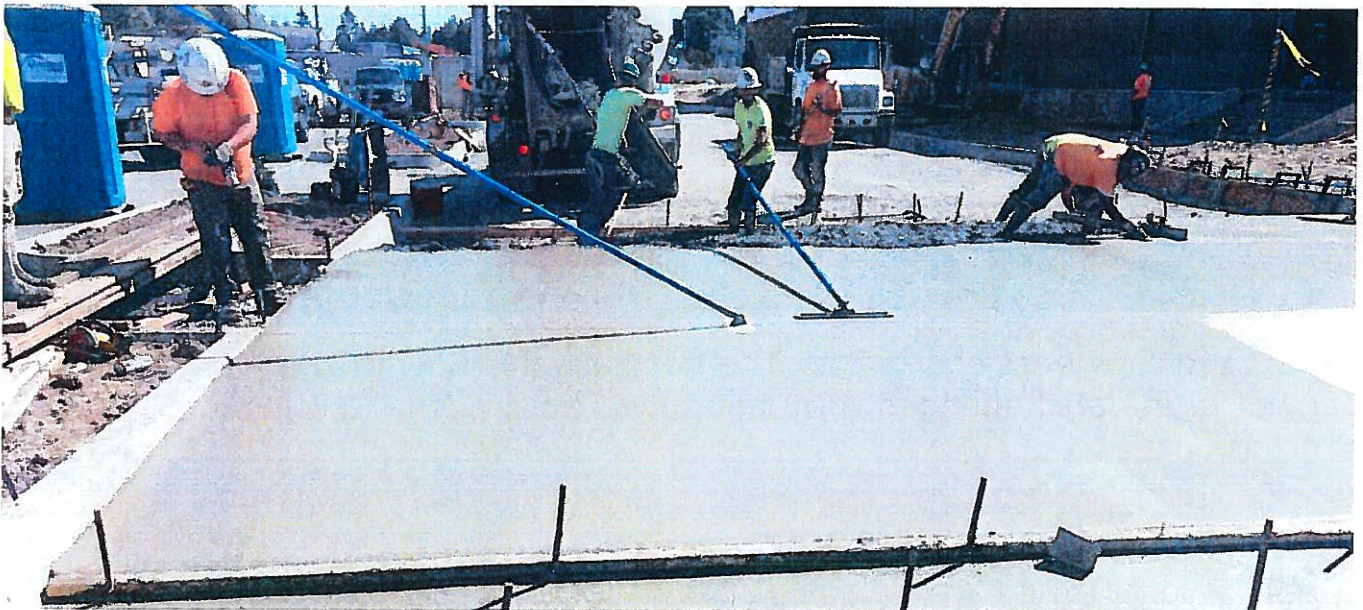
SRIS / VRMS – North (main entry) drive – wide speed bump for controlled speed and ADA accessibility. Paving this drive by 6/27.
