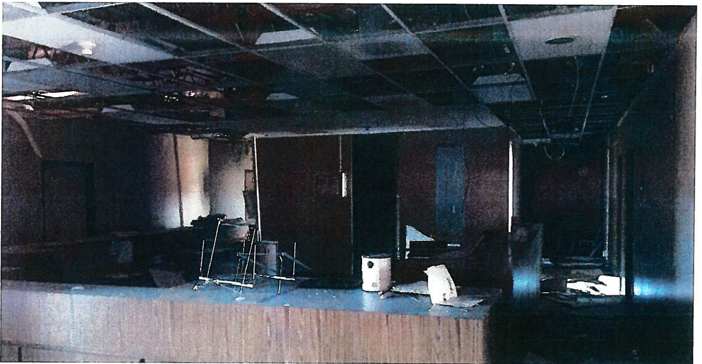
HIGH SCHOOL – Old Office abated and systems cut. Demolition in progress – that coffee cup didn't make it.
