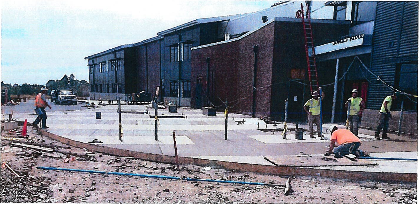
SRIS / VRMS – South entry concrete now placed with plenty of time to cure before movers arrive 7/2.
