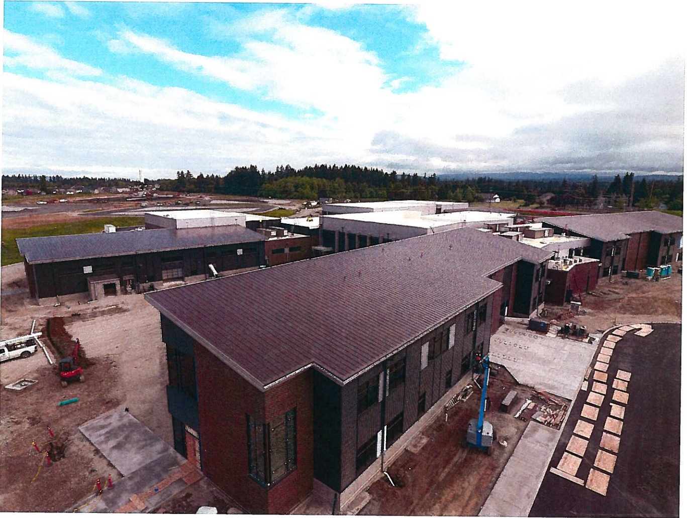
MIDDLE SCHOOL - The most recent aerial photo is from May 14th. Sidewalks going in and planters being prepped.
