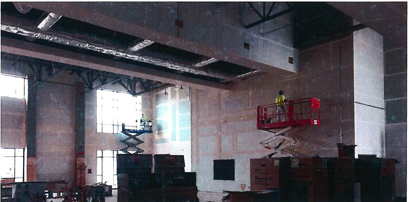
Commons wallboard being taped. Scheduled to start painting first week of May.
