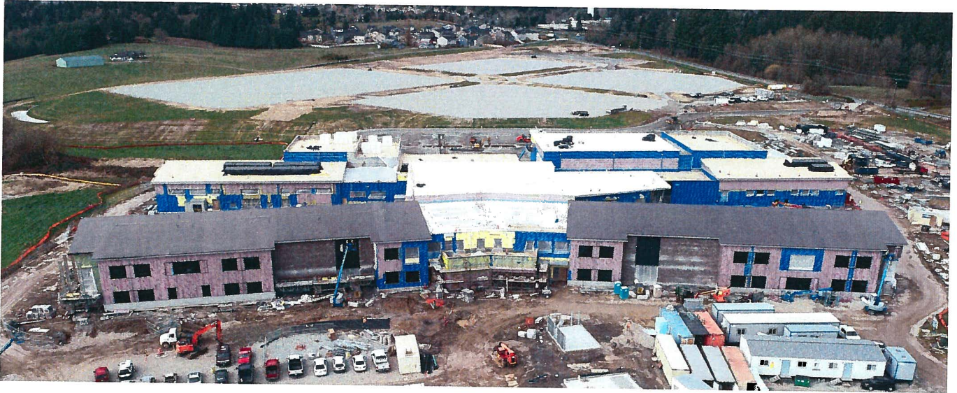
Aerial from South – Permanent roofs on classroom wings, commons, and main gym. RORC field prep in the background.
