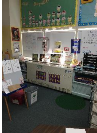
Original Unit Ventilator
