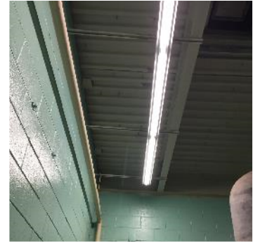
Typical Industrial Fluorescent Fixture
