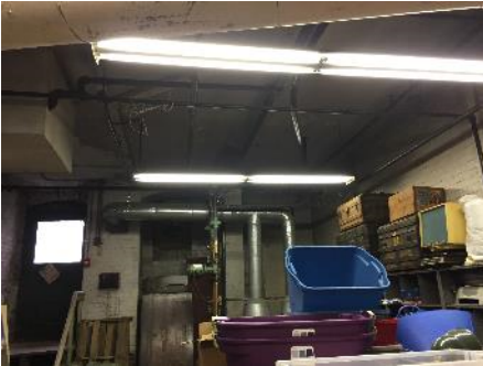
Pendant Industrial Fluorescent Fixtures
