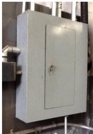
Newer Electrical Panel
