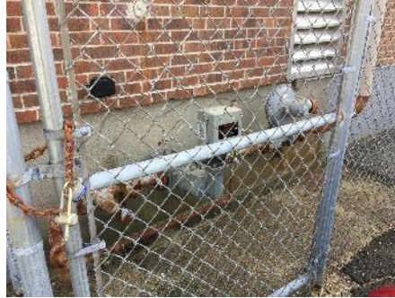
Natural Gas Service Equipment
