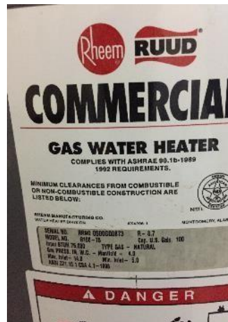
Natural Gas Fired Water Heater
