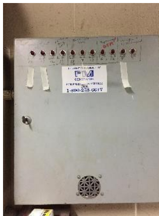
Emergency Lighting Relays
