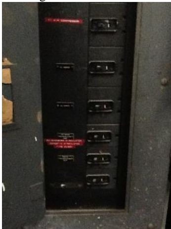
Original Electrical Panel
