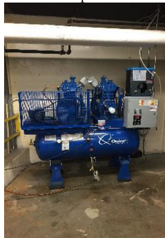
Temperature Control System Compressor
