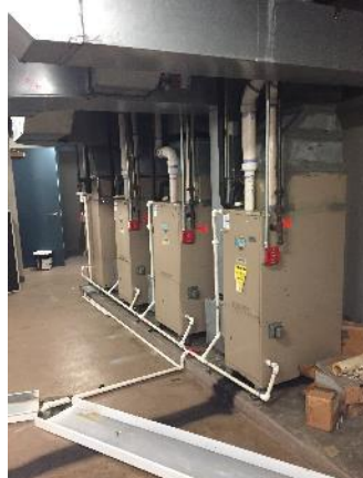
Typical Air Handling Units
