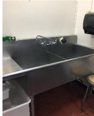
2-Bay Sink in Kitchen
