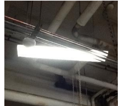
Pendant Industrial Fluorescent Fixture
