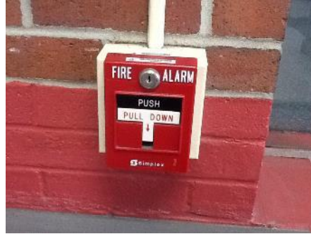
Typical Fire Alarm Manual Pullstation
