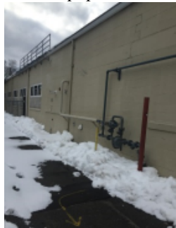
Natural Gas Service Equipment
