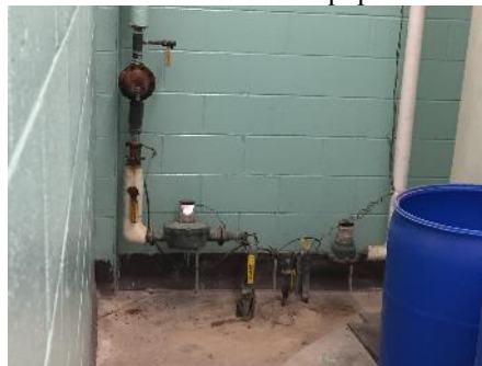
Water Services and Equipment
