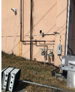
Gas Service Equipment
