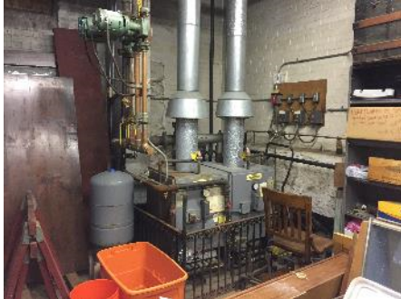
Existing Hot Water Boilers
