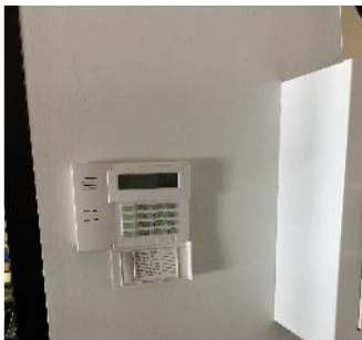
Fire Alarm/Security System Control Panel
