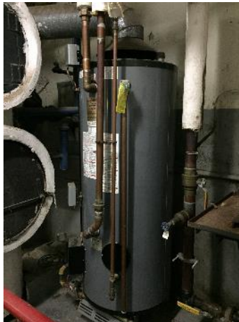
Domestic Water Heater
