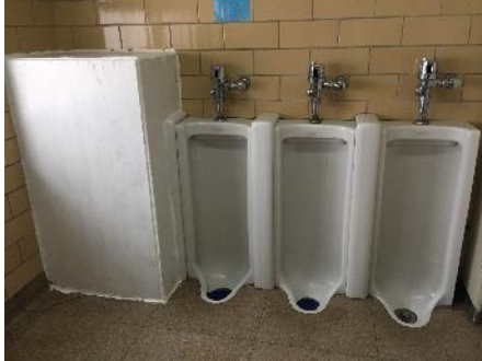
Floor Mounted Urinals
