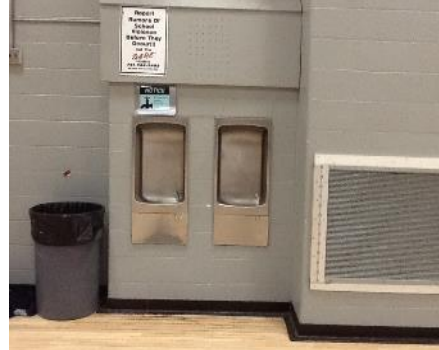
Recessed Drinking Fountains in Gym
