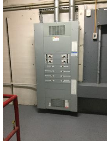
Main Distribution Panelboard
