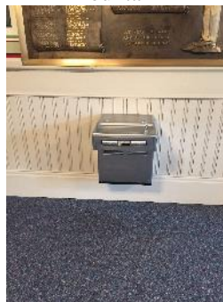
Typical Drinking Fountain
