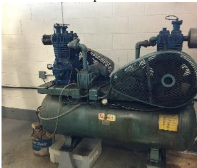
Temperature Control System Air Compressor
