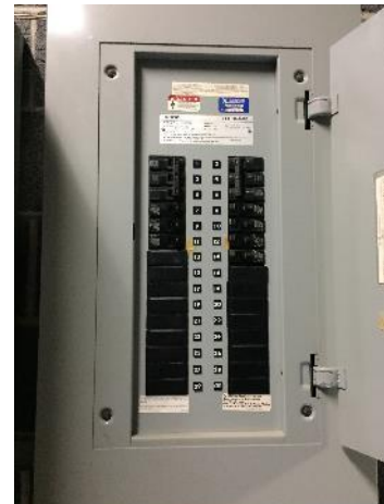
New Electrical Panel
