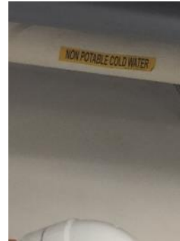
Non potable Cold Water
