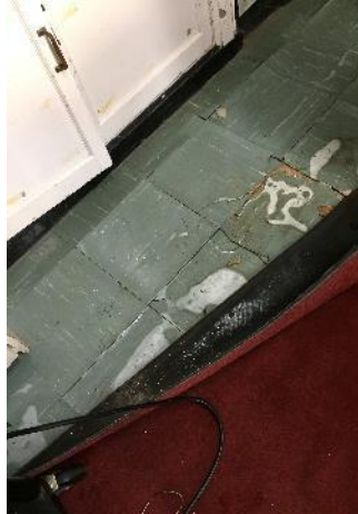
Floor Tiles Lifting Due to Steam Leak under Floor
