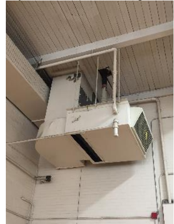
Gymnasium Air Handling Unit
