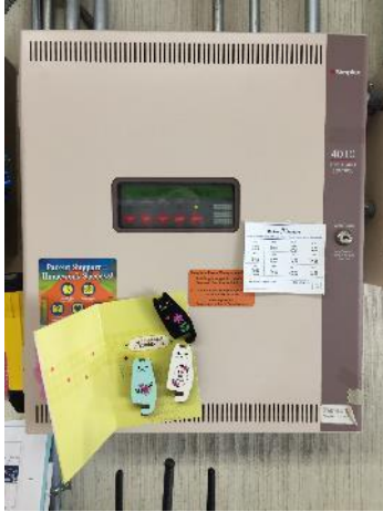
Fire Alarm Control Panel
