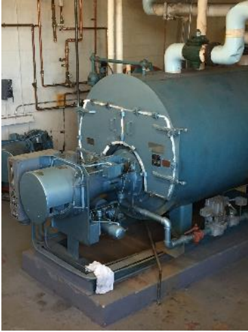
Fire Tube Boiler
