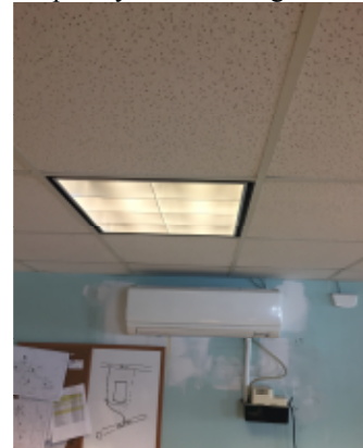
Split System Cooling Unit
