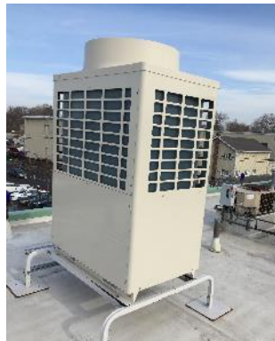
VRF System Condensing Unit on Roof
