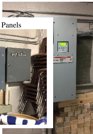
Automatic Transfer Switch
