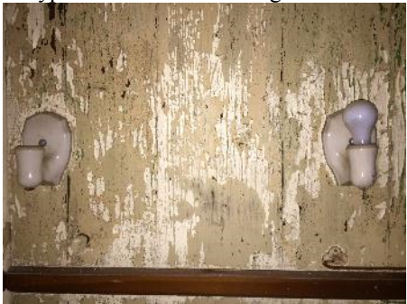
Typical Wall Mounted Light Fixtures
