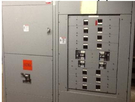
Main Electrical Service Equipment
