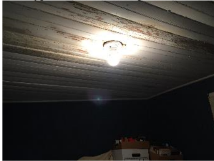
Typical Bare Bulb Light Fixture
