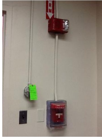
Typical Fire Alarm Manual Pullstation and Horn/Strobe
