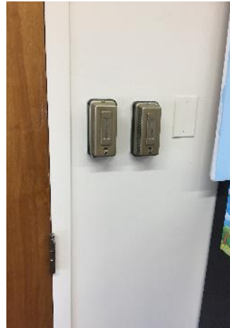
Typical Pneumatic Thermostats
