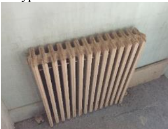
Typical Cast Iron Radiator
