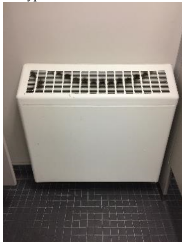
Typical Hot Water Radiator
