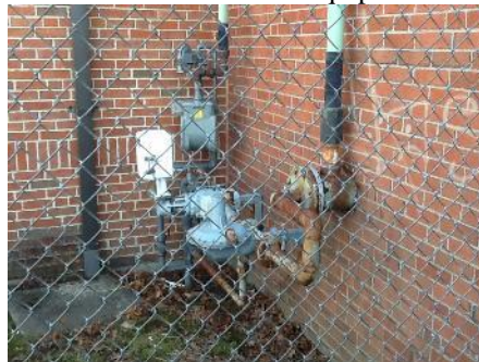
Natural Gas Service Equipment
