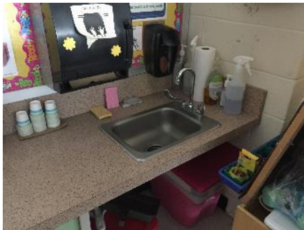
Classroom Sink w/o Bubbler
