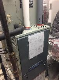
Gas Fire Furnace
