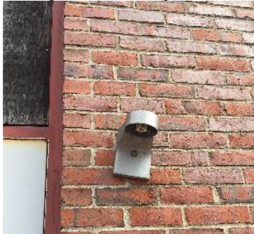
Damaged Exterior Light Fixture
