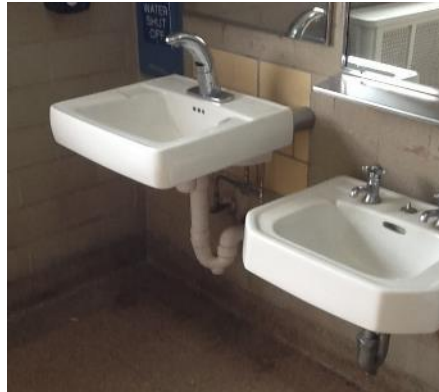
Wall Mounted Lavatories
