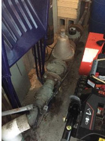
Domestic Water Service Equipment
