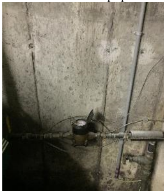
Water Service Equipment
