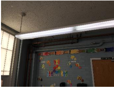
Typical Classroom Pendant Fluorescent Fixture
