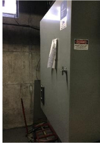
Automatic Transfer Switch
