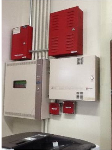
Fire Alarm Control Panel and Wireless Master Box
