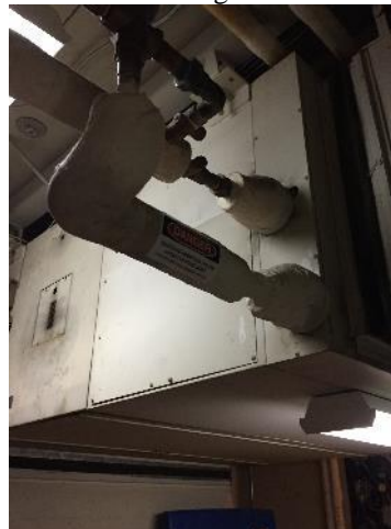
Gymnasium Indoor Air Handling Unit
