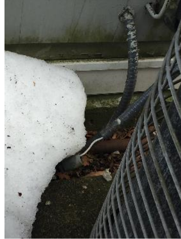
Damaged Electrical Wiring
