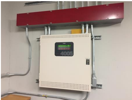
Fire Alarm Control Panel
