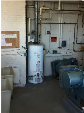
Domestic Water Heater
