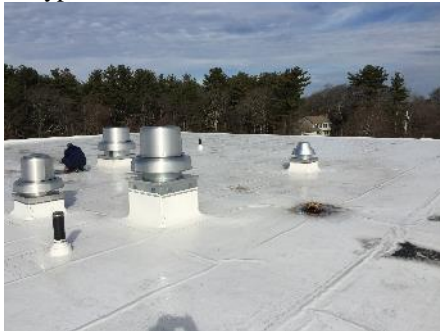
Typical Roof Mounted Exhaust Fans
