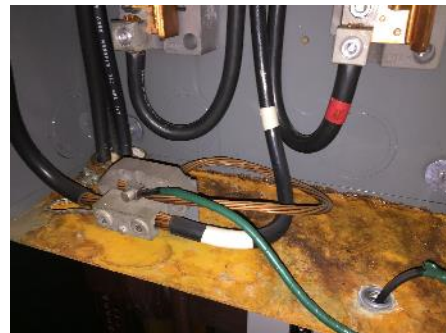
Evidence of Water in Main Service Disconnect Switch
