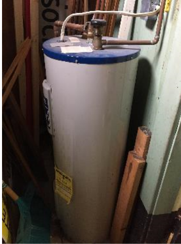
Existing Domestic Water Heater
