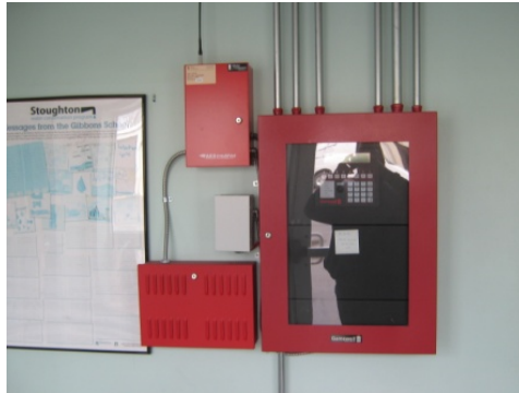
Fire Alarm Control Panel
