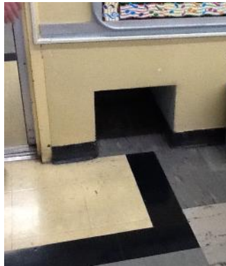
Typical Exhaust Shaft in Classrooms
