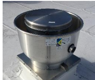
Roof Mounted Kitchen Exhaust Fan
