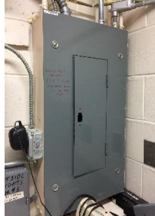
Typical Electrical Panel
