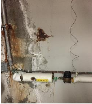
Domestic Water Service and Damaged Insulation
