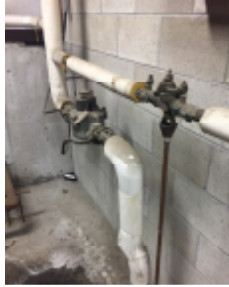
Domestic Water Service Equipment
