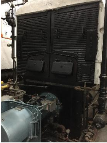
Cast Iron Boiler (1 of 2)
