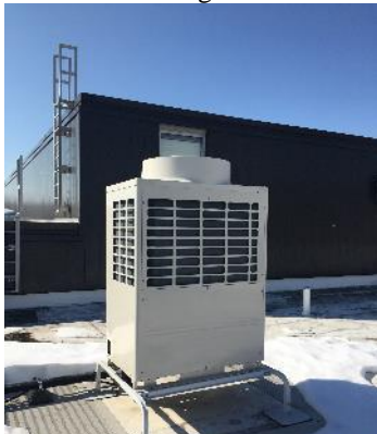
VRF Condensing Unit on Roof
