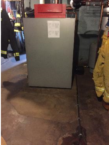
New Hot Water Boiler
