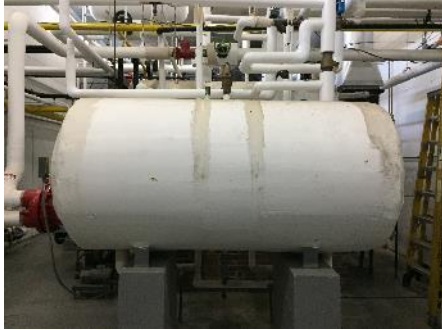
Domestic Hot Water Storage Tank
