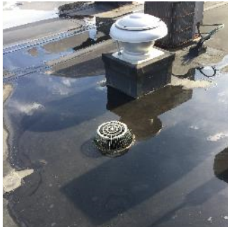
Roof Drain with Ponding Water
