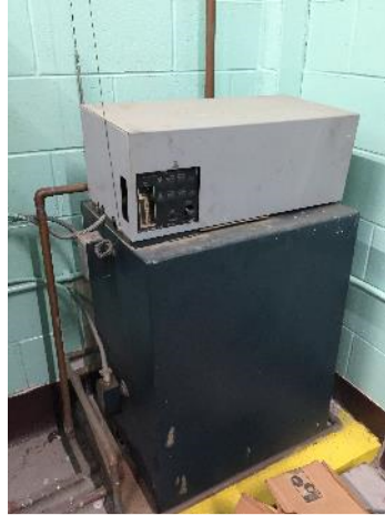
Generator Day Tank
