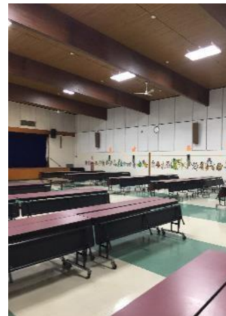
LED Fixtures in Cafeteria
