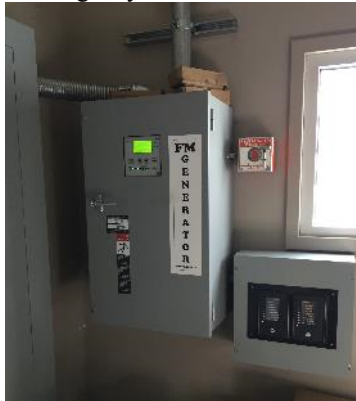
Automatic Transfer Switch, Annunciator, Emergency Shut-Down Switch
