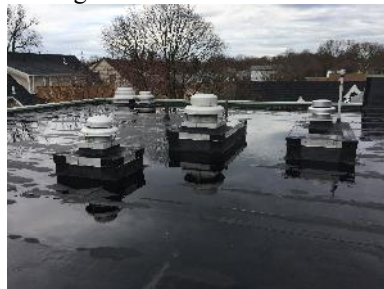
Existing Roof Mounted Exhaust Fans
