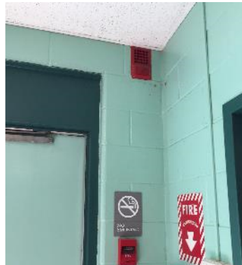
Non-ADA Fire Alarm Pullstation and Horn Strobe
