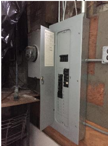
Electrical Service Equipment
