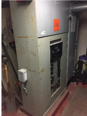
Main Switch and Distribution
