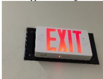
Typical Exit Sign
