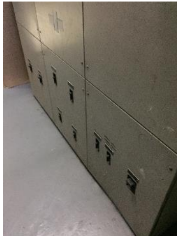
Main Electrical Switchboard
