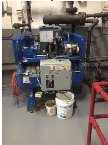
Temperature Control System Compressor
