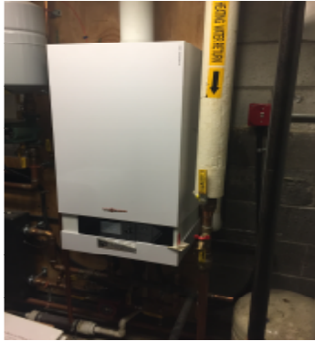
Hot Water Boiler
