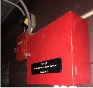
Existing Fire Alarm Control Panel
