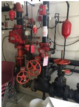
Fire Protection Service Equipment
