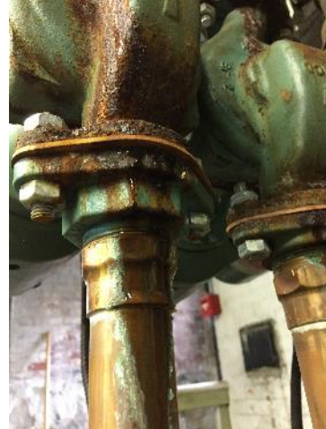
Existing Flanges that are Leaking
