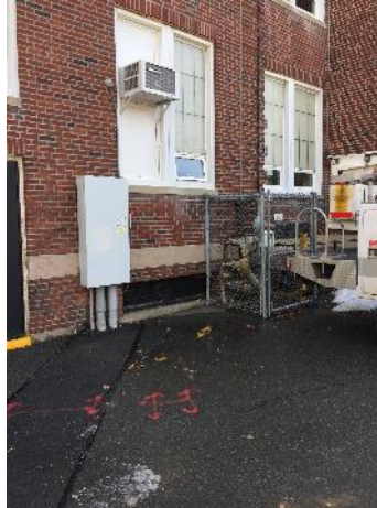
Electric Service Main Disconnect Switch
