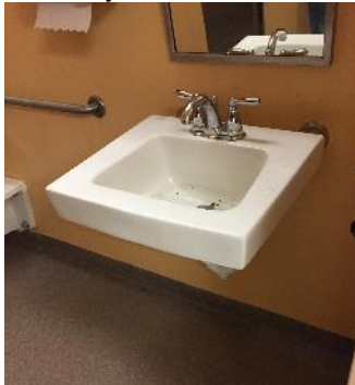
Lavatory with Lever Faucets
