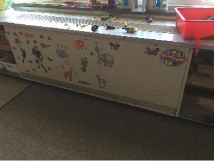
Typical Classroom Unit Ventilator
