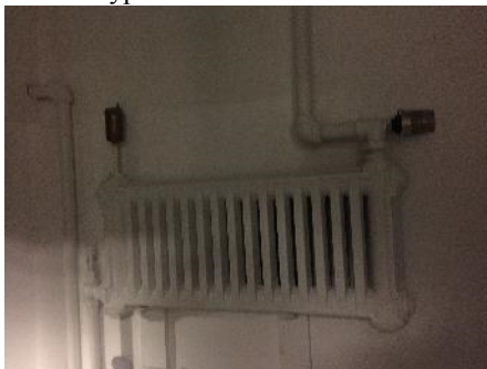
Typical Cast Iron Radiator
