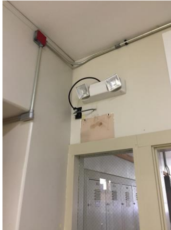
Typical Emergency Lighting Fixture
