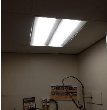
Recessed Fluorescent Fixture
