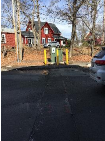
Utility Co. Transformer with Revenue Meter
