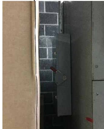
Disconnect Switch with not the required clearance
