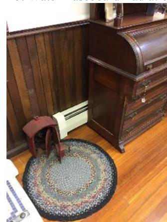
Hot Water Baseboard Radiation
