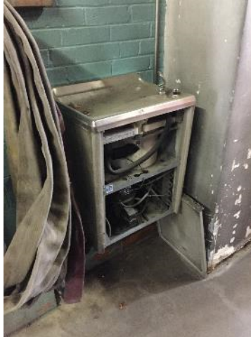
Drinking Fountain in Apparatus Bay
