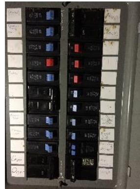
Electric Service Panelboard
