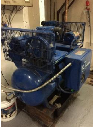
Temperature Control System Compressor
