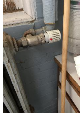
Typical Manual Valve on Radiator
