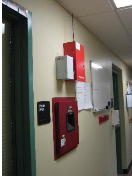
Fire Alarm Control Panel and Dialer
