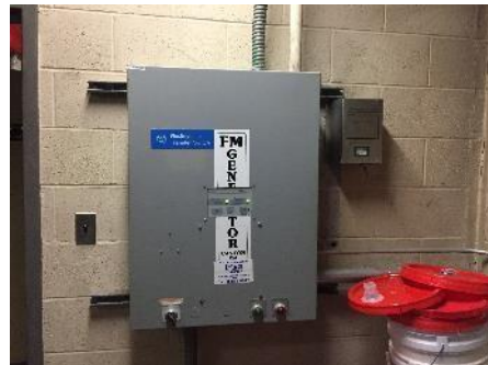
Automatic Transfer Switch
