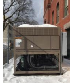
Air Cooled Chiller
