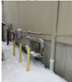
Natural Gas Service Equipment
