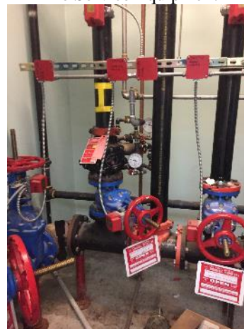
Fire Service Equipment
