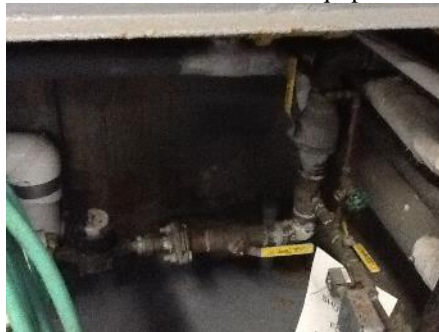
Domestic Water Service Equipment
