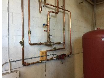
Tempering Valve and Piping
