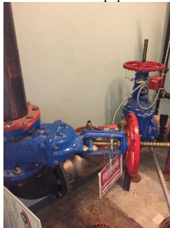
Fire Service Equipment
