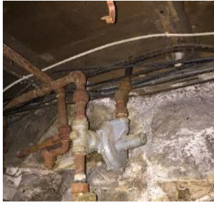
Remains of Gas Service
