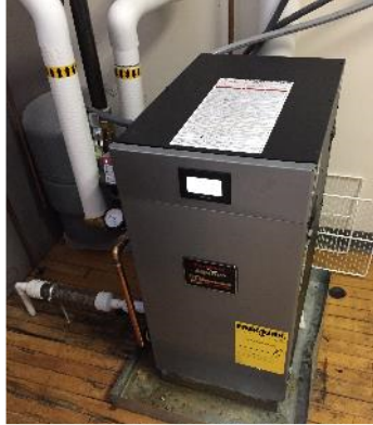
Hot Water Boiler
