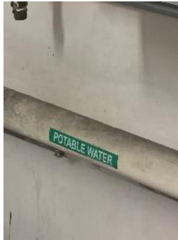
Potable Cold Water
