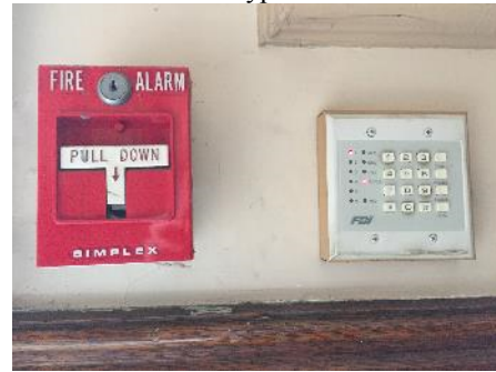
Typical Manual Pullstation and Security Keypad
