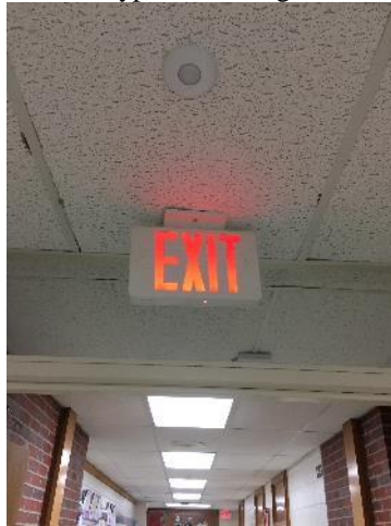
Typical Exit Sign
