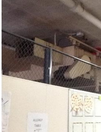
Cafeteria Air Handling Equipment
