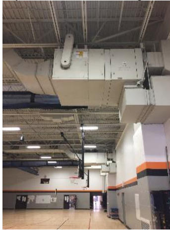
Gymnasium Air Handling Unit
