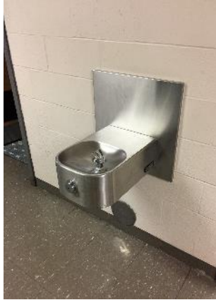
Single Level Drinking Fountain
