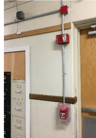
Typical Fire Alarm Manual Pullstation and Horn Strobe
