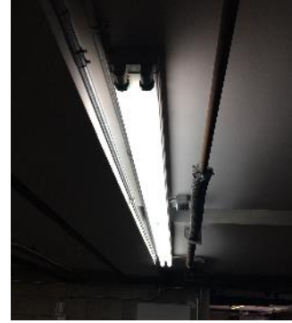
Typical Industrial Fluorescent Fixture
