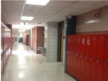
Wall Mounted Drinking Fountain in Corridor
