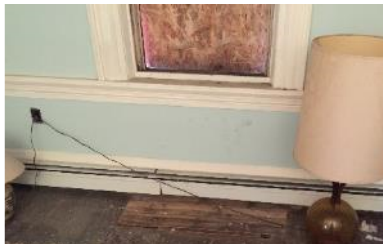
Hot Water Baseboard Radiation
