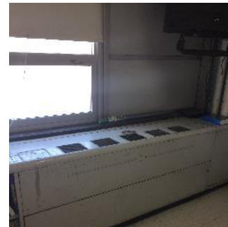
Typical Classroom Unit Ventilator
