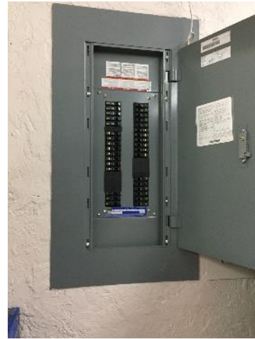
New Electrical Panels
