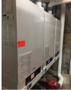
Hot Water Boiler
