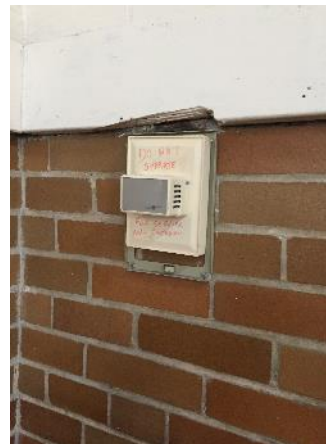
Wall Mounted Temperature Sensor
