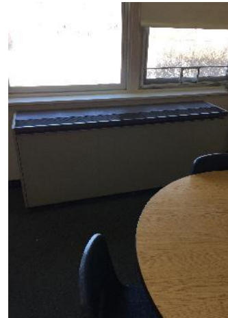
Newer Unit Ventilator
