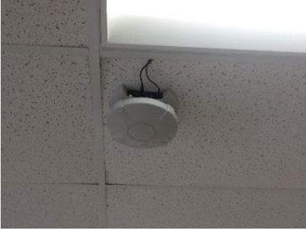
Typical Wireless Access Point
