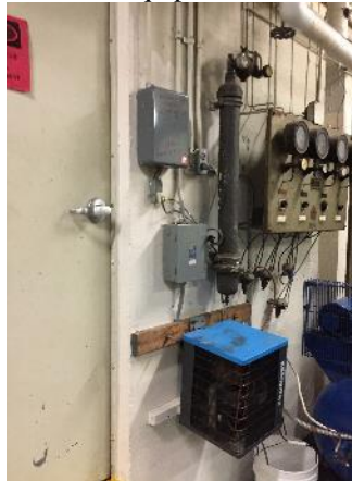
Temperature Control System Air Dryer and other Equipment
