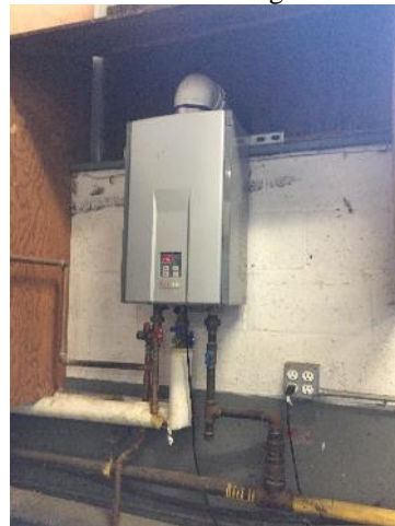
Water Heater Serving Kitchen
