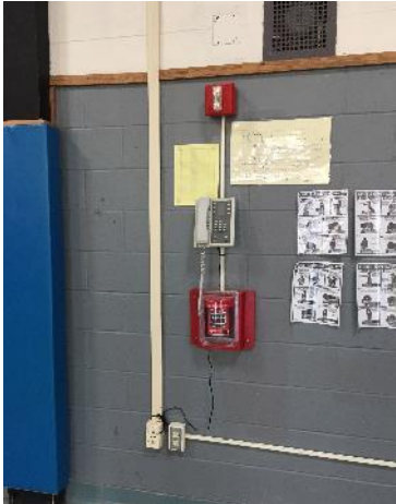
Fire Alarm Pullstation, Horn Strobe
