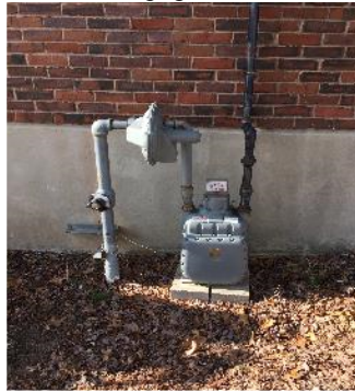
Natural Gas Service Equipment
