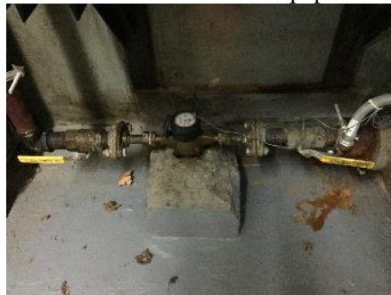
Domestic Water Service Equipment
