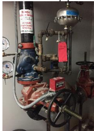
Fire Service Equipment
