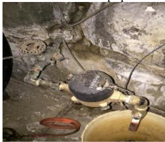
Water Service Equipment
