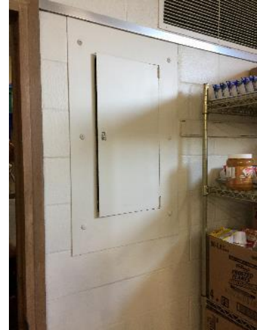
Typical Electrical Panel Cover
