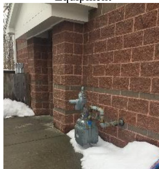
Natural Gas Service Equipment
