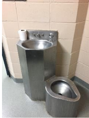
Typical Cell Area Fixture
