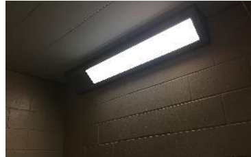
Wall Mounted Fluorescent Fixture in Cells
