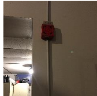
Existing Fire Alarm Horn/Strobe
