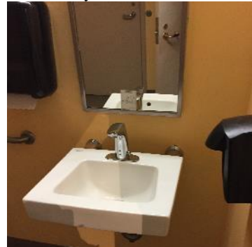
Lavatory with Sensor Faucet
