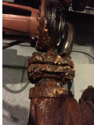
Leaking Flange at Pump
