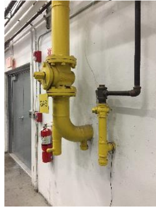
Natural Gas Piping as it enters the Building
