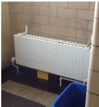
Cast Iron Radiator
