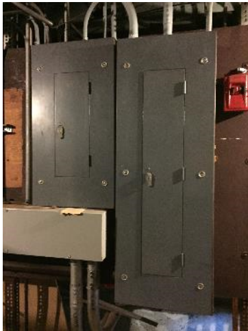
Older Electrical Panels
