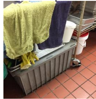
Above Grade Grease Interceptor
