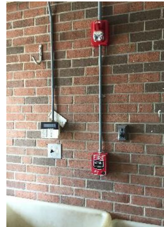
Typical Fire Alarm Pullstation and Horn/Strobe
