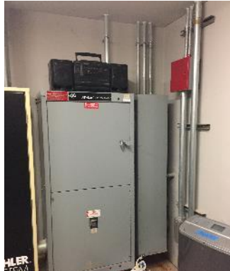
Electric Service Main Disconnect Switch
