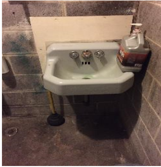
Lavatory in Garage
