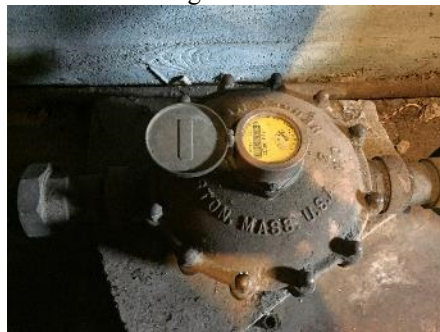
Existing Water Meter
