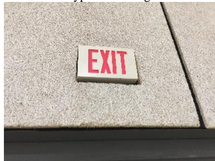
Typical Exit Sign
