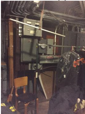
Electrical Service Equipment
