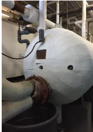
Domestic Hot Water Storage Tank
