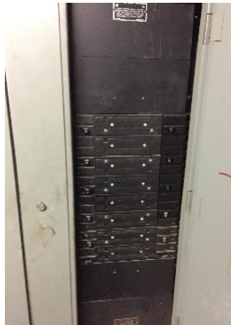
Typical Original Electrical Panel
