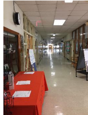
Recessed Fluorescent Fixture
