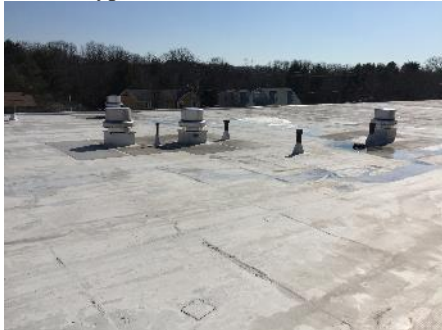
Typical Roof Exhaust Fans
