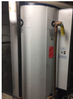
Domestic Water Heater
