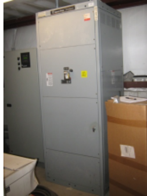
Main service switch
