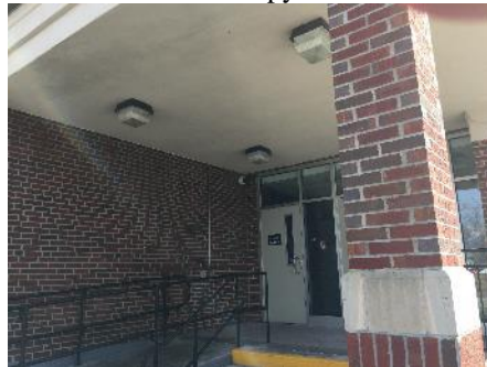
Surface Mounted Fixtures at Entrance Canopy
