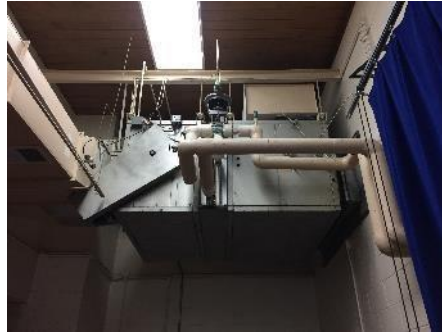
Indoor Air Handling Unit
