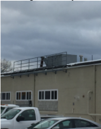
Packaged Roof Top Unit
