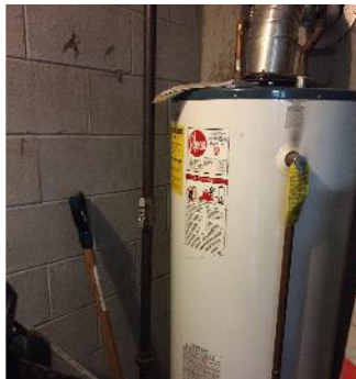
Domestic Water Heater
