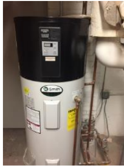
Domestic Hot Water Heater
