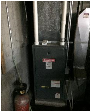
Hot Air Furnace
