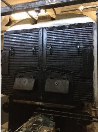
Cast Iron Boiler
