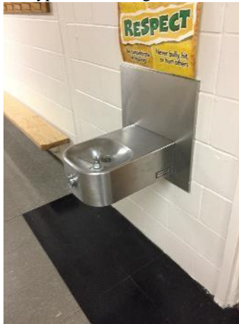
Typical Drinking Fountain
