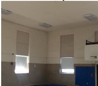
LED Fixtures in Gymnasium
