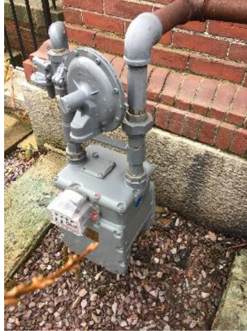
Natural Gas Service Equipment
