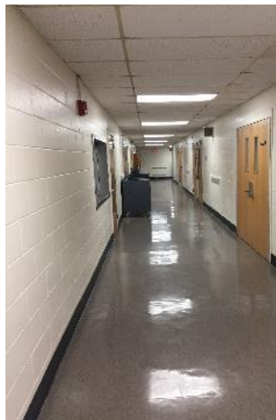
Typical Recessed Fluorescent Fixtures
