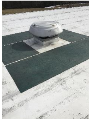
Typical Roof Exhaust Fan
