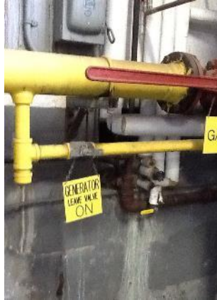
Natural Gas piping as it enters the Boiler Room
