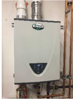
Domestic Hot Water Heater
