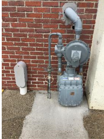
Natural Gas Service Equipment
