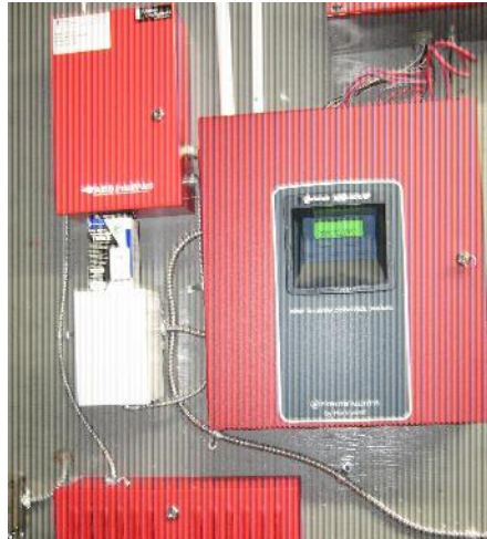
Fire Alarm Control Panel and Dialer
