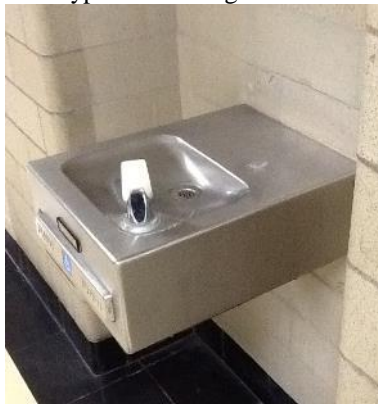
Typical Drinking Fountain
