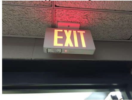
Typical Exit Sign
