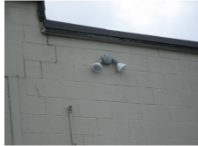
Wall mounted Flood Light Fixtures
