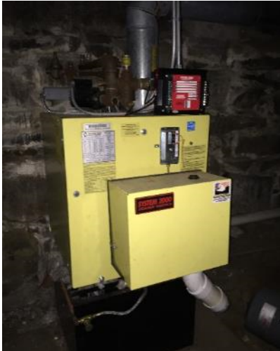
Hot Water Boiler
