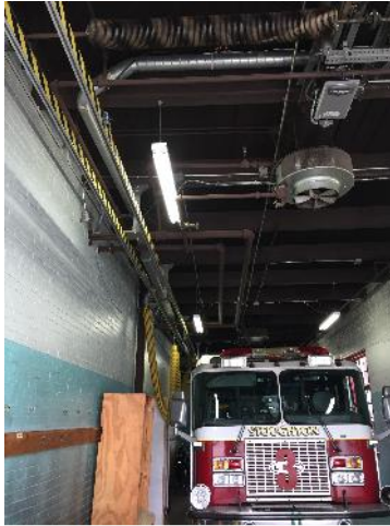
Apparatus Bay Unit Heater
