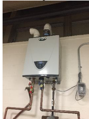
High Efficiency Water Heater Serving Kitchen
