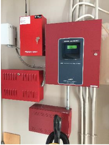
Fire Alarm Control Panel and Wireless Transmitter
