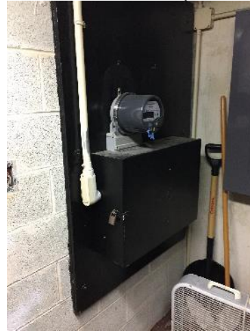
C/T Cabinet and Utility Meter
