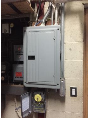
Electrical Load Center
