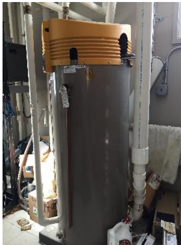
Domestic Water Heater
