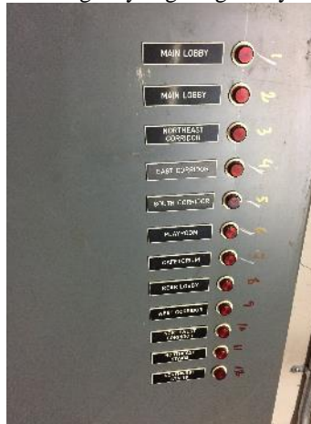
Emergency Lighting Relays
