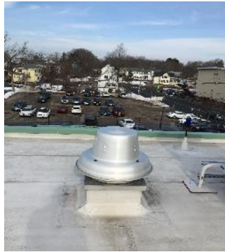
Typical Roof Mounted Exhaust Fan
