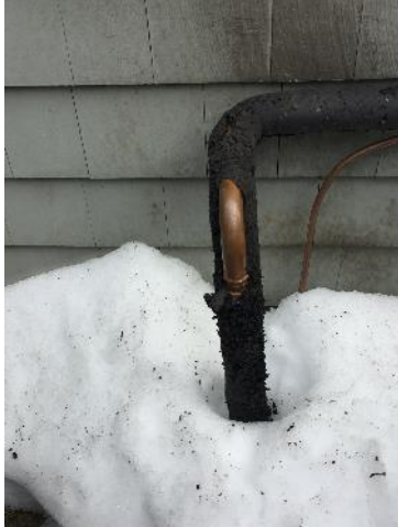
Damaged Refrigeration Piping Insulation
