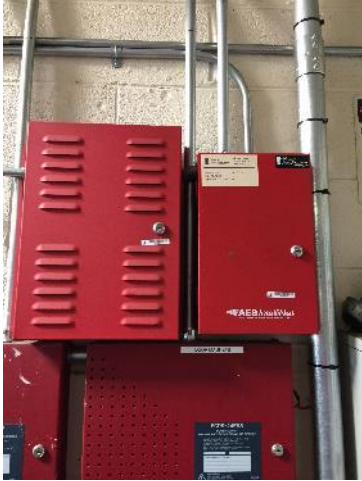
Fire Alarm Wireless Master Box
