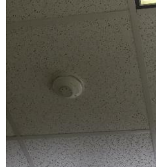
Typical Heat Detector
