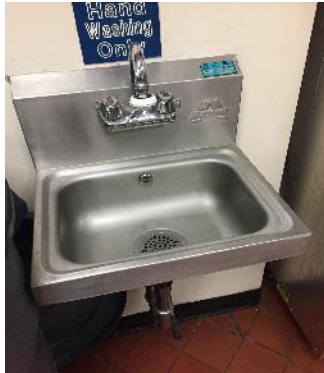
Handwash Sink in Kitchen
