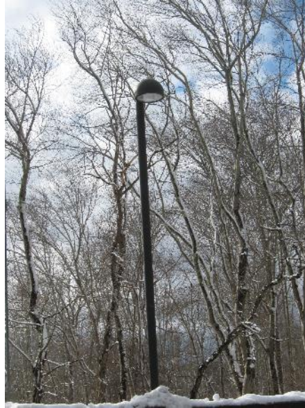
Pole Mounted Site Lighting Fixture
