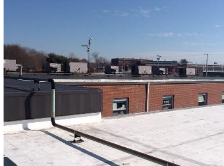
Packaged Roof-Top Units on Portable Classrooms
