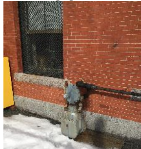
Natural Gas Service Equipment
