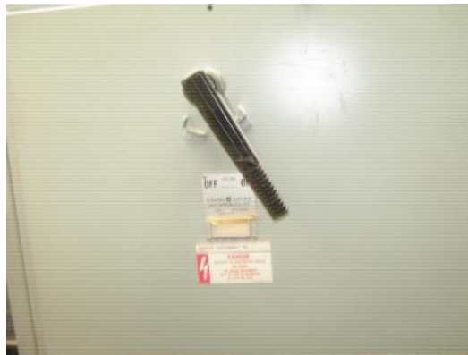
Main service switch
