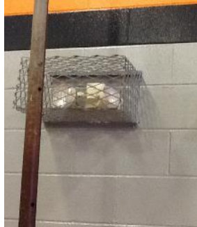
Typical Emergency Lighting Fixture
