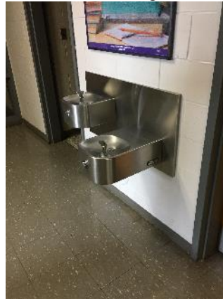
Two Level Drinking Fountain
