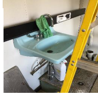
Kitchen Hand Wash Sink and Grease Interceptor Below
