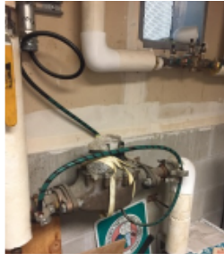
Domestic Water Service Equipment
