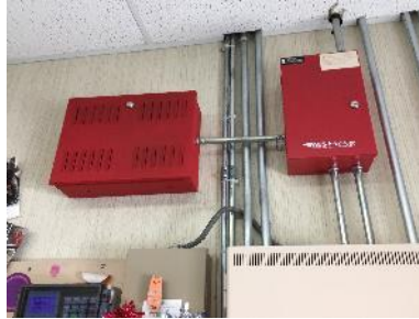
Fire Alarm Master Box
