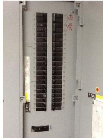
Newer Electrical Panel
