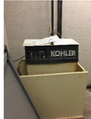
Generator Day Tank
