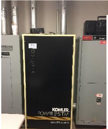
Automatic Transfer Switch
