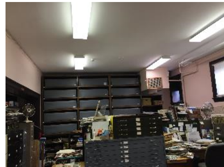
Surface Mounted Wraparound Fluorescent fixtures
