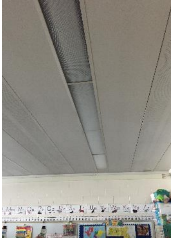
Recessed 1x4 Fixture in Classroom
