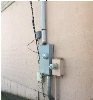
Electrical Service Entrance Equipment
