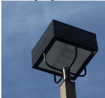
Typical Post-Top LED Site Lighting Fixture
