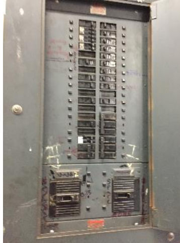
Typical Electrical Panel Interior
