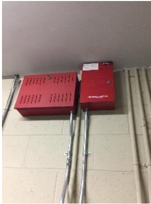
Fire Alarm Wireless Master
