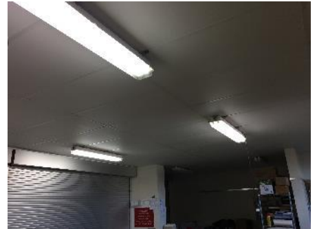
Surface Fluorescent in Kitchen
