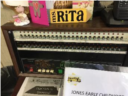
PA System Head End Equipment
