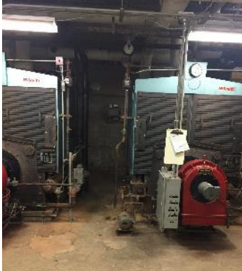
Hot Water Boilers
