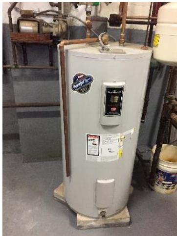
Domestic Water Heater
