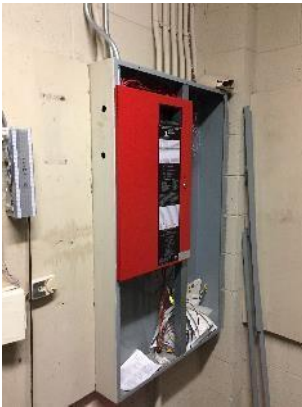
Fire Alarm Control Panel
