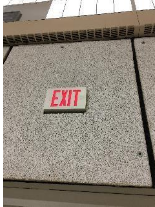
Typical Exit Sign
