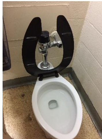
Floor Mounted Water Closet
