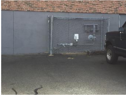
Natural Gas Service Equipment on the Exterior of the Building
