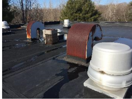
Roof Mounted Exhaust Fans, Condensing Unit, Intake Hoods
