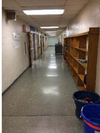
Recessed Fluorescent Fixtures in Corridors
