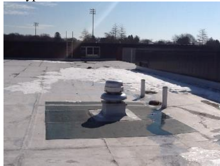
Typical Roof Mounted Exhaust Fan
