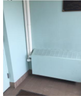
Typical Hot Water Radiator
