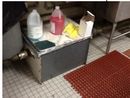
Above Grade Grease Interceptor
