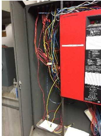
Wiring in Adjacent Pull Box
