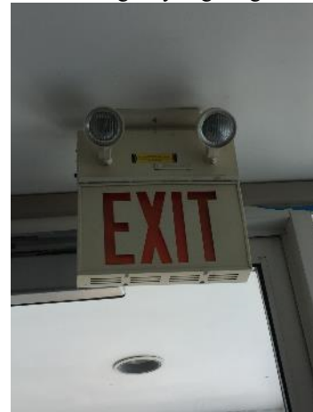
Exit Sign with Plastic Housing and Emergency Lighting
