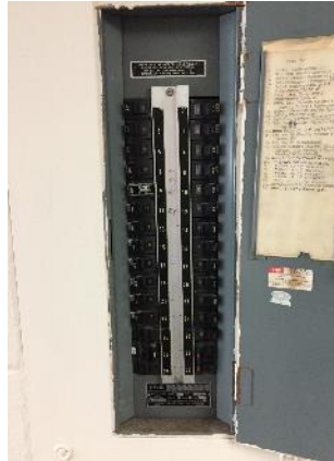
Typical Electrical Panel
