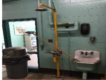
Janitor Sink and Emergency Eyewash/Shower Unit
