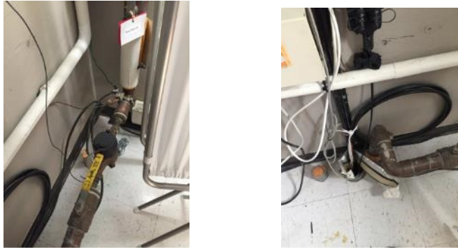
Domestic Water Service
