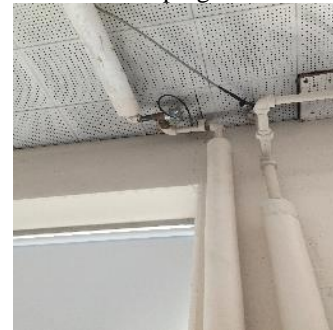
Typical Exposed Steam Piping
