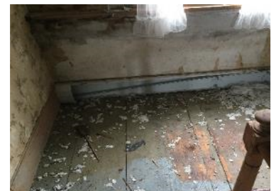
Damaged Hot Water Baseboard Radiation
