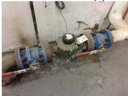
Domestic Water Service Equipment
