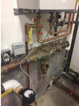
Domestic Water Service
