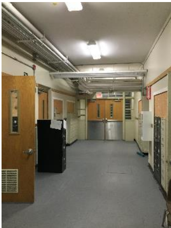
Typical Surface Mounted Fluorescent Fixture
