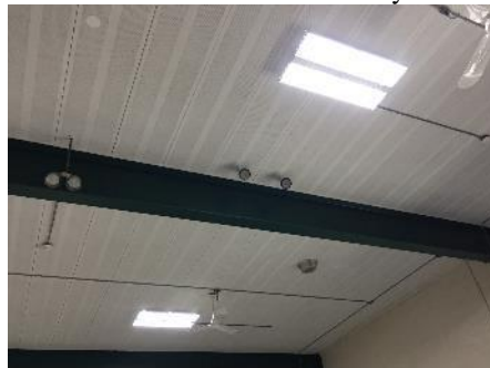
Surface LED Fixtures in Gym
