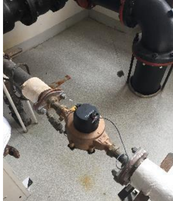
Existing Water Service Equipment
