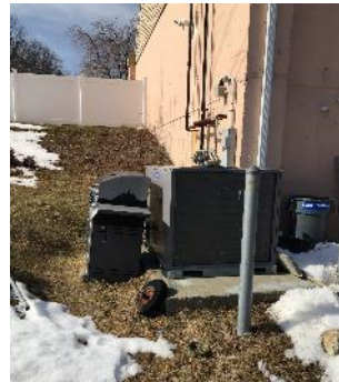
Condensing Unit Serving Hot Air Furnace
