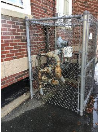
Natural Gas Service Equipment
