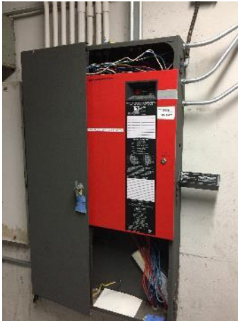
Fire Alarm Control Panel
