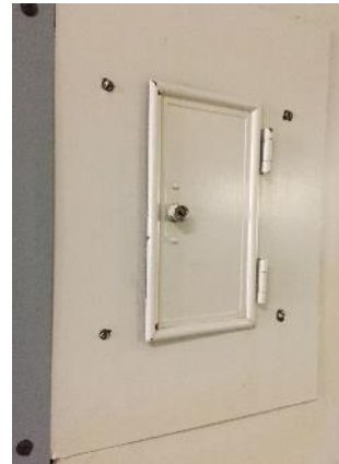
Old Electrical Panel
