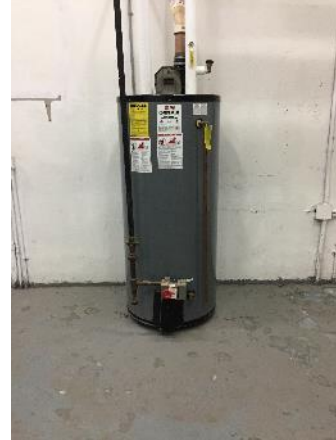
Natural Gas Fired Water Heater
