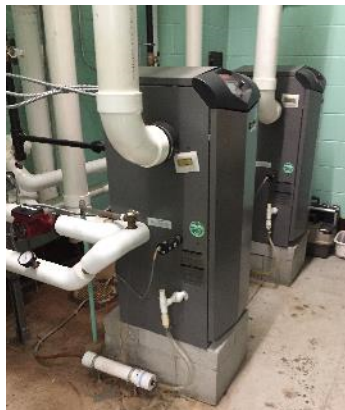
New Boiler Plant
