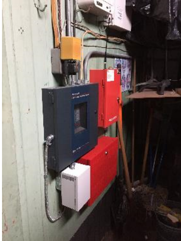
Fire Alarm Control Panel and Wireless Transmitter
