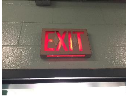
Typical Exit Sign
