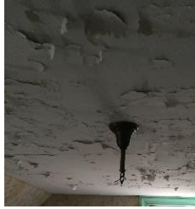
Damaged Decorative Pendant Light Fixture
