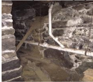
Sanitary Service Piping
