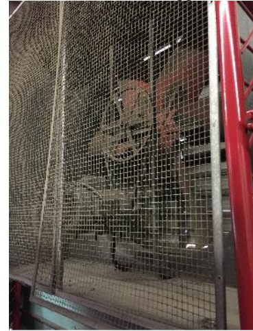
Exhaust Fan in Rear of Apparatus Bay
