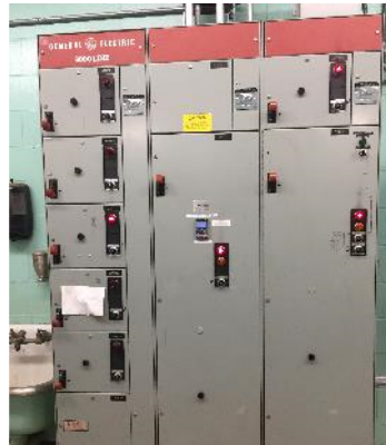
Motor Control Center
