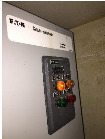
Manual Transfer Switch
