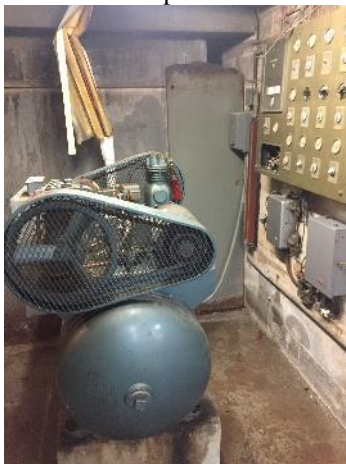
Temperature Control System Compressor
