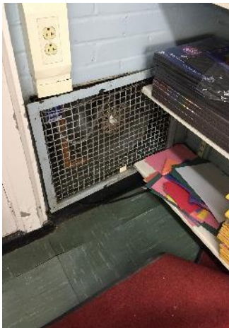
Classroom Exhaust Fan
