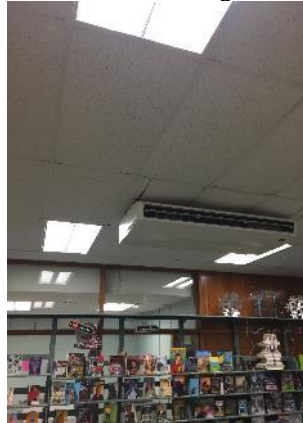
VRF Air Handling Unit
