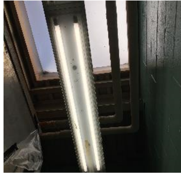
Typical 2-Lamp Industrial Fluorescent Fixture
