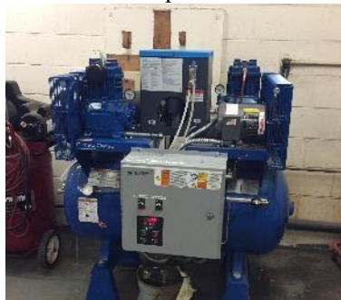
Temperature Control System Compressor
