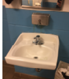
Lavatory with Metered Faucet
