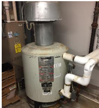
Domestic Water Heater
