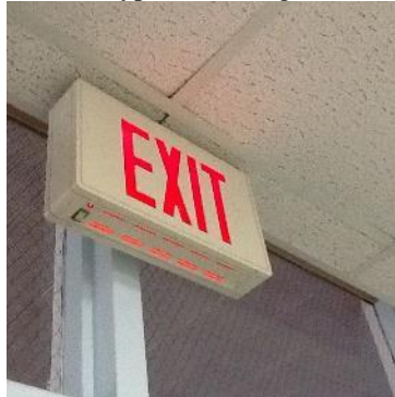
Typical Exit Sign
