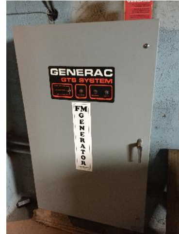
Automatic Transfer Switch
