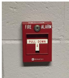
Typical Fire Alarm Pullstation
