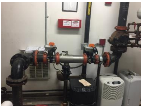
Fire Protection Service
