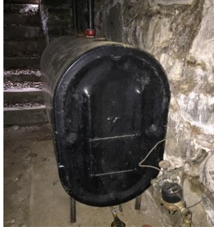
Existing Fuel Oil Tank
