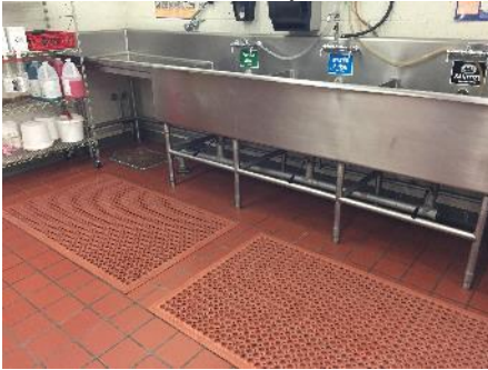
Kitchen 3-Bay Sink
