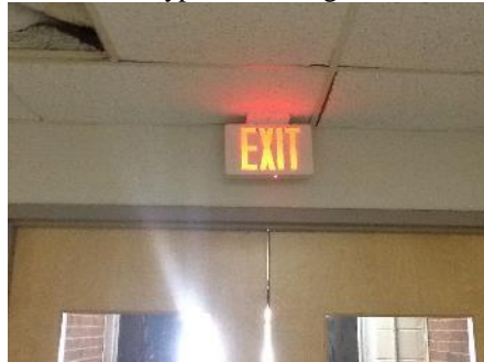
Typical Exit Sign
