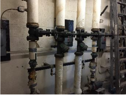
Heating Water System Valves
