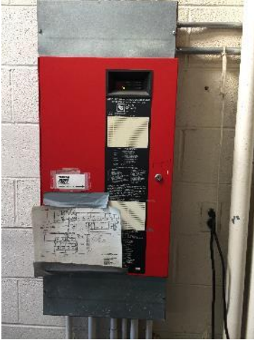
Fire Alarm Control Panel
