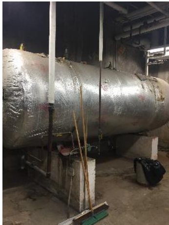
Domestic Hot Water Storage Tank
