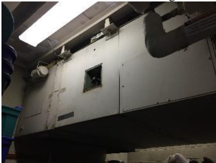
Cafeteria Indoor Air Handling Unit
