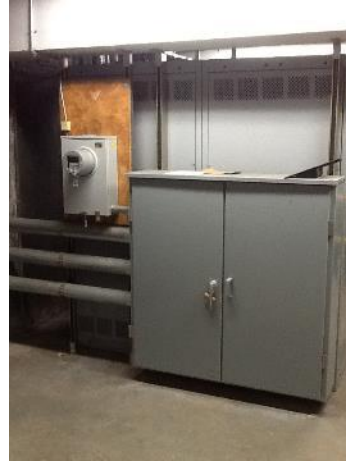
C/T Cabinet and Electric Meter
