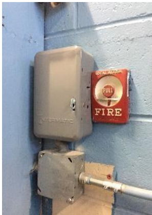
Typical Fire Alarm Pullstation
