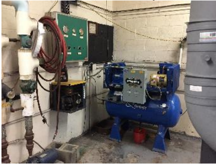
Temperature Control System Air Compressor and Dryer
