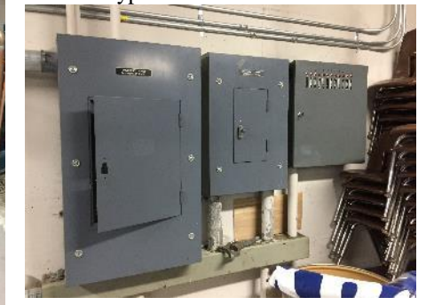
Typical Electrical Panels
