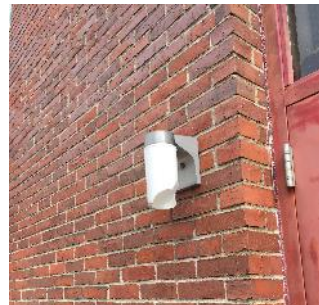
Damaged Exterior Light Fixture
