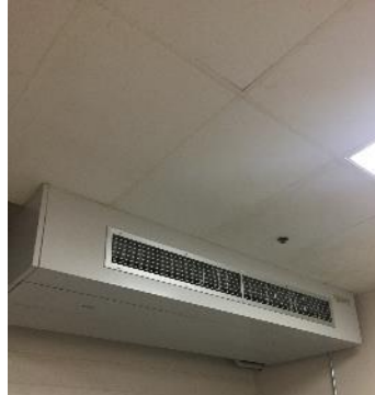
Typical Ceiling Mounted Radiation
