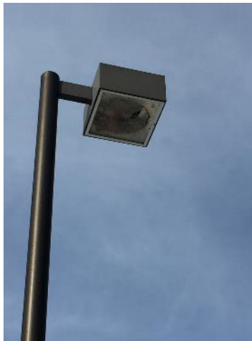
Typical Pole Mounted Site Lighting Fixture
