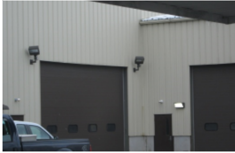
Wall Mounted HID Flood Light Fixtures
