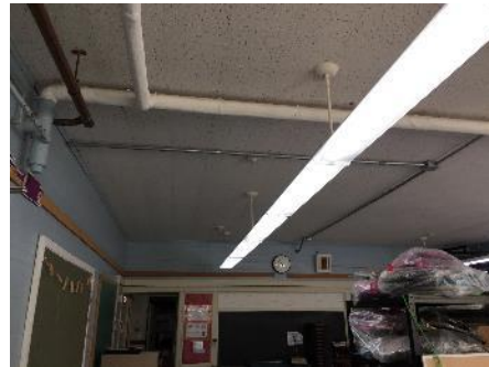
Typical Classroom Pendant Fluorescent Fixture
