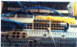
The overhaul of our infrastructure has made the technology advancements in the classroom possible.
