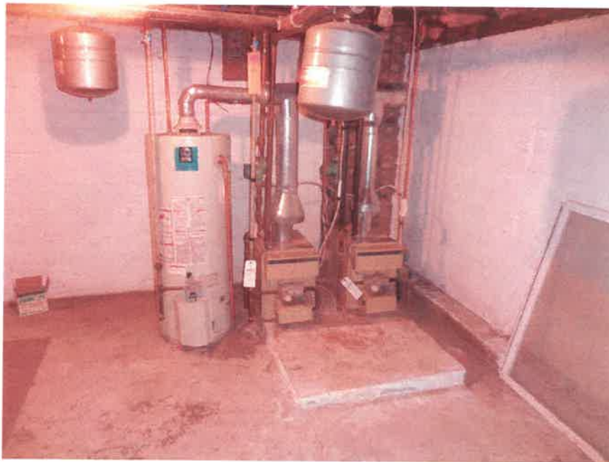
Basement – Boiler Units
