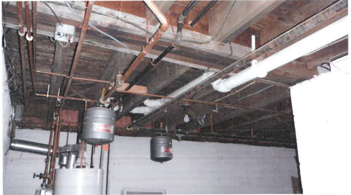
First Floor Framing at Basement Mechanical Room
