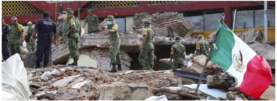
Soldiers remove debris from a partly collapsed municipal building felled
